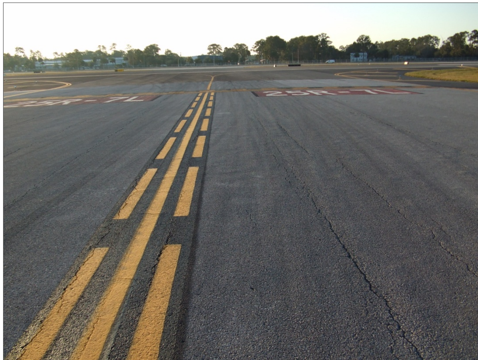
Taxiway November 3, Section 1430, Sample Unit 305 – Low to medium severity (48) Longitudinal / Transverse Cracking; and low to medium severity (52) Weathering and Raveling.
