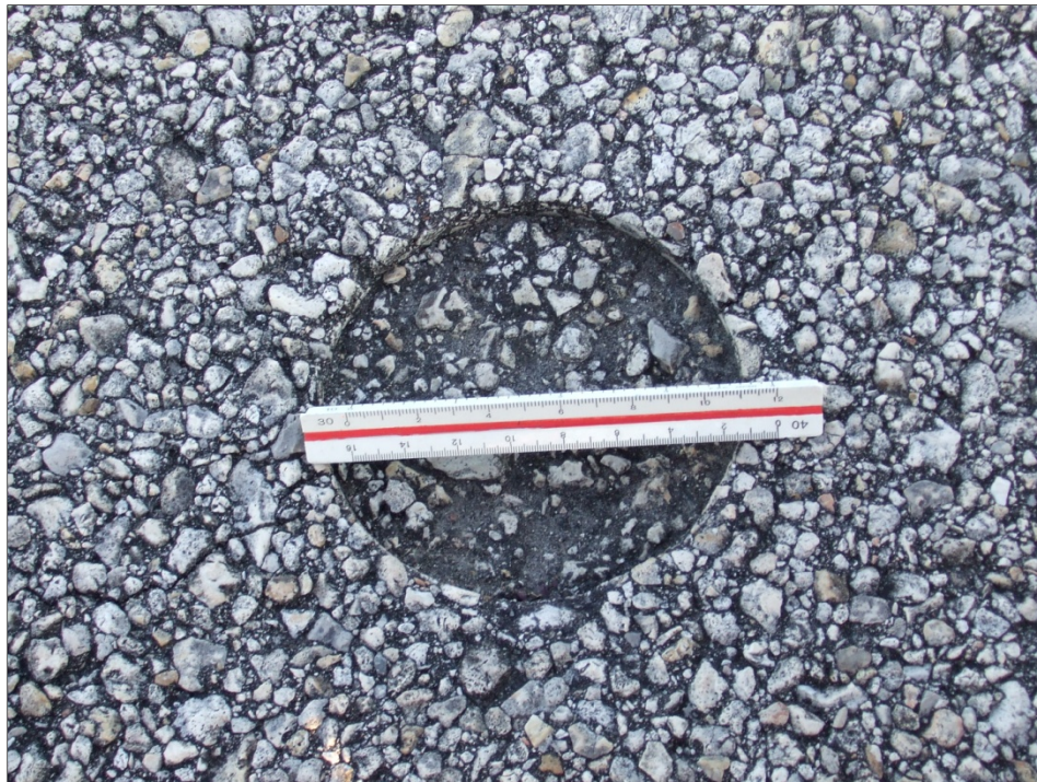
Taxiway November 4, Section 1440, Sample Unit 410 – Medium severity (50) Patching; and low severity (52) Weathering and Raveling.
