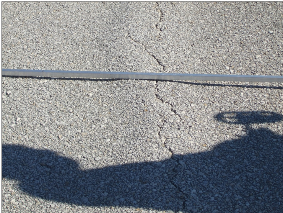
NE Apron, Section 4250, Sample Unit 307– Low severity (48) Longitudinal / Transverse Cracking; low severity (52) Weathering and Raveling; and medium severity (56) Swelling.
