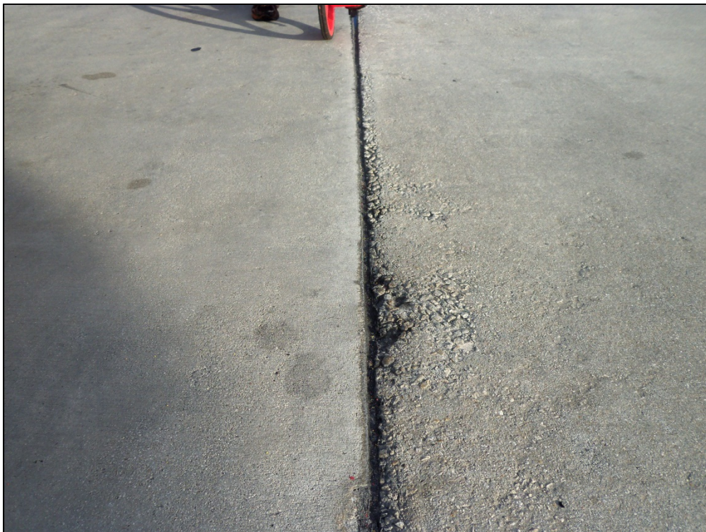
Common Aprons, Section 4082, Sample Unit 940 – Low severity (74) Joint Spalling
