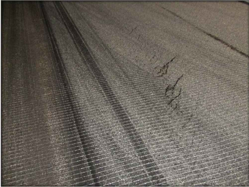
Runway 9L-27R, Section 6135, Sample Unit 326 – (55) Slippage Cracking, low severity (52) Weathering and Raveling
