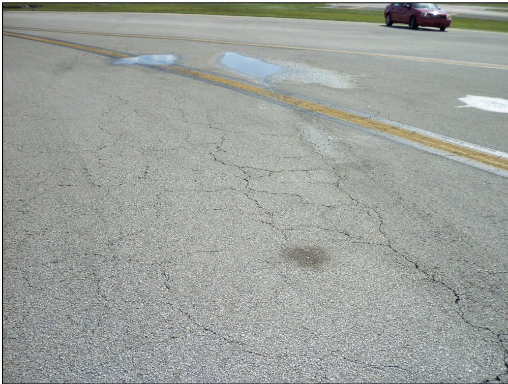
Taxiway T, Section 2010, Sample Unit 207 – Low severity (41) Alligator Cracking, low severity (43) Block Cracking, low severity (45) Depression, medium severity (52) Weathering and Raveling
