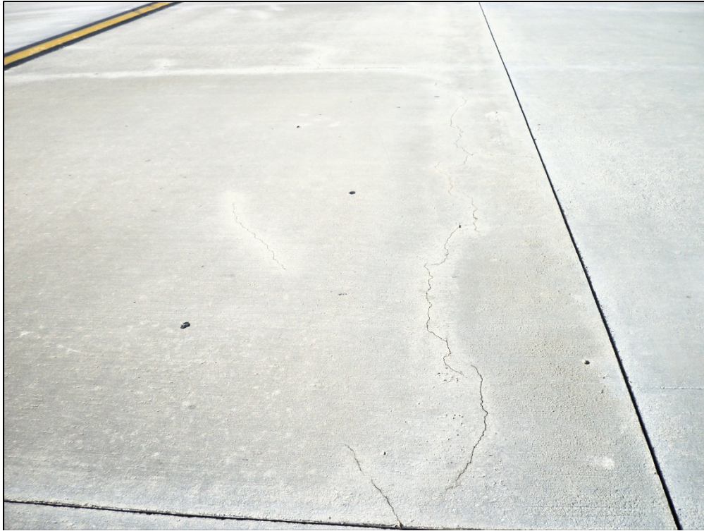
Common Aprons, Section 4080, Sample Unit 734 – (73) Shrinkage Cracking
