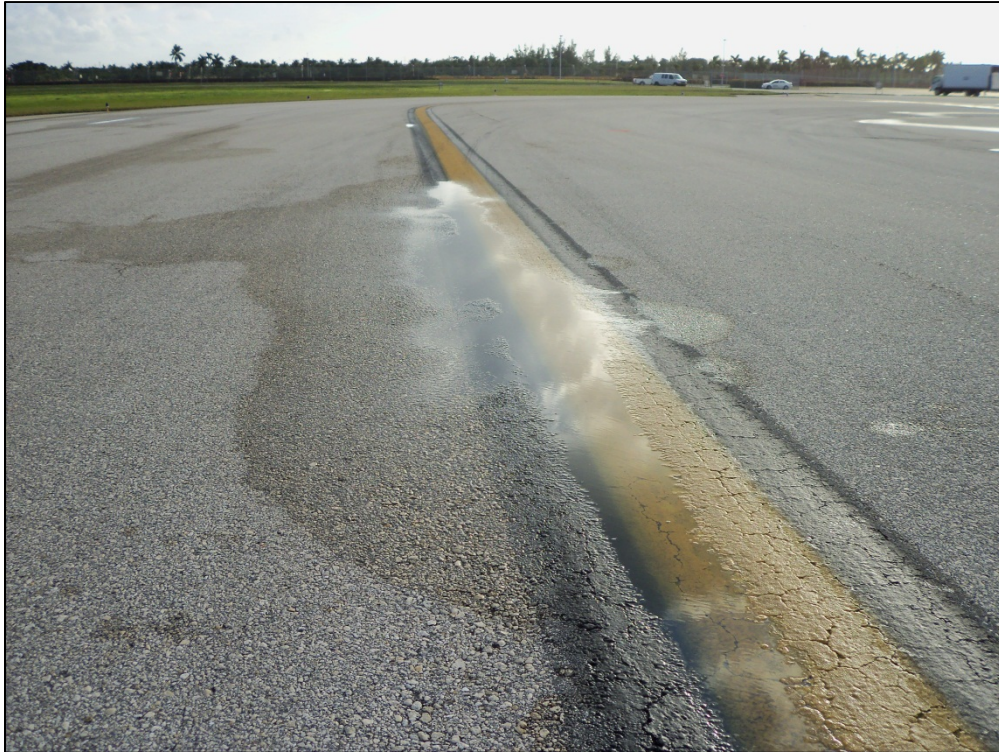
Taxiway B6, Section 290, Sample Unit 207 – Low severity (48) Longitudinal and Transverse Cracking, low severity (52) Weathering and Raveling, low severity (53) Rutting
