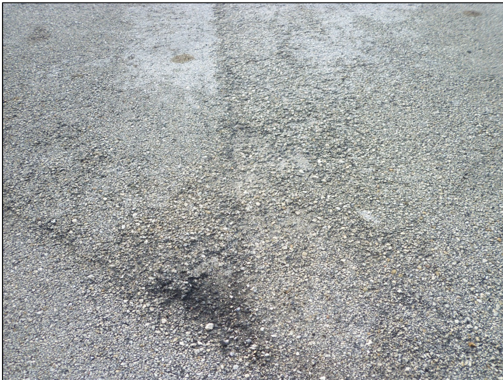
Common Aprons, Section 4045, Sample Unit 244 – Medium and high severity (52) Weathering and Raveling
