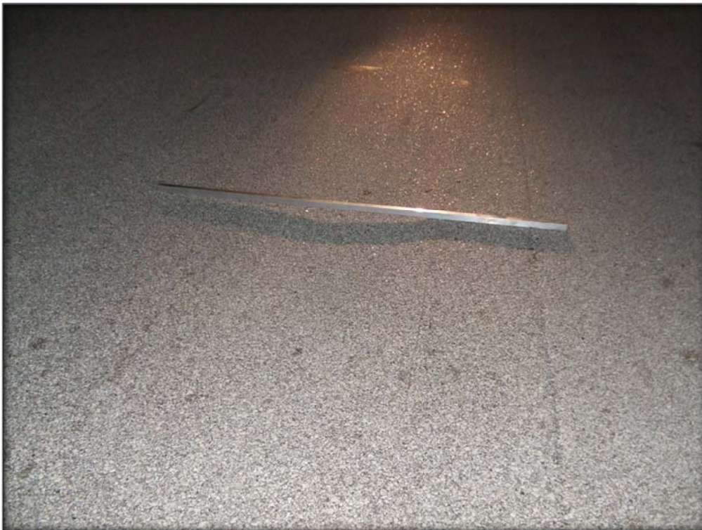
Taxiway B, Section 205, Sample Unit 513 – Low severity (52) Weathering and Raveling, High severity (53) Rutting
