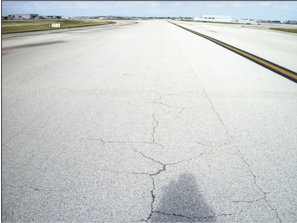
Taxiway D, Section 450, Sample Unit 514 – Medium severity (52) Weathering and Raveling, low severity (48) Longitudinal and Transverse Cracking, low severity (43) Block Cracking
