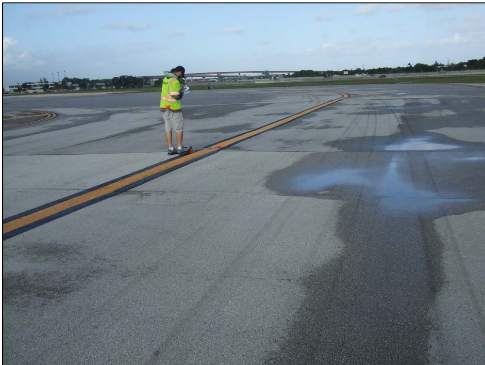
Taxiway A, Section 415, Sample Unit 406 – Low severity (50) Patching, Low severity (52) Weathering and Raveling, Low severity (48) Longitudinal and Transverse Cracking
