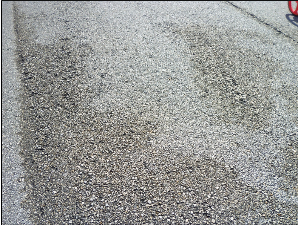
Taxiway T, Section 2005, Sample Unit 194 – Medium severity (52) Weathering and Raveling, low severity (48) Longitudinal and Transverse Cracking
