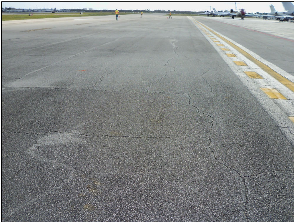
Taxiway E, Section 524, Sample Unit 811 – Low severity (43) Block Cracking, low severity (52) Weathering and Raveling
