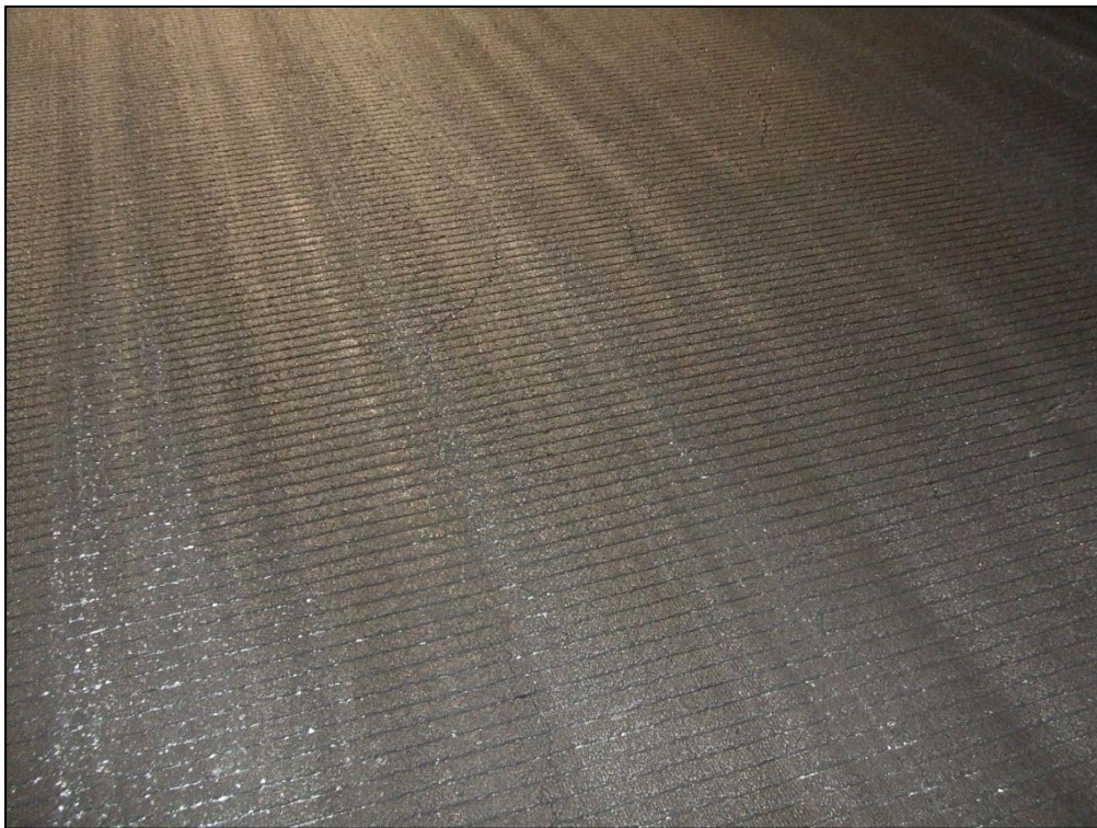
Runway 9L-27R, Section 6145, Sample Unit 364 – Low severity (52) Weathering and Raveling, Low severity (48) Longitudinal and Transverse Cracking
