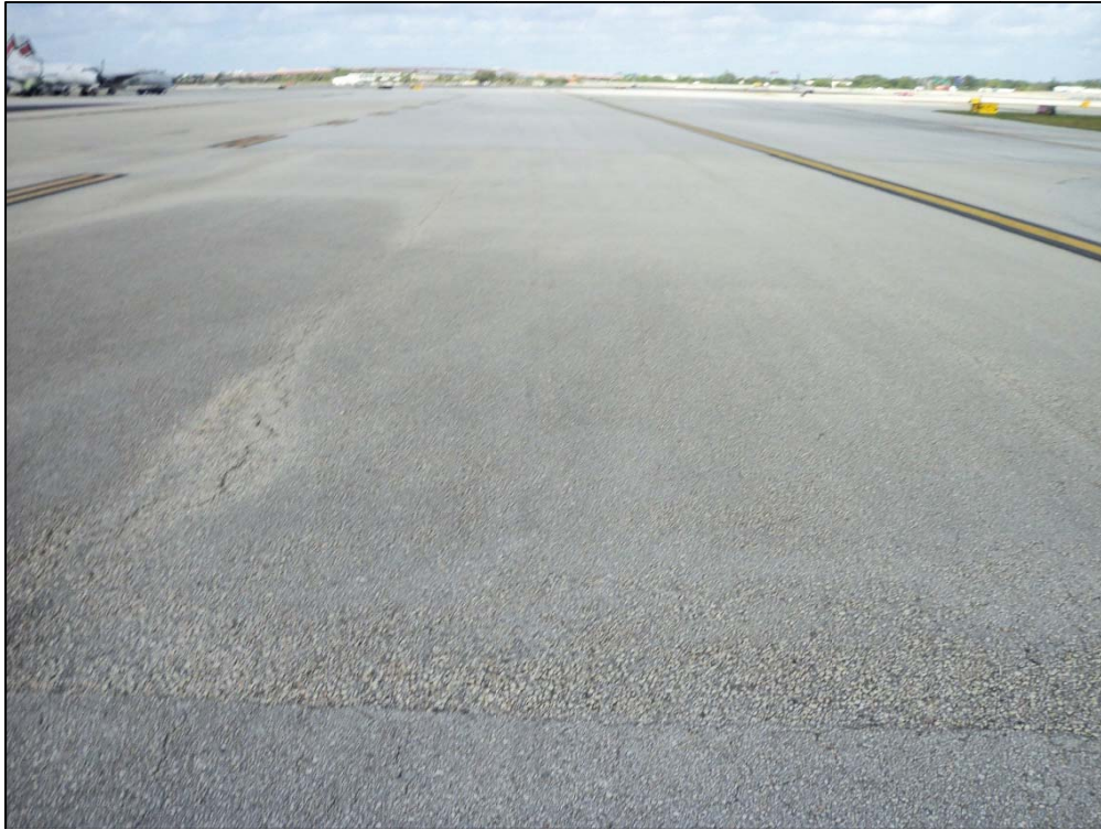
Taxiway E, Section 525, Sample Unit 646 – Low severity (48) Longitudinal and Transverse Cracking, low severity (52) Weathering and Raveling
