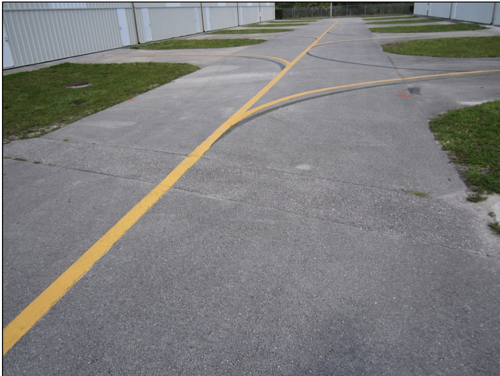
T-Hangar Apron E, Section 4420, Sample Unit 706 – Low severity (52) Weathering and Raveling, low severity (50) Patching
