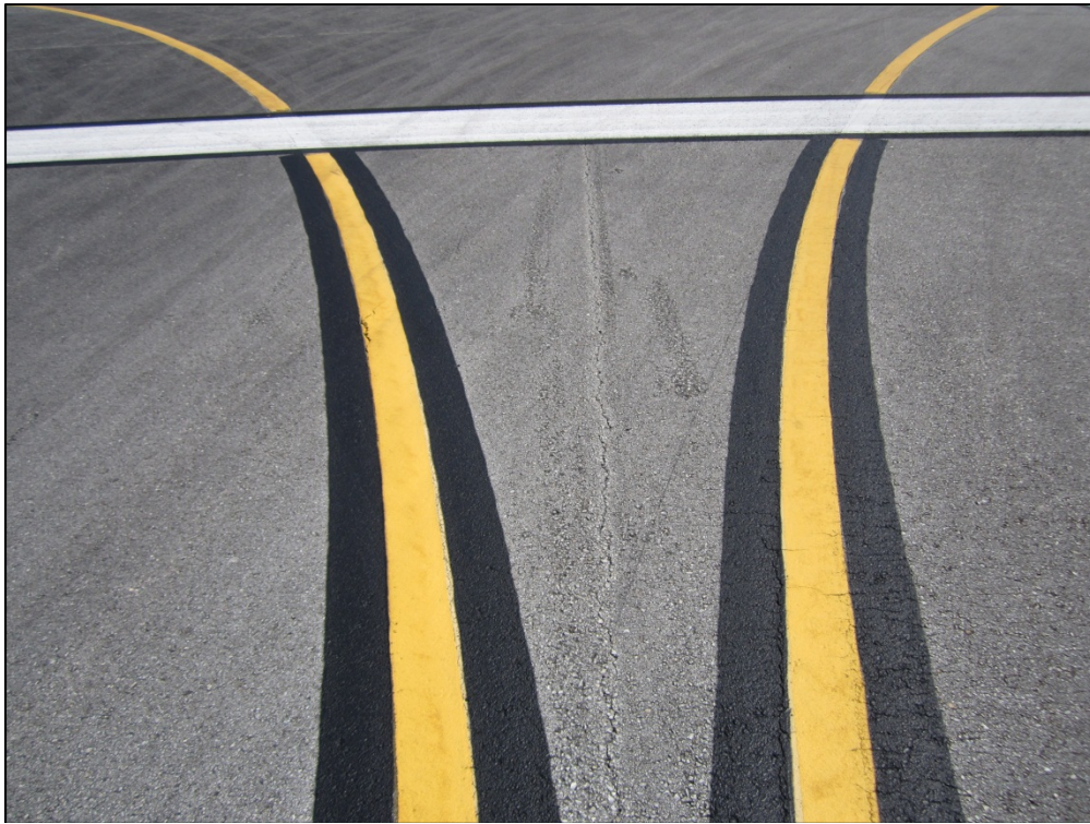
Taxiway Oscar, Section 1505, Sample Unit 400 – Low severity (48) Longitudinal and Transverse Cracking, low and medium severity (52) Weathering and Raveling
