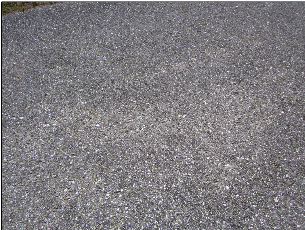
T-Hangar Apron N, Section 4305, Sample Unit 801 – Low severity (52) Weathering and Raveling
