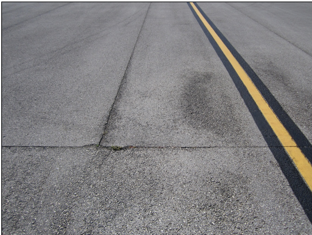
North Apron, Section 4105, Sample Unit 704 – Low severity (48) Longitudinal and Transverse Cracking, low and medium severity (52) Weathering and Raveling
