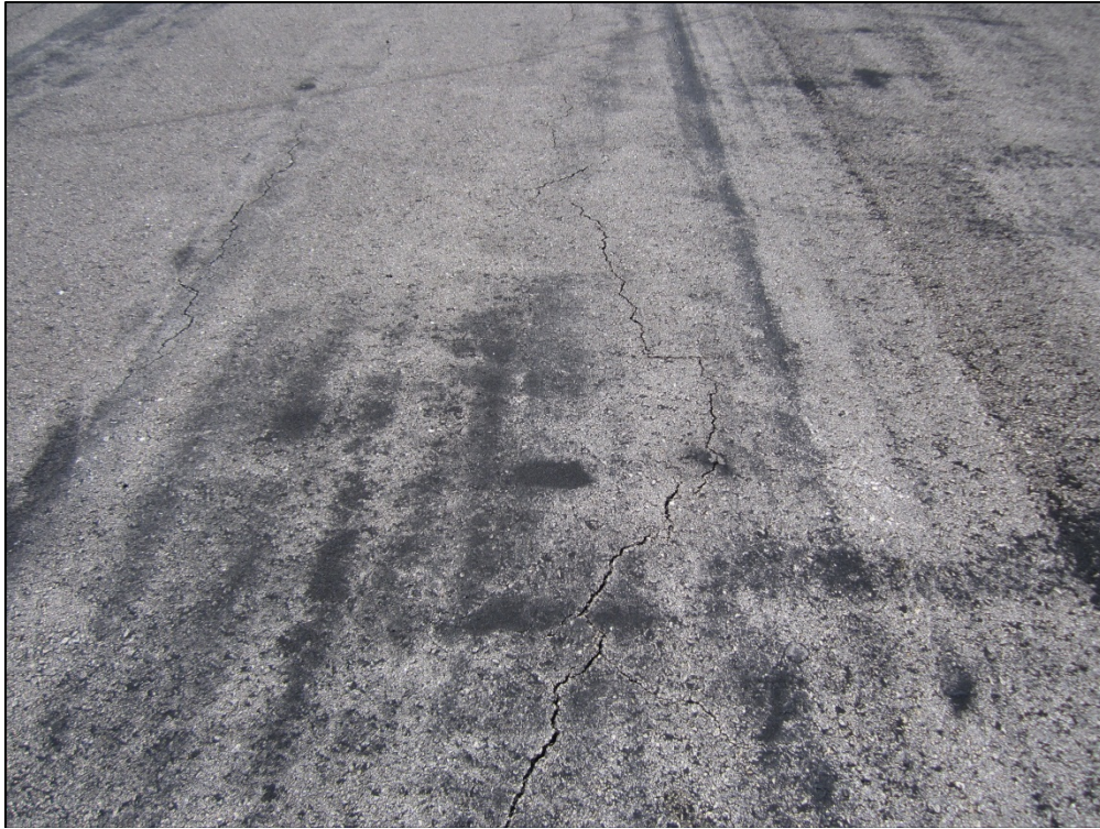
North Apron, Section 4120, Sample Unit 206 – Low severity (48) Longitudinal and Transverse Cracking, low severity (52) Weathering and Raveling, low severity (56) Swelling
