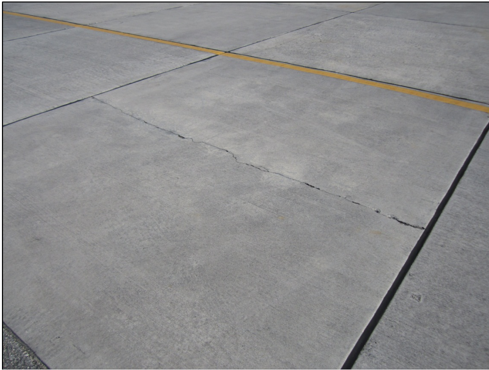
North Apron, Section 4115, Sample Unit 751 – low severity (63) Longitudinal, Transverse and Diagonal Cracking
