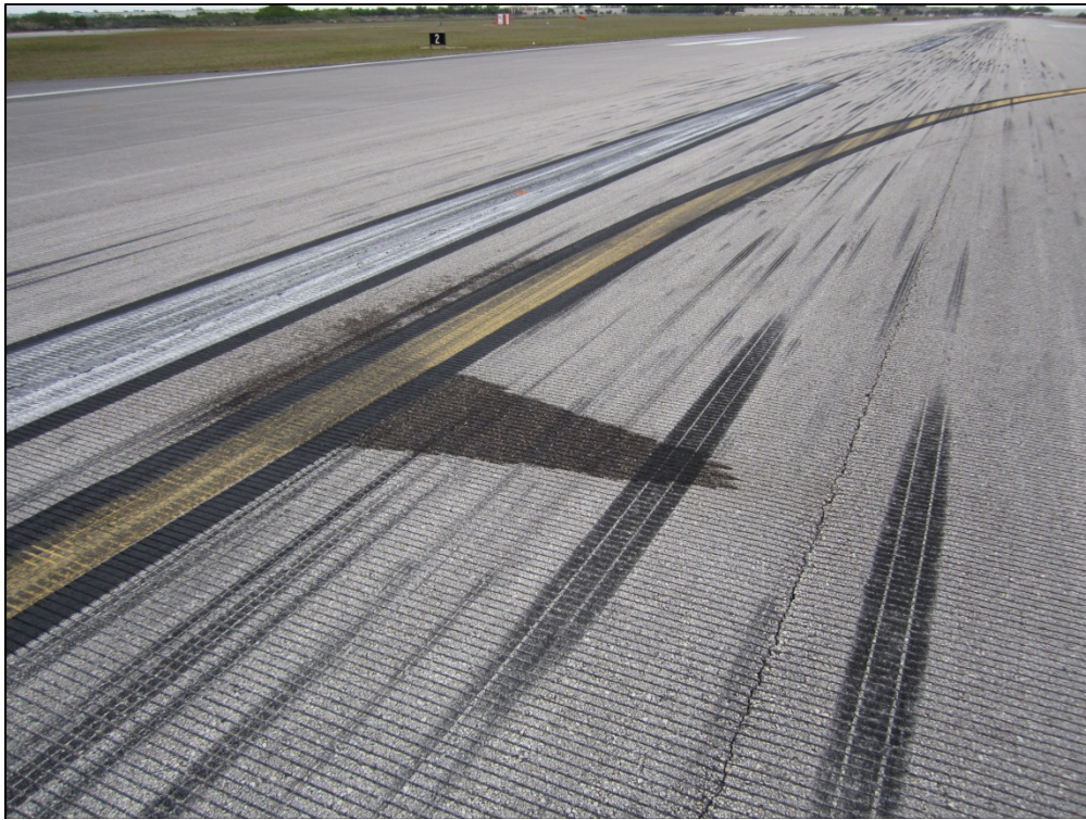
Runway 12-30, Section 6205, Sample Unit 351 – Low and medium severity (48) Longitudinal and Transverse Cracking, low severity (52) Weathering and Raveling, (49) Oil Spillage
