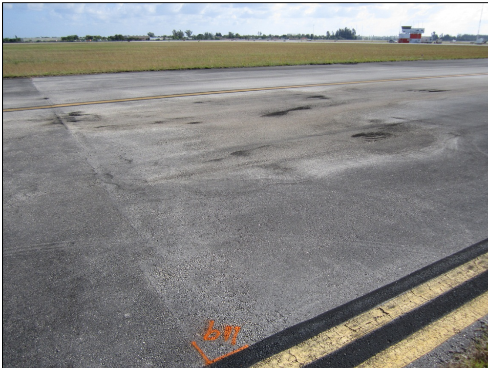
Taxiway Sierra, Section 1920, Sample Unit 109 – Medium severity (45) Depression, low severity (48) Longitudinal and Transverse Cracking, low severity (52) Weathering and Raveling
