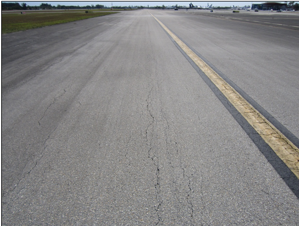
Taxiway November, Section 1423, Sample Unit 211 – Low severity (43) Block Cracking, low severity (41) Alligator Cracking, low severity (53) Rutting, low severity (52) Weathering and Raveling, low severity (48) Longitudinal and Transverse Cracking
