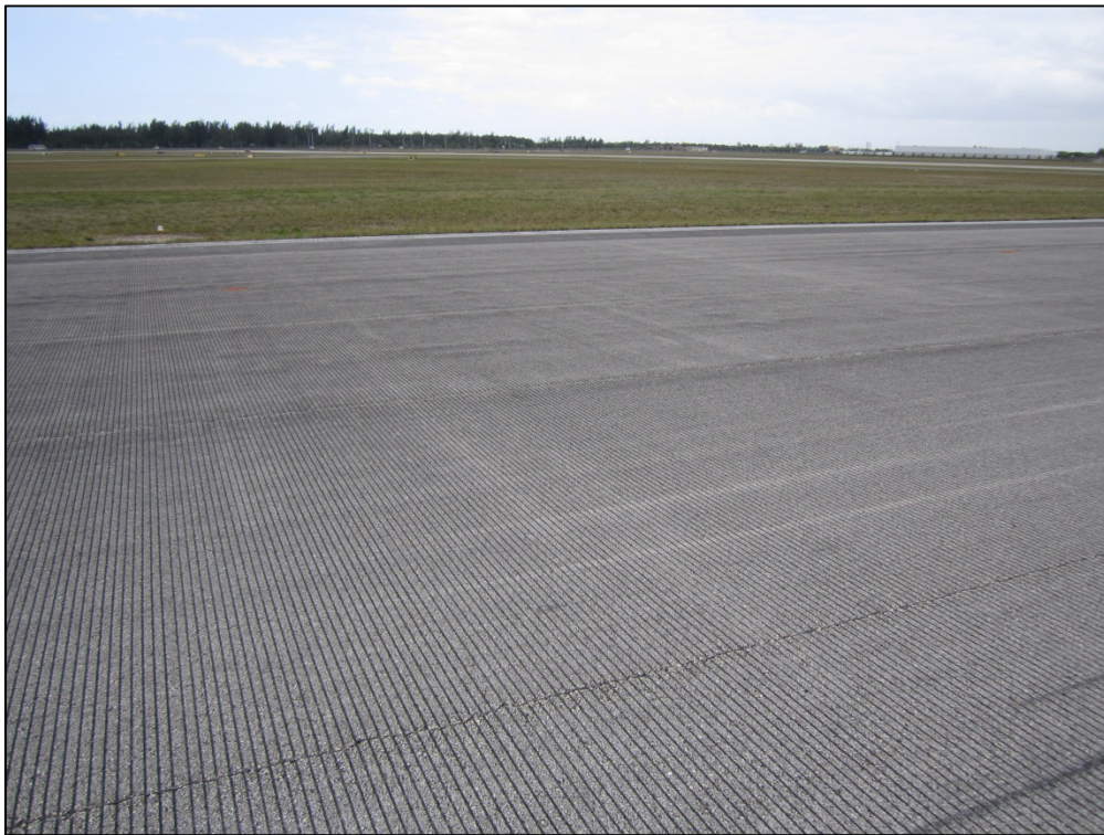
Runway 12-30, Section 6205, Sample Unit 399 – Low severity (56) Swelling, low severity (52) Weathering and Raveling, low and medium severity (48) Longitudinal and Transverse Cracking
