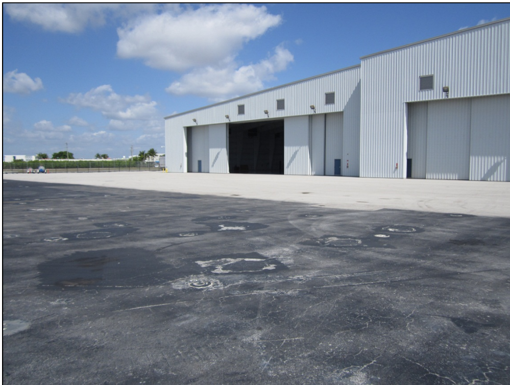
T-Hangar Apron, Section 4507, Sample Unit 262 – Low severity (43) Block Cracking; low severity (52) Weathering and Raveling; low, medium, and high severity (50) Patching
