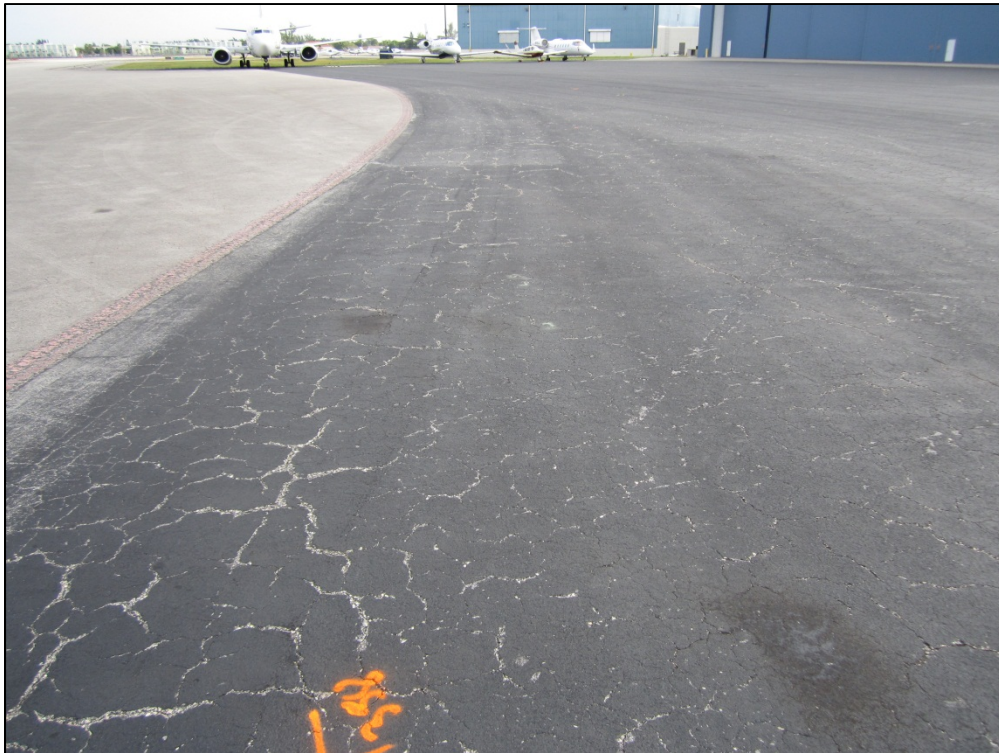
East Apron, Section 4210, Sample Unit 358 – Low severity (43) Block Cracking, low severity (52) Weathering and Raveling
