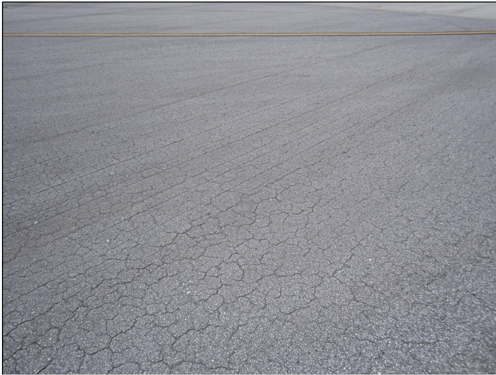
Taxiway Papa, Section 1660, Sample Unit 358 – Low severity (45) Depression, low severity (43) Block Cracking, low severity (52) Weathering and Raveling
