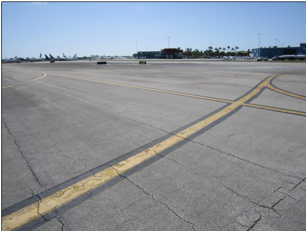
Taxiway November, Section 1423, Sample Unit 221 – Medium severity (43) Block Cracking, low severity (52) Weathering and Raveling, low severity (45) Depression, low severity (53) Rutting
