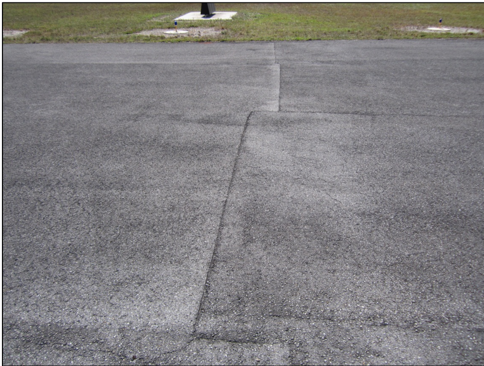
Taxiway Y-2, Section 1060, Sample Unit 304 – Low severity (48) Longitudinal and Transverse Cracking, low and medium severity (52) Weathering and Raveling
