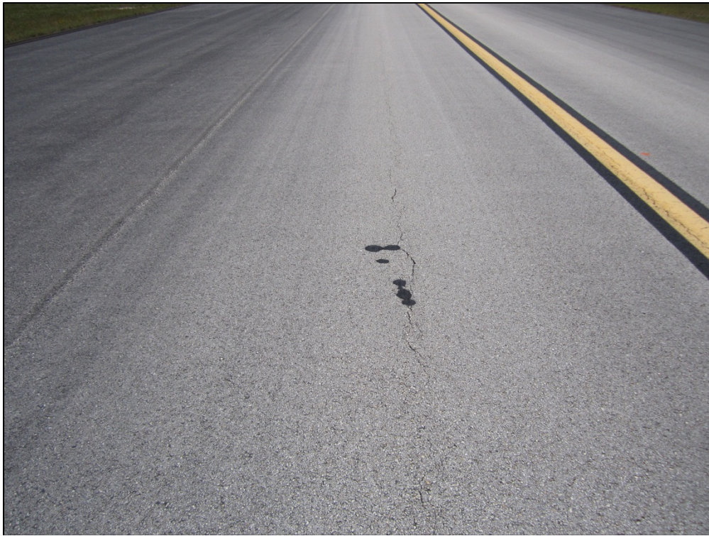
Taxiway Tango, Section 2005, Sample Unit 119 – Low severity (48) Longitudinal and Transverse Cracking, low severity (52) Weathering and Raveling
