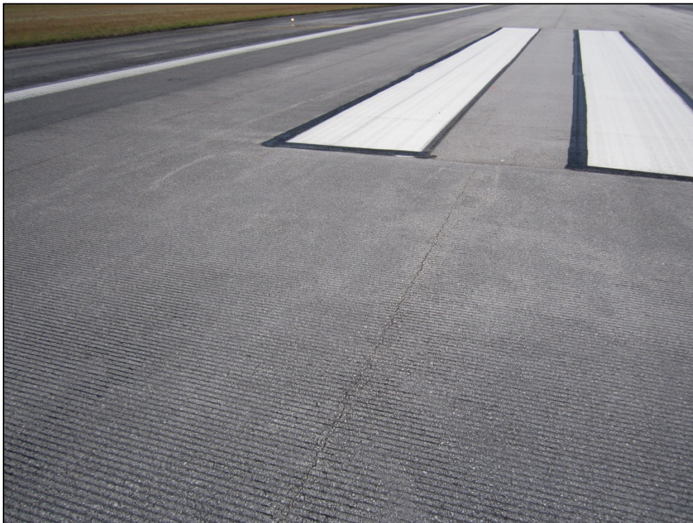
Runway 9L-27R, Section 6130, Sample Unit 564 – Low severity (48) Longitudinal and Transverse Cracking, low severity (50) Patching, low severity (52) Weathering and Raveling
