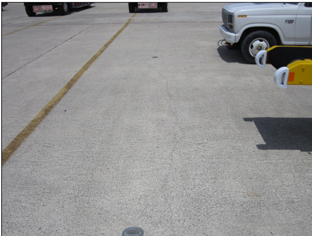
Center Apron, Section 4120, Sample Unit 601 – Low severity (72) Shattered Slab
