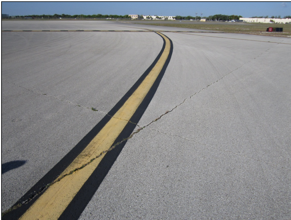
Taxiway November, Section 1412, Sample Unit 201 – Low and medium severity (47) Joint Reflection Cracking, low severity (52) Weathering and Raveling
