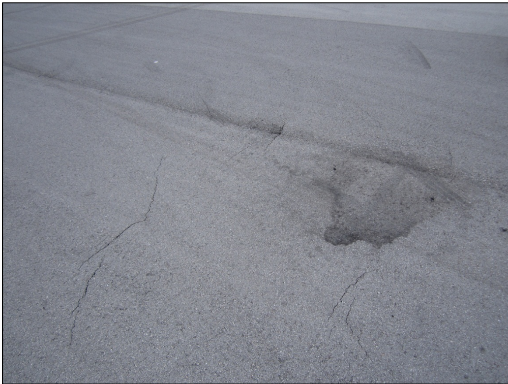
Taxiway Hotel, Section 6315, Sample Unit 324 – Low severity (48) Longitudinal and Transverse Cracking, (49) Oil Spillage
