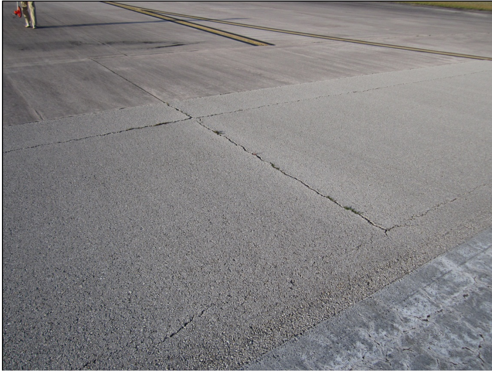
Taxiway November, Section 1437, Sample Unit 698 – Low and medium severity (47) Joint Reflection Cracking, low severity (48) Longitudinal and Transverse Cracking, low severity (52) Weathering and Raveling
