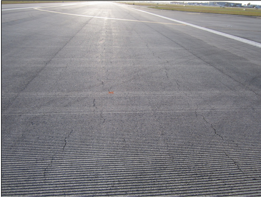
Runway 9L-27R, Section 6120, Sample Unit 531 – Low severity (48) Longitudinal and Transverse Cracking, low severity (52) Weathering and Raveling
