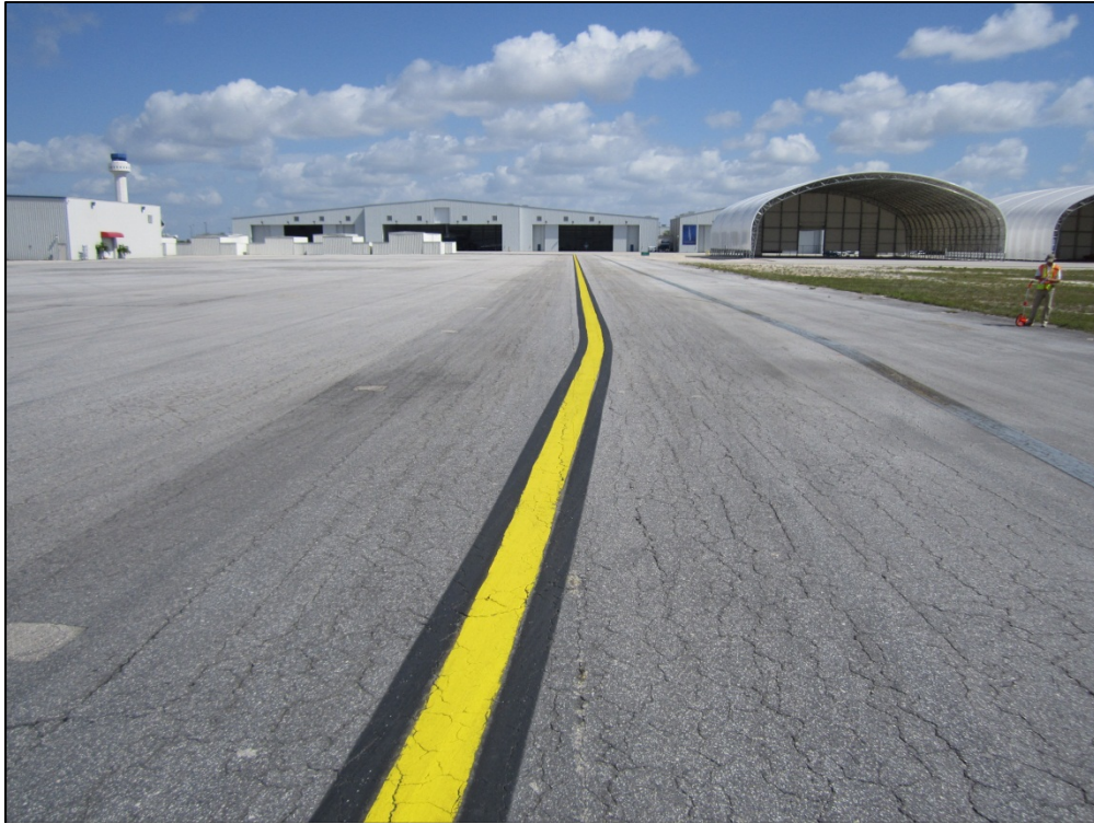
T-Hangar Apron, Section 4510, Sample Unit 105 – Medium severity (50) Patching, low severity (43) Block Cracking, low and medium severity (53) Rutting, low severity (45) Depression, low severity (52) Weathering and Raveling
