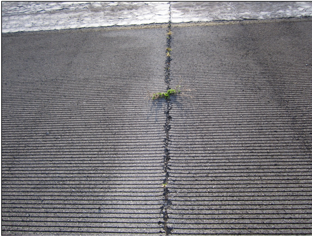
Runway 9L-27R, Section 6130, Sample Unit 179 – High severity (48) Longitudinal and Transverse Cracking, low severity (52) Weathering and Raveling
