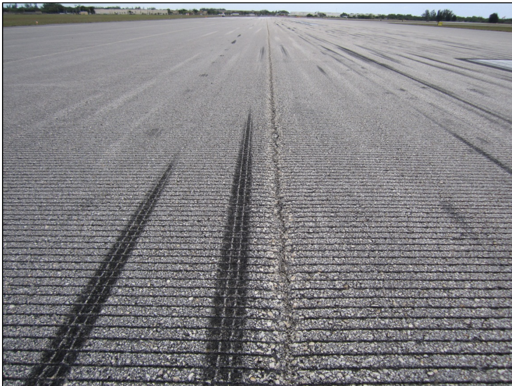
Runway 12-30, Section 6205, Sample Unit 326 – Low and medium severity (48) Longitudinal and Transverse Cracking, low severity (52) Weathering and Raveling
