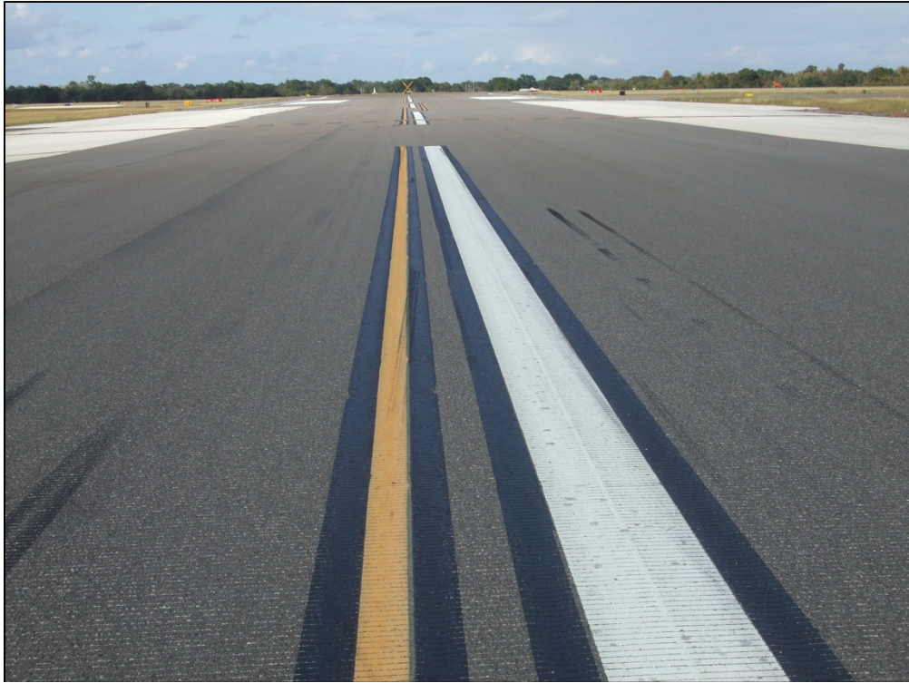
Runway 18-36, Section 6280, Sample Unit 385 – Low severity (52) Weathering and Raveling
