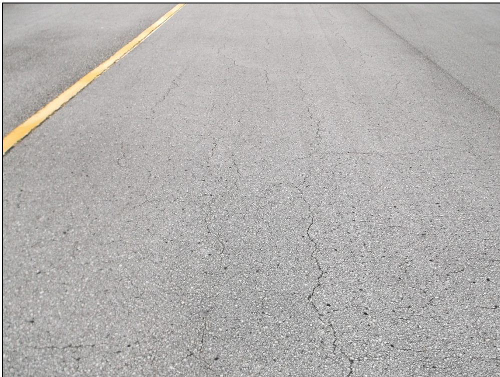
Taxiway Connector B-2, Section 215, Sample Unit 203 – Low Severity (48) Longitudinal and Transverse Cracking, low severity (52) Weathering and Raveling
