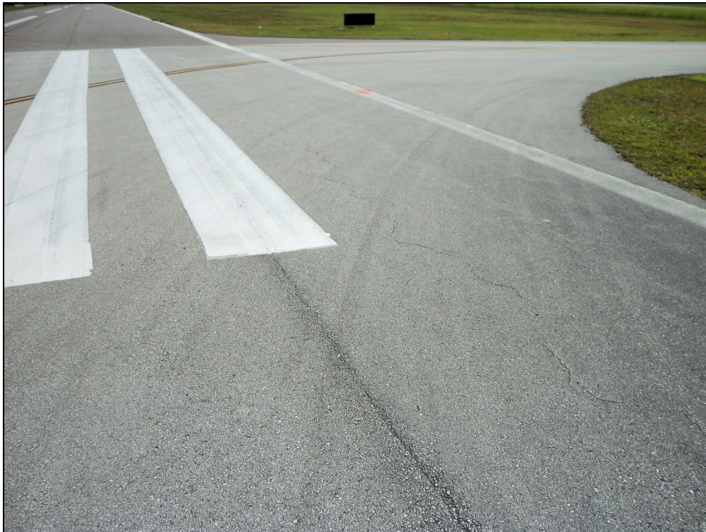
Runway 9R-27L, Section 6405, Sample Unit 172 – Low Severity (48) Longitudinal and Transverse Cracking and low severity (52) Weathering and Raveling
