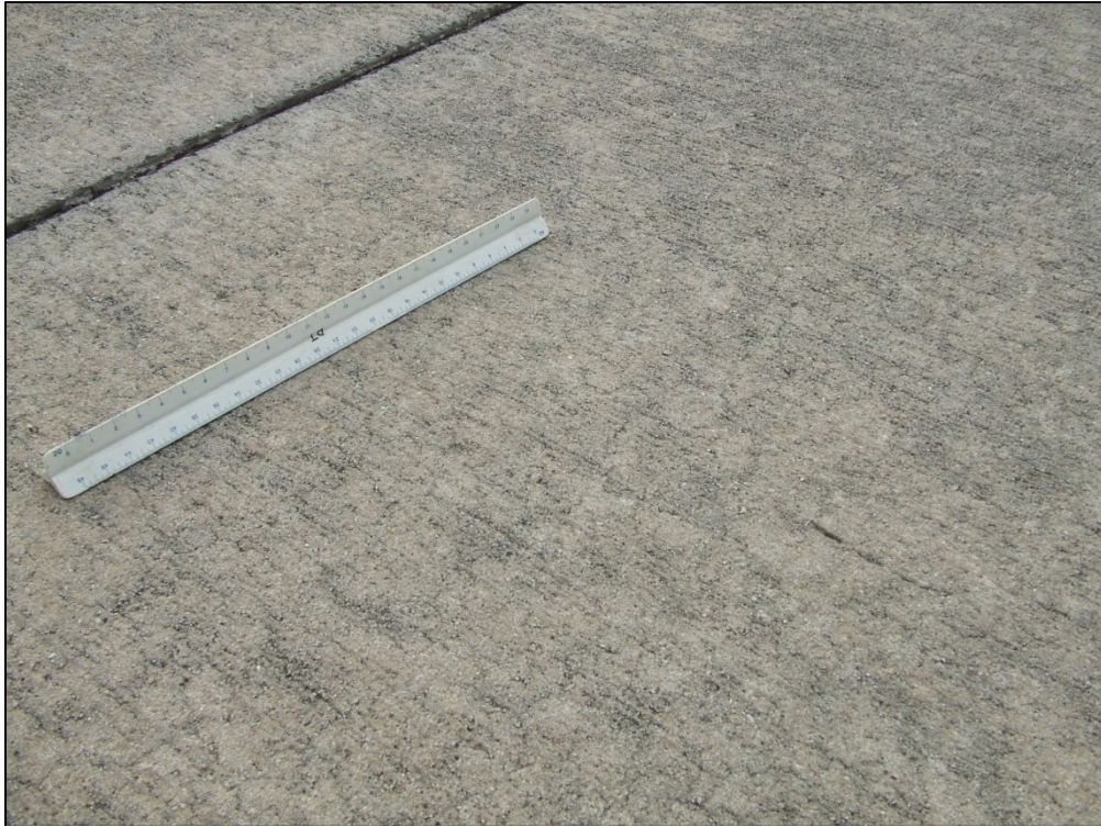
Terminal Apron, Section 4120, Sample Unit 502 – Low severity (70) Scaling, Crazing and Map Cracking
