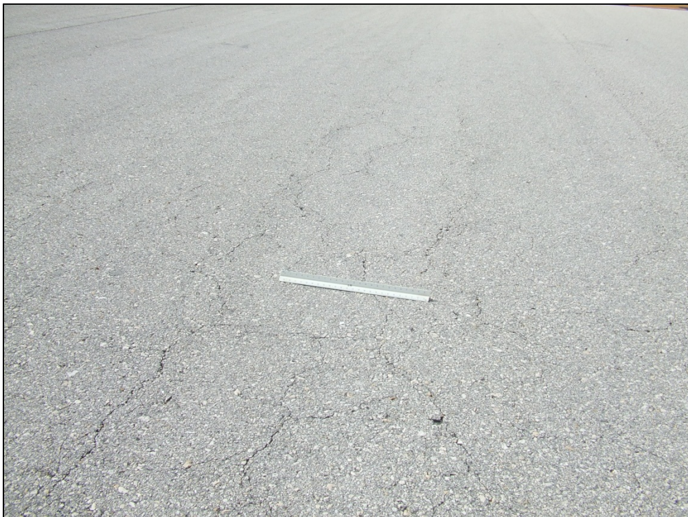
Taxiway Charlie, Section 320, Sample Unit 302 – Low severity (52) Weathering and Raveling, Low severity (43) Block Cracking
