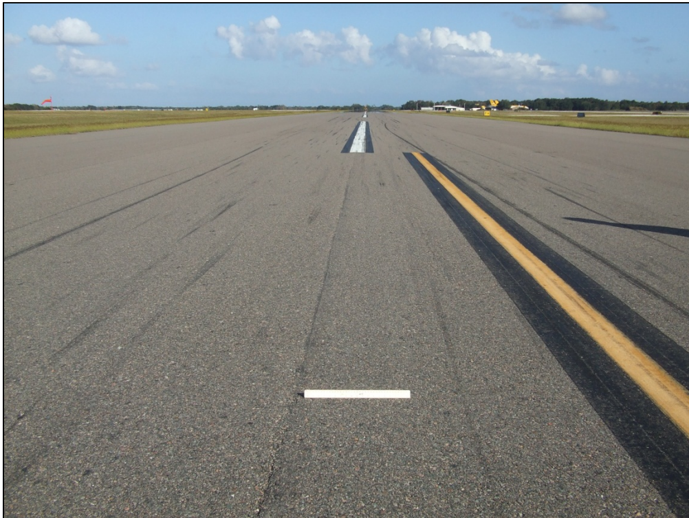
Runway 9C-27C, Section 6305, Sample Unit 147 – Low severity (48) Longitudinal and Transverse Cracking, Low severity (52) Weathering and Raveling
