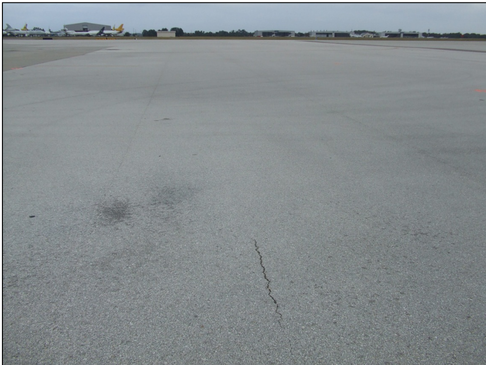
Terminal Apron, Section 4140, Sample Unit 560 – Low severity (48) Longitudinal and Transverse Cracking, (49) Oil Spillage, Low severity (52) Weathering and Raveling
