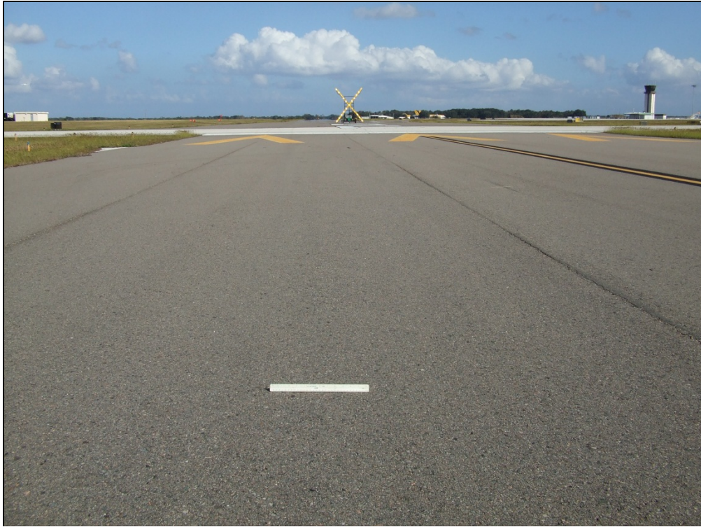
Taxiway K-1, Section 1005, Sample Unit 114 – Low severity (56) Swelling, Low severity (48) Longitudinal and Transverse Cracking, Low severity (52) Weathering and Raveling
