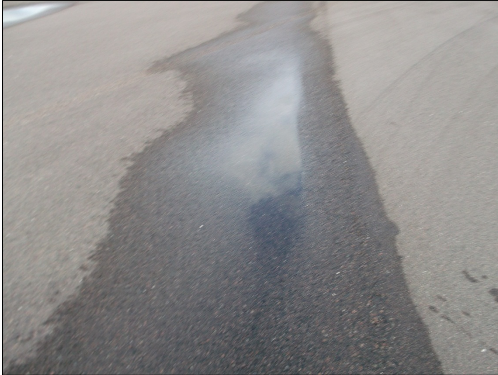
Taxiway Bravo, Section 202, Sample Unit 336 – Low Severity (45) Depression
