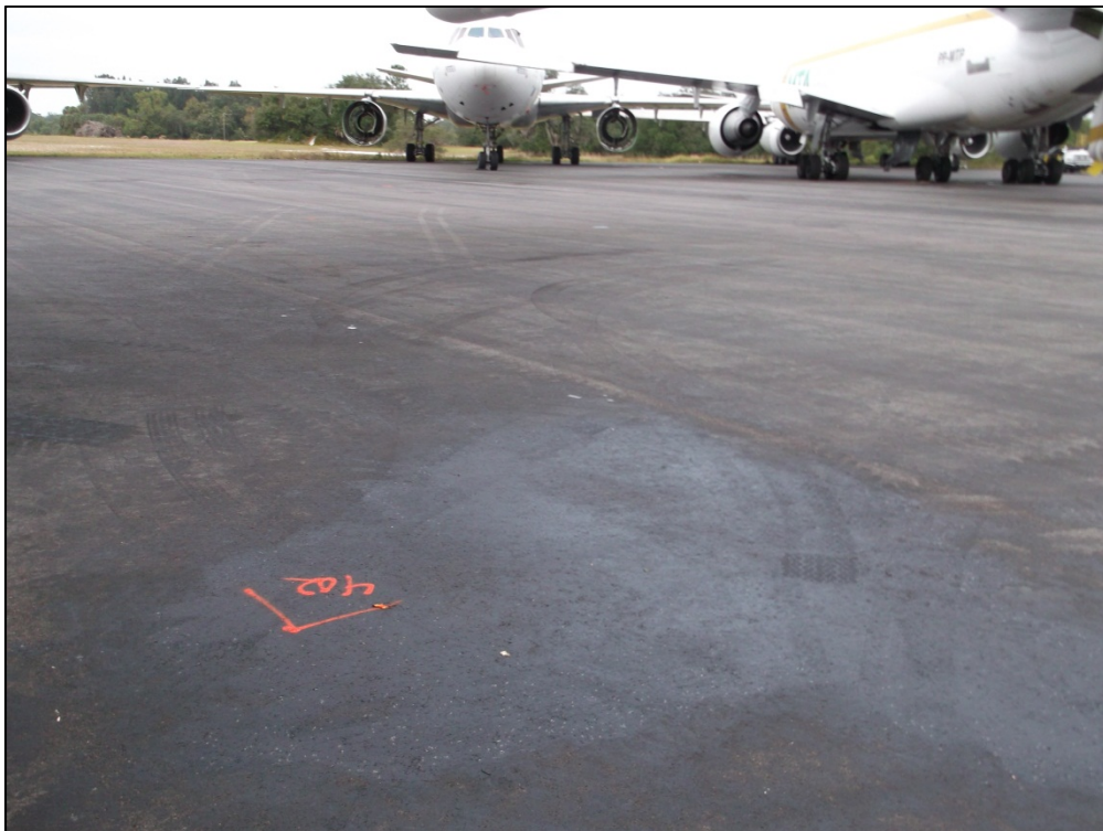
North Apron, Section 4310, Sample Unit 402 – (49) Oil Spillage
