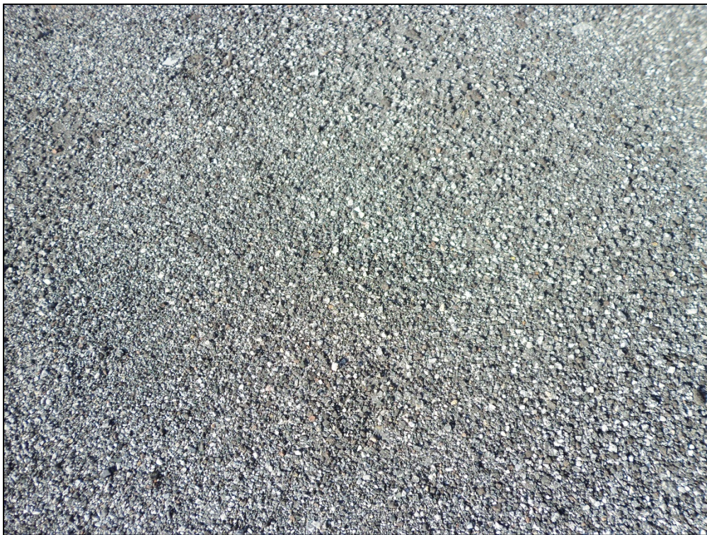
Southwest Apron, Section 4210, Sample Unit 907 – High Severity (52) Weathering and Raveling
