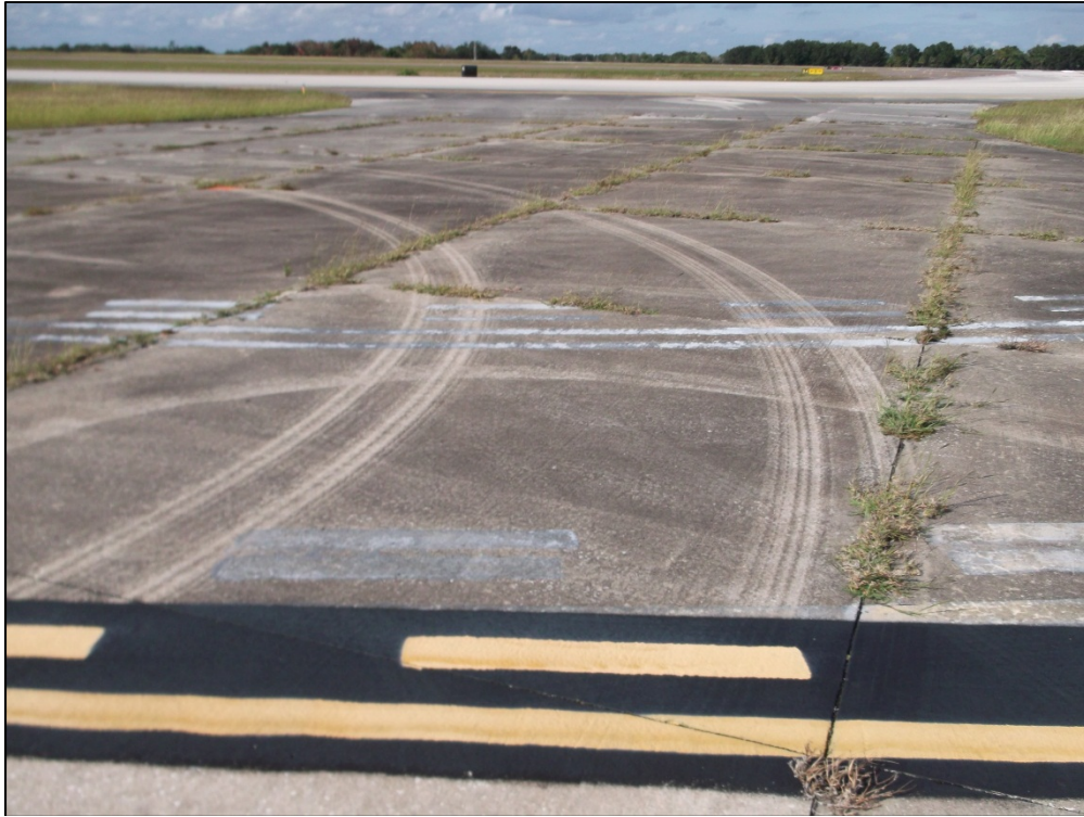
East Apron, Section 4505, Sample Unit 400 – Medium Severity (65) Joint Seal Damage
