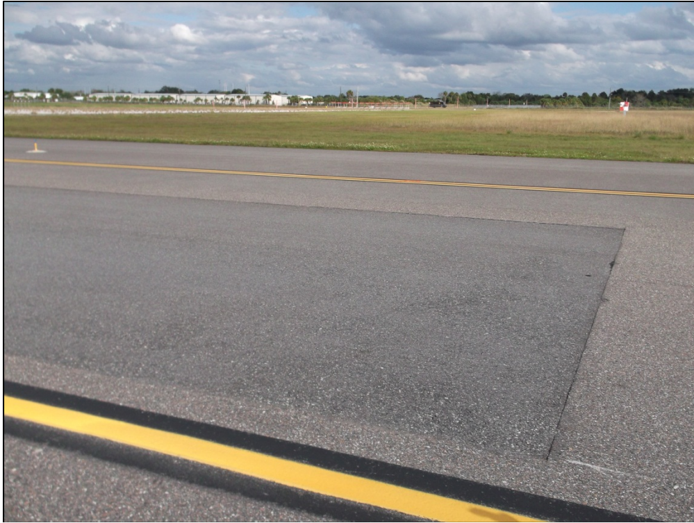
Taxiway Bravo, Section 610, Sample Unit 120 – Low Severity (50) Patch
