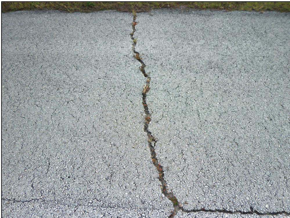
FBO Apron Connector, Section 105, Sample Unit 105 – High Severity (48) Longitudinal and Transverse Cracking, low severity (52) weathering and raveling
