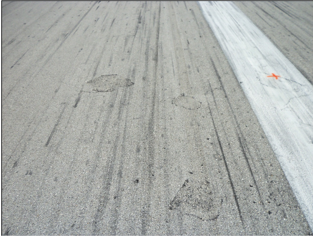
Runway 9R-27L, Section 6405, Sample Unit 145 – Low Severity (48) Longitudinal and Transverse Cracking, Medium and Low Severity (50) Patch and Low Severity (52) Weathering and Raveling
