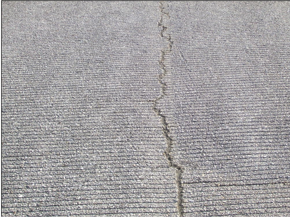
Runway 18-36, Section 6210, Sample Unit 540 – Low and medium severity (48) Longitudinal and Transverse Cracking, Low severity (56) Swelling, Low severity (52) Weathering and Raveling
