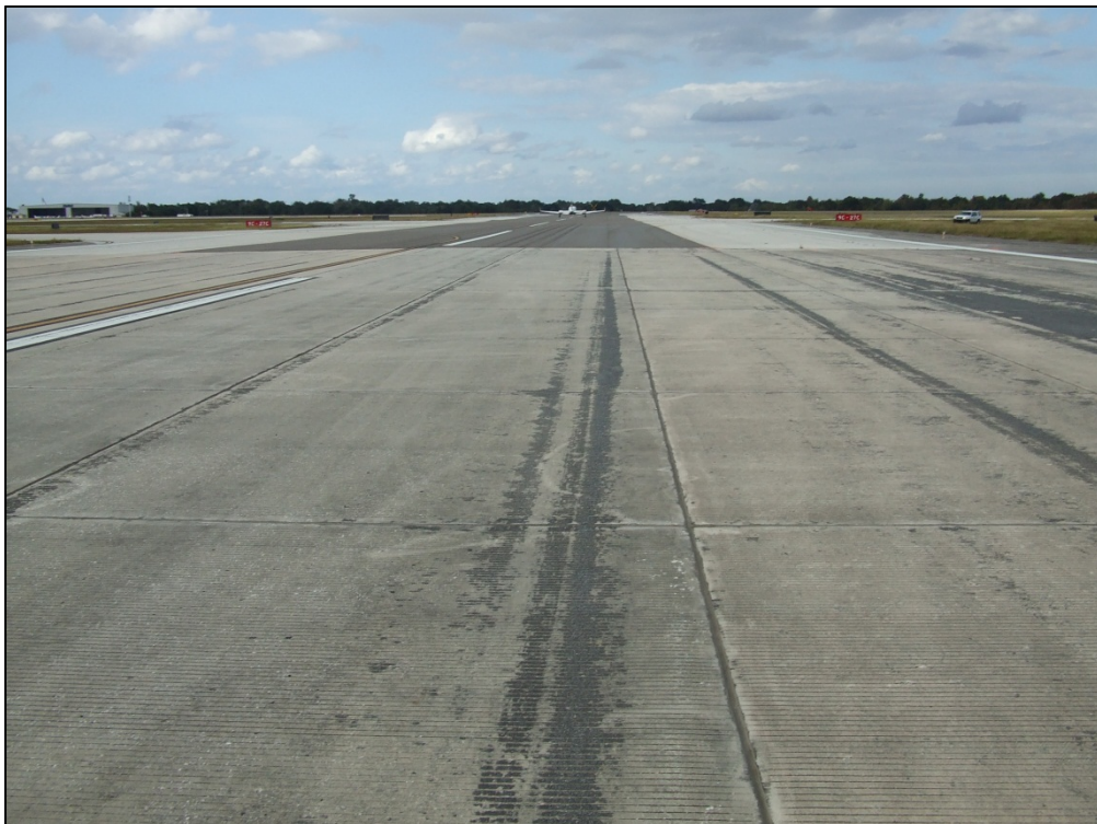
Runway 18-36, Section 6215, Sample Unit 372 – Low severity (70) Scaling, Crazeing and Map Cracking, (73) Shrinkage Cracking
