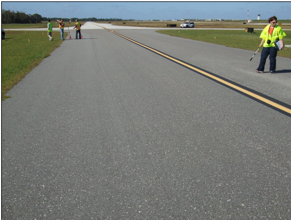
Taxiway Sierra, Section 1925, Sample Unit 201 – Low severity (52) Weathering and Raveling
