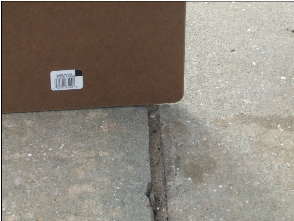
Terminal Apron, Section 4110, Sample Unit 504 – Low severity (74) Joint Spalling, Low severity (71) Faulting
