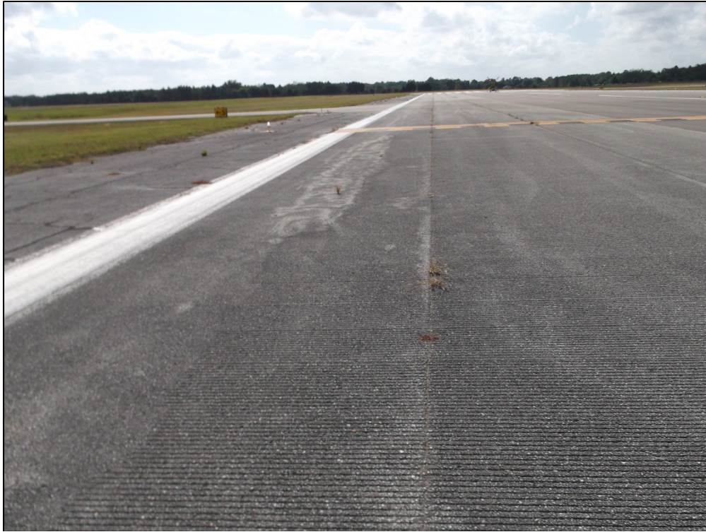
Runway 18-36, Section 6210, Sample Unit 516 – Medium Severity (48) Longitudinal and Transverse Cracking, low severity (52) weathering and raveling
