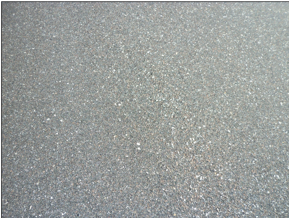
Runway 9R-27L, Section 6405, Sample Unit 145 –Low Severity (52) Weathering and Raveling
