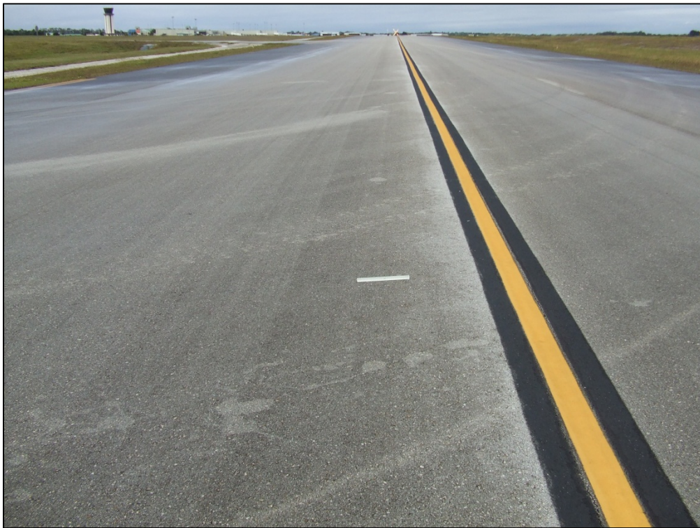
Taxiway Charlie, Section 350, Sample Unit 134 – Low severity (52) Weathering and Raveling, Low severity (48) Longitudinal and Transverse Cracking
