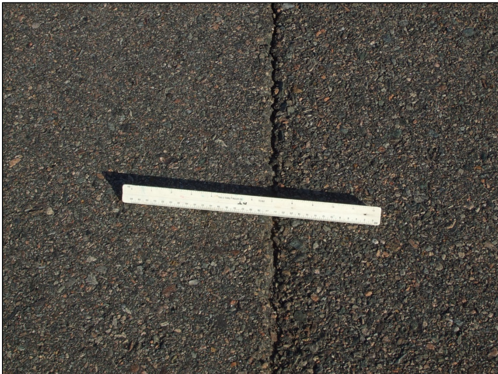
Runway 9C-27C, Section 6305, Sample Unit 125 – Low severity (48) Longitudinal and Transverse Cracking, Low severity (52) Weathering and Raveling
