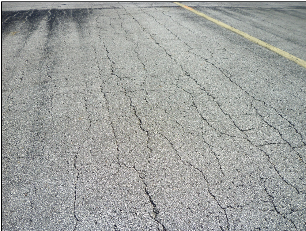
Taxiway Hotel, Section 810, Sample Unit 112 – Low Severity (43) Block Cracking, low severity (52) Weathering and Raveling
