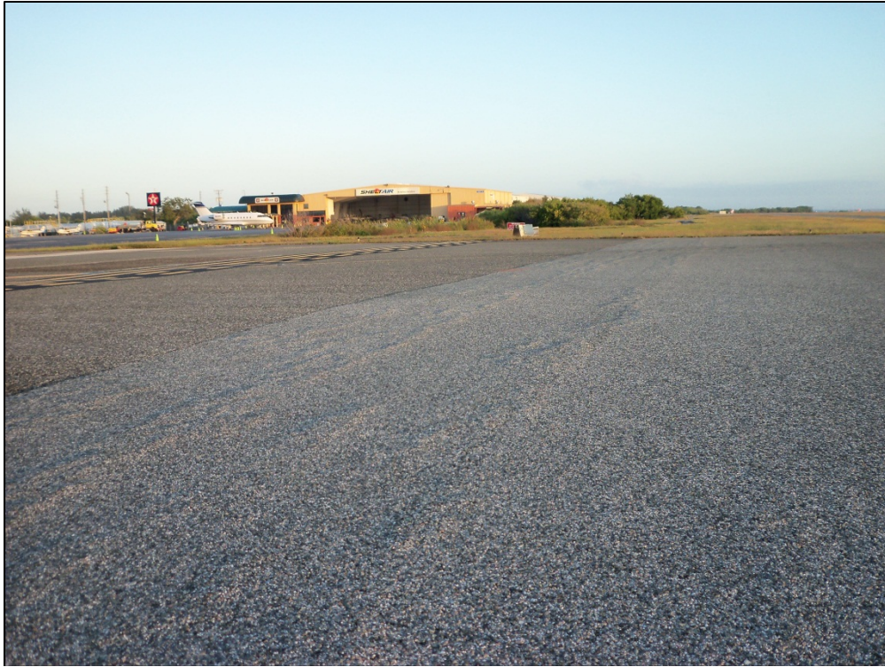
Taxiway Lima, Section 1220, Sample Unit 202 – Low Severity (56) Swelling
