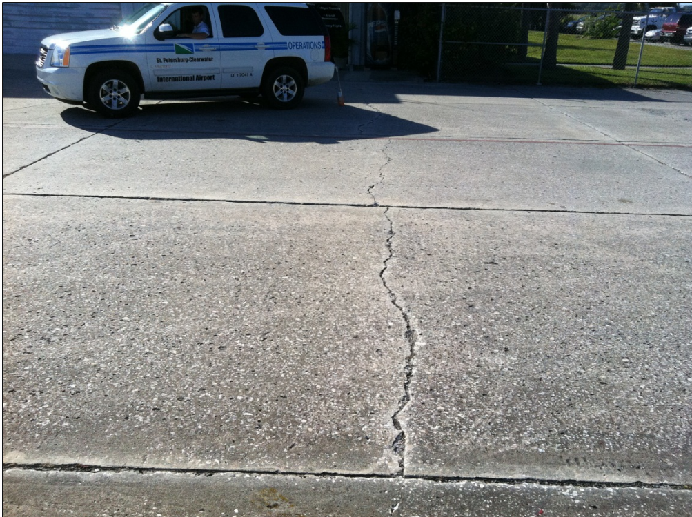
Main Apron, Section 4190, Sample Unit 101 – Medium Severity (63) Longitudinal, Transverse, and Diagonal Cracking
