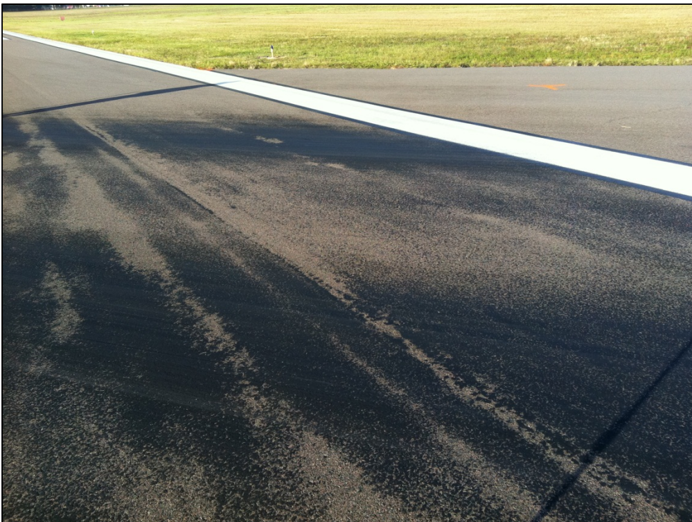
Runway 4-22, Section 6225, Sample Unit 212 – (42) Bleeding
