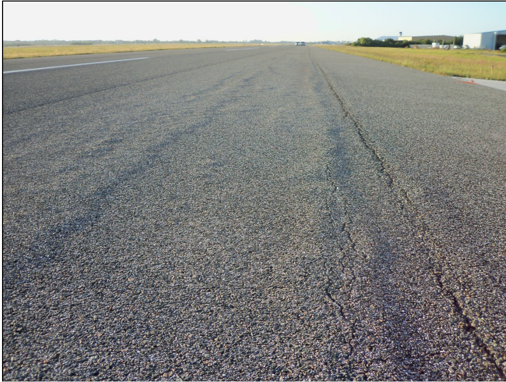
Runway 18R-36L, Section 6405, Sample Unit 375 – Low Severity (56) Swelling, low severity (48) Longitudinal and Transverse Cracking
