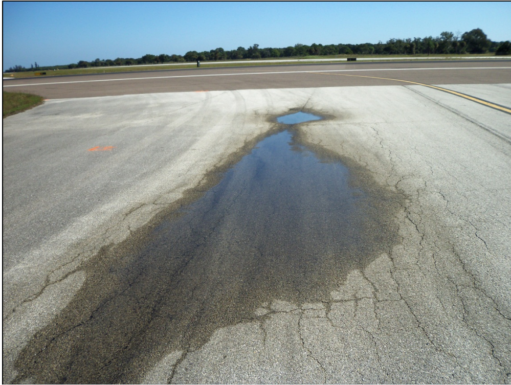
Taxiway Mike, Section 1310, Sample Unit 101 – Low Severity (45) Depression, low severity (43) Block Cracking, low severity (52) Weathering and Raveling
