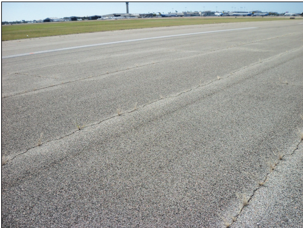
Runway 9-27, Section 6315, Sample Unit 338 – Low and Medium Severity (48) Longitudinal and Transverse Cracking, Low Severity (52) Weathering, Raveling
