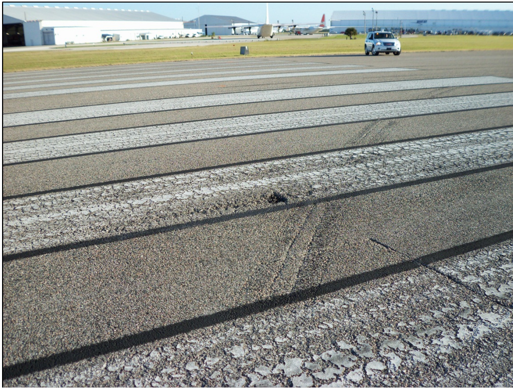
Runway 9-27, Section 6365, Sample Unit 400 – High Severity (52) Weathering, Raveling
