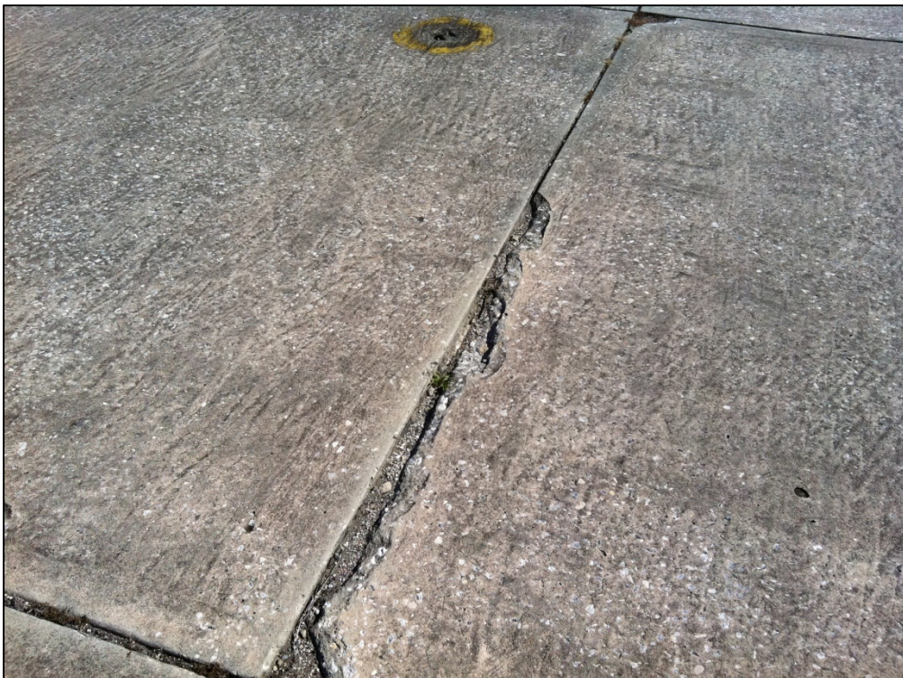
Main Apron, Section 4175, Sample Unit 403 – Medium Severity (74) Joint Spalling
