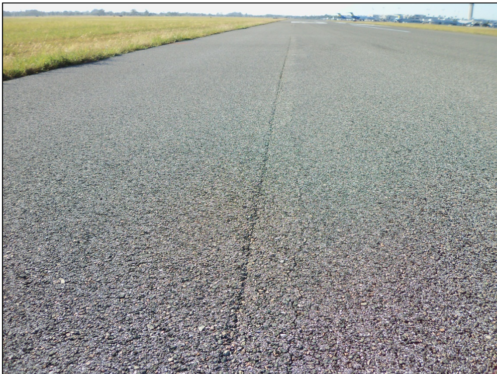
Runway 18R-36L, Section 130, Sample Unit 324 – Low Severity (56) Longitudinal and Transverse Cracking
