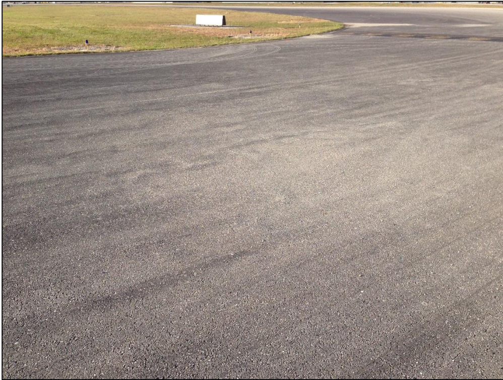
Taxiway Tango, Section 2010, Sample Unit 607 – Low Severity (45) Depression, Low Severity (52) Raveling, Low Severity (56) Swelling, Low Severity (57) Weathering
