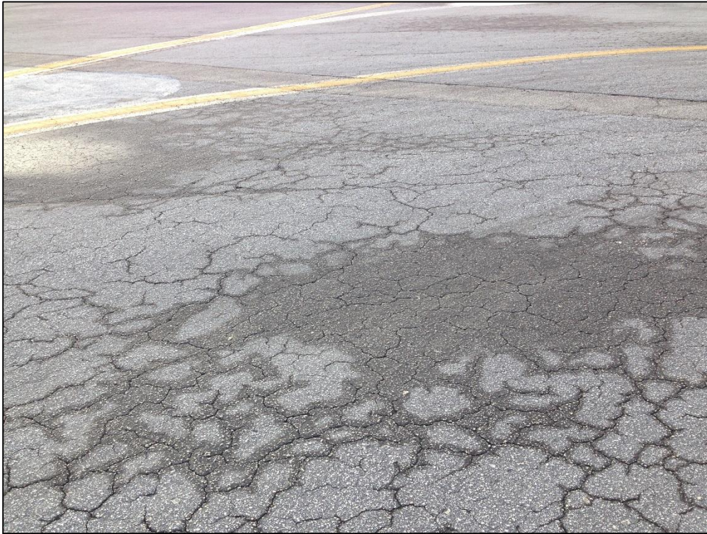
Taxiway Papa, Section 1660, Sample Unit 366 – Medium Severity (43) Block Cracking, Low Severity (45) Depression, Medium Severity (50) Patching, Low Severity (52) Raveling
