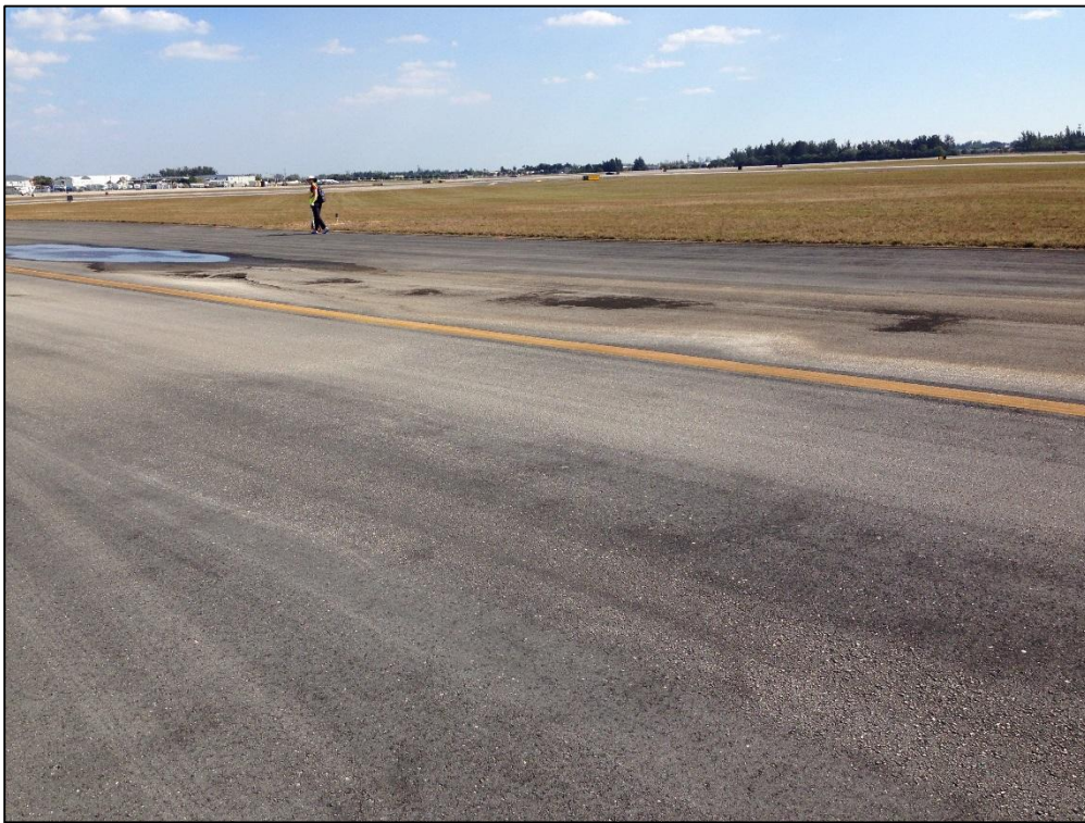
Taxiway Sierra, Section 1920, Sample Unit 109 – High Severity (45) Depression, Low Severity (52) Raveling, Low Severity (53) Rutting, Medium Severity (53) Rutting, Low Severity (57) Weathering
