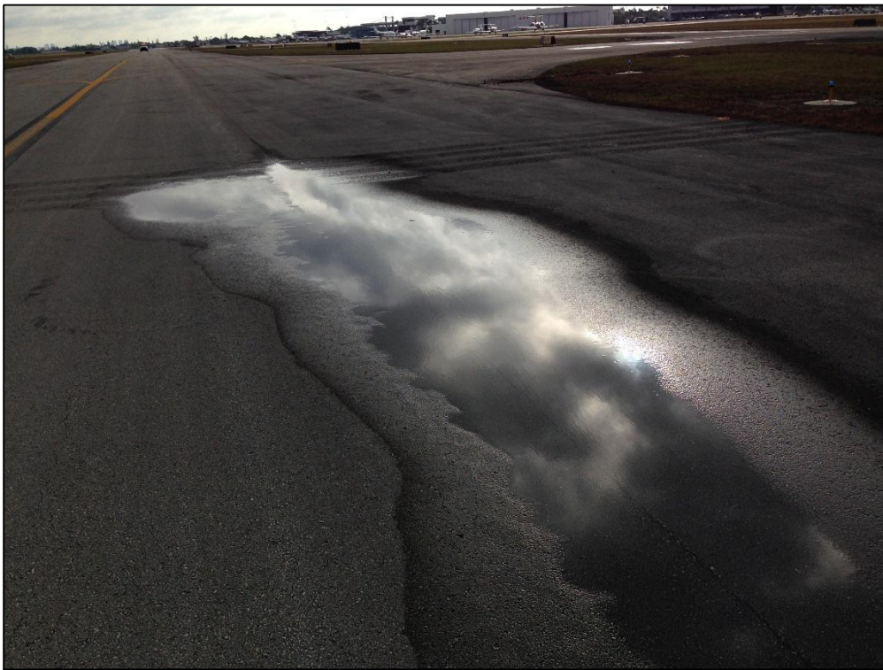
Taxiway November, Section 1422, Sample Unit 168 – Low Severity (52) Raveling, Medium Severity (53) Rutting, Medium Severity (57) Weathering
