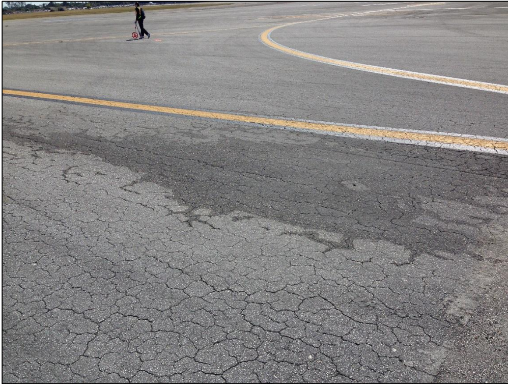
Taxiway Papa, Section 1660, Sample Unit 358 – Medium Severity (41) Alligator Cracking, Medium Severity (43) Block Cracking, Low Severity (52) Raveling, Low Severity (53) Rutting
