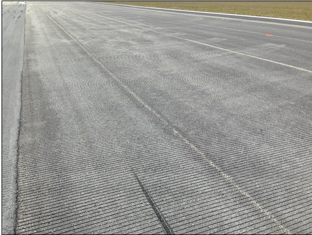
Runway 12-30, Section 6205, Sample Unit 326 – Low and Medium Severity (48) Longitudinal and Transverse Cracking, Low Severity (50) Patching, Low Severity (52) Raveling, Medium Severity (57) Weathering
