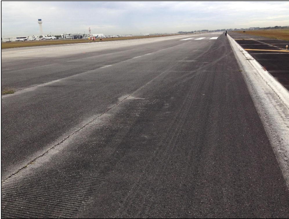
Runway 9L-27R, Section 6130, Sample Unit 176 – Low Severity (47) Joint Reflection Cracking, Medium Severity (47) Joint Reflection Cracking, Low Severity (52) Raveling, Low Severity (57) Weathering
