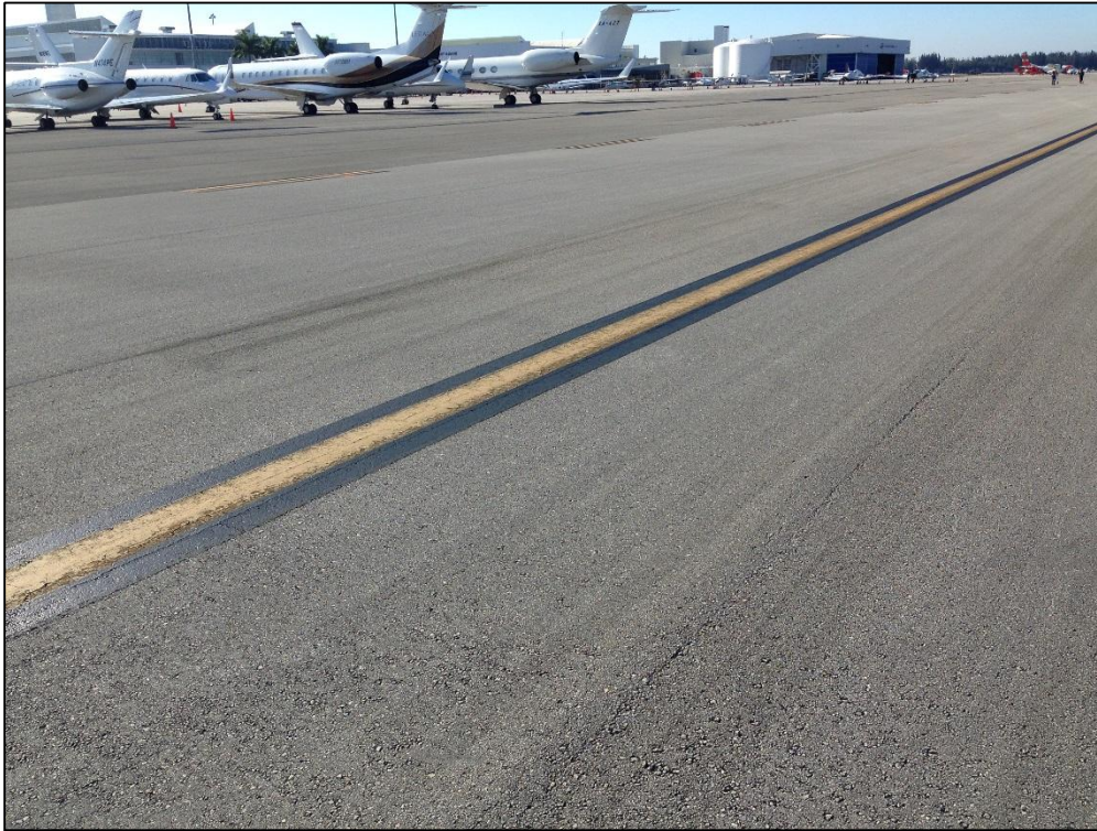
Taxiway Echo, Section 515, Sample Unit 519 – Low Severity (52) Raveling, Low Severity (53) Rutting, Low Severity (57) Weathering
