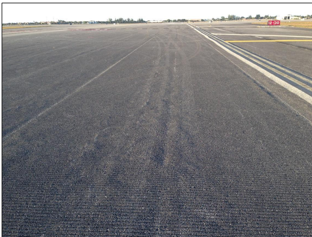
Taxiway Hotel, Section 6326, Sample Unit 532 – Low Severity (48) Longitudinal and Transverse Cracking, Low Severity (52) Raveling, Low Severity (56) Swelling
