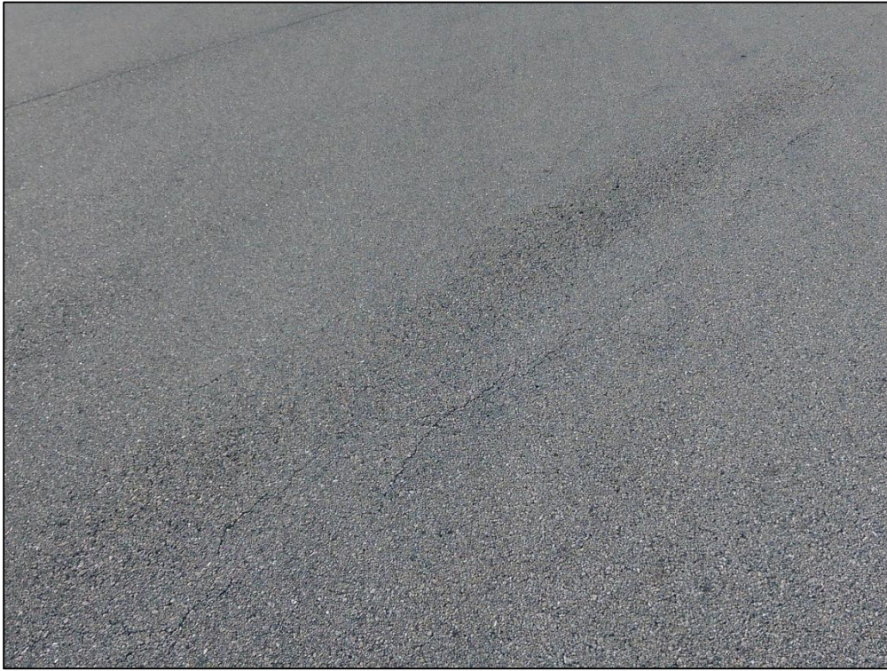
Taxiway G2, Section 530, Sample Unit 456 – Low Severity (41) Alligator Cracking, Low Severity (52) Raveling, Low Severity (57) Weathering
