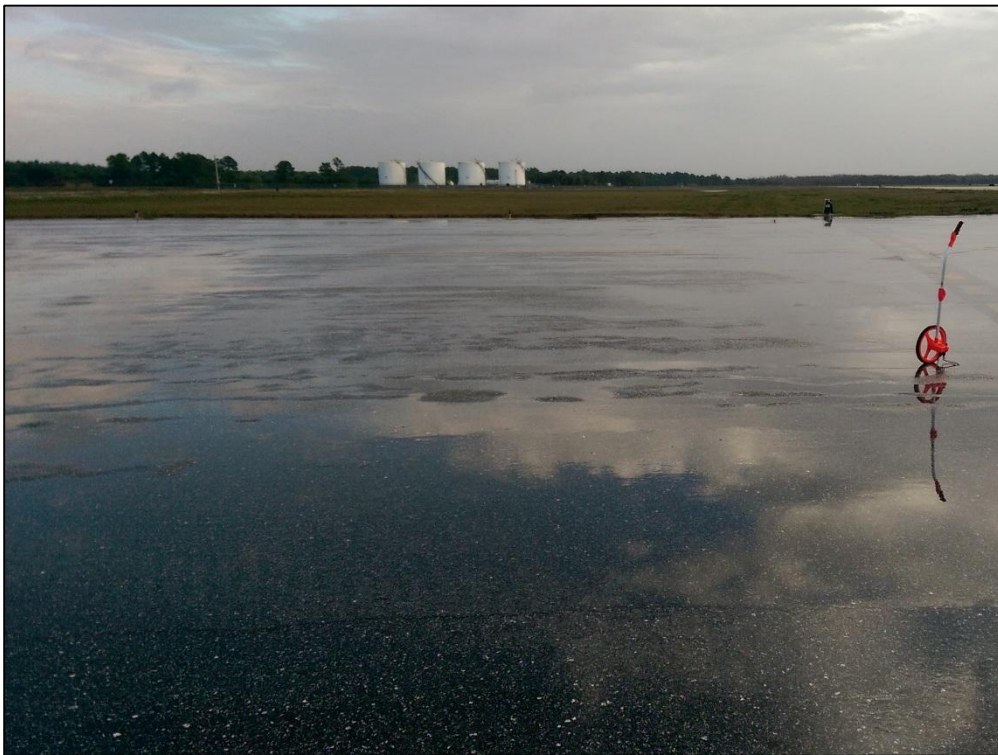
Taxiway A8, Section 825, Sample Unit 800 – Low Severity (48) Longitudinal and Transverse Cracking, Low Severity (45) Depression, Low Severity (56) Swelling, Low Severity (57) Weathering
