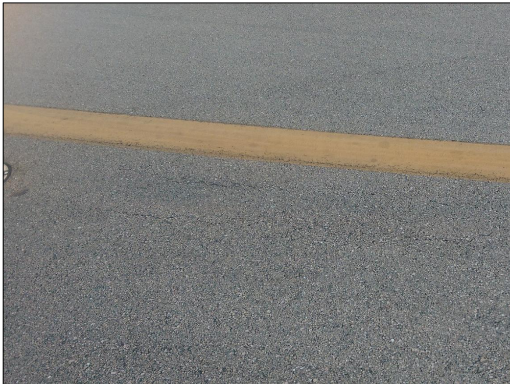
Taxiway F7, Section 750, Sample Unit 707 – Low Severity (53) Rutting, Low Severity (57) Weathering
