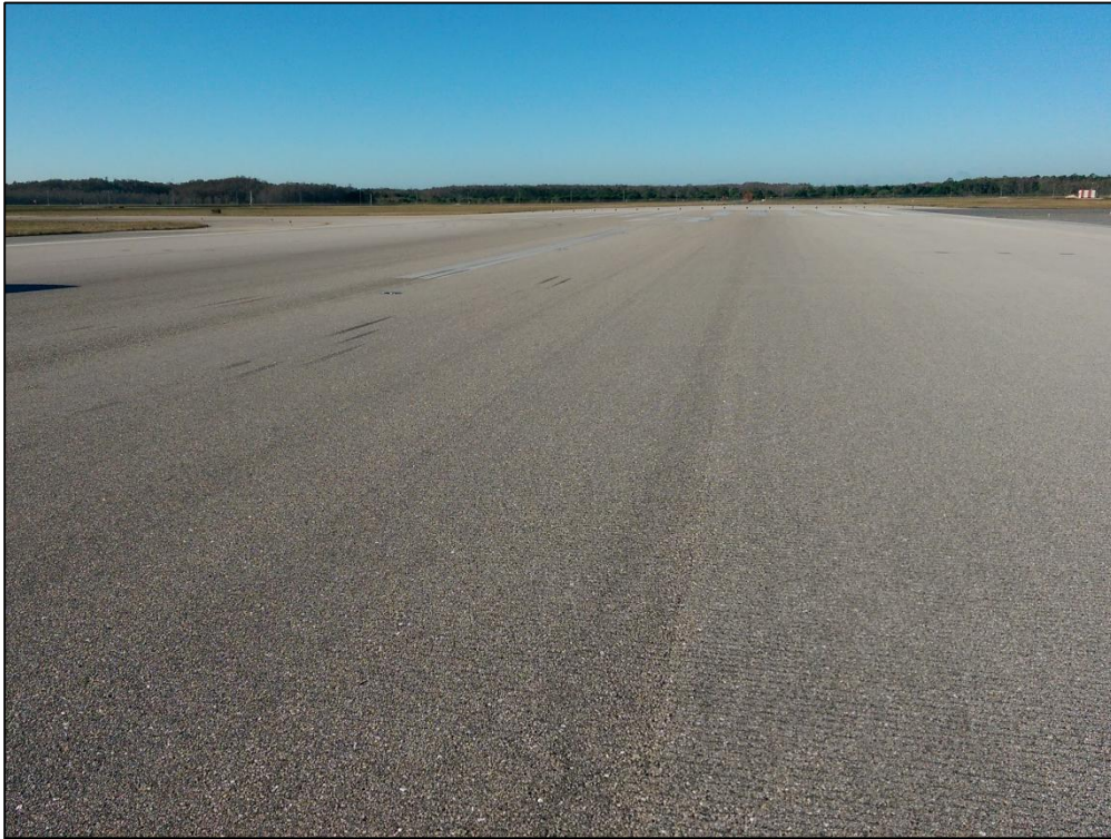
Runway 6-34, Section 6104, Sample Unit 484 – Low Severity (48) Longitudinal and Transverse Cracking, Low Severity (53) Rutting, Low Severity (57) Weathering
