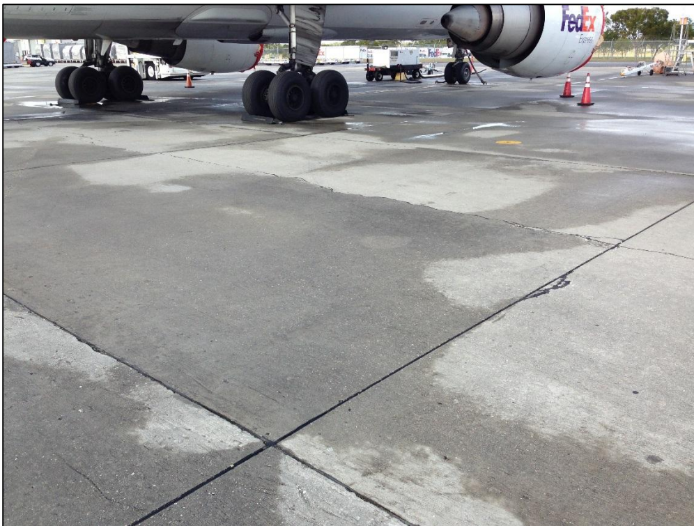
Apron Cargo, Section 4110, Sample Unit 153 – Low Severity (63) Longitudinal, Transverse, and Diagonal Cracking
