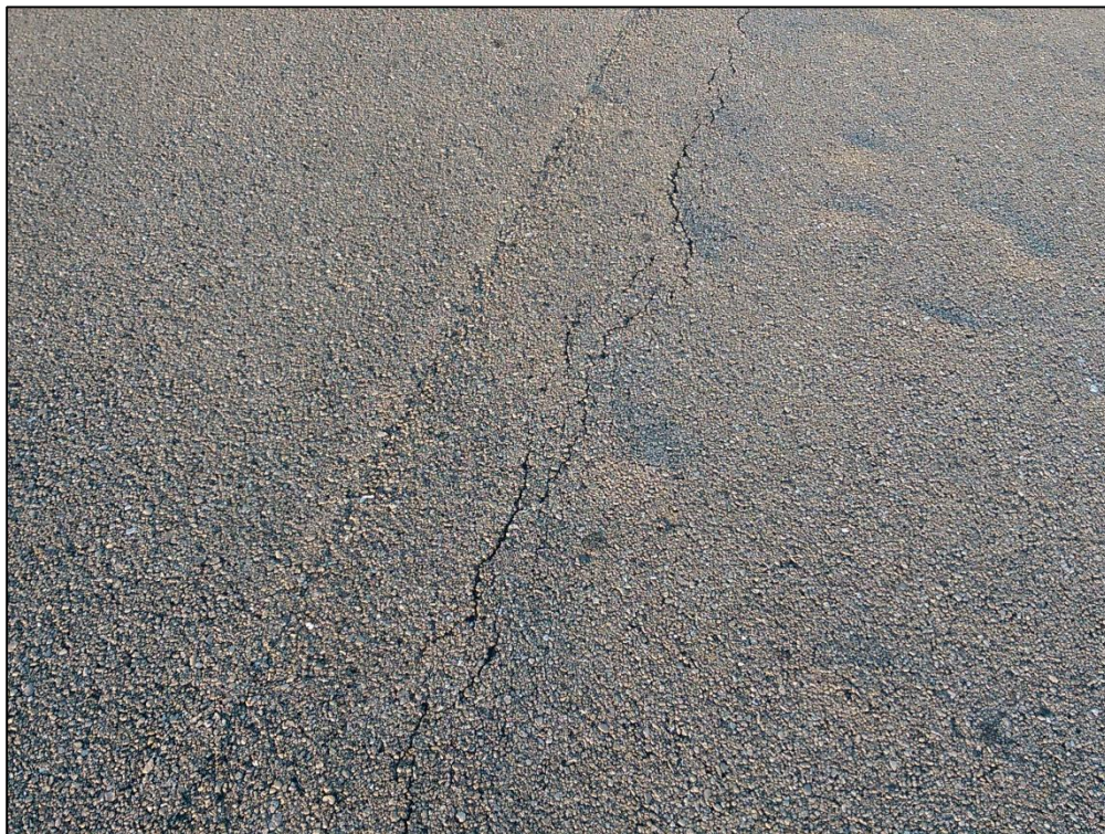
Taxiway Foxtrot, Section 260, Sample Unit 258 – Low Severity (41) Alligator Cracking, Low Severity (48) Longitudinal and Transverse Cracking, Low Severity (52) Raveling, Low Severity (56) Swelling, Low Severity (57) Weathering
