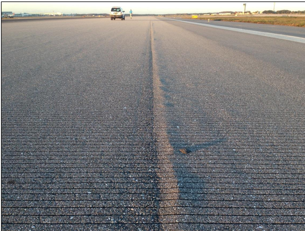
Runway 6-34, Section 6110, Sample Unit 428 – Low Severity (48) Longitudinal and Transverse Cracking, Low Severity (56) Swelling, Low Severity (57) Weathering
