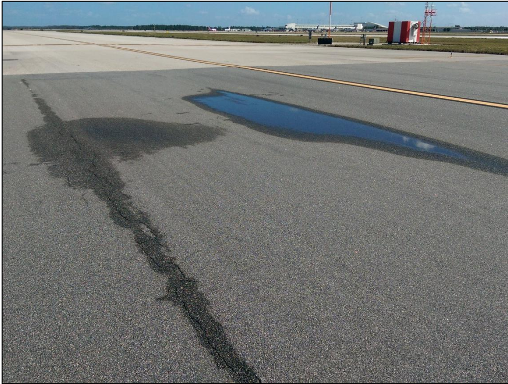
Taxiway Alpha, Section 109, Sample Unit 78 – Low Severity (41) Alligator Cracking, Low Severity (53) Rutting, Low Severity (52) Raveling, Low Severity (57) Weathering
