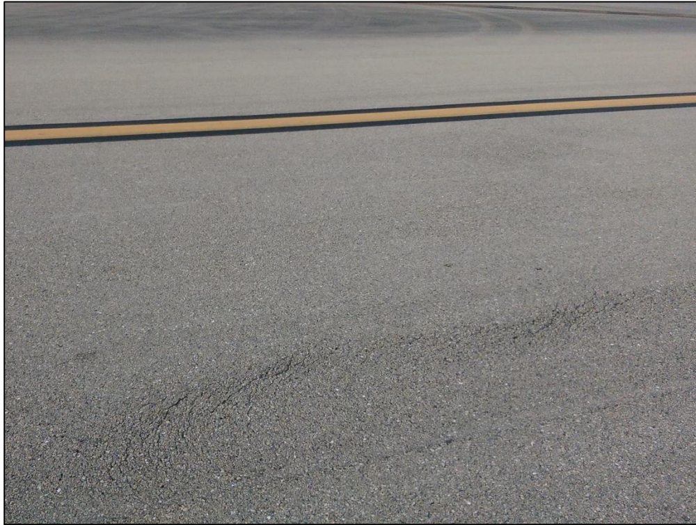
Taxiway Foxtrot, Section 260, Sample Unit 306 – (55) Slippage Cracking, Low Severity (57) Weathering
