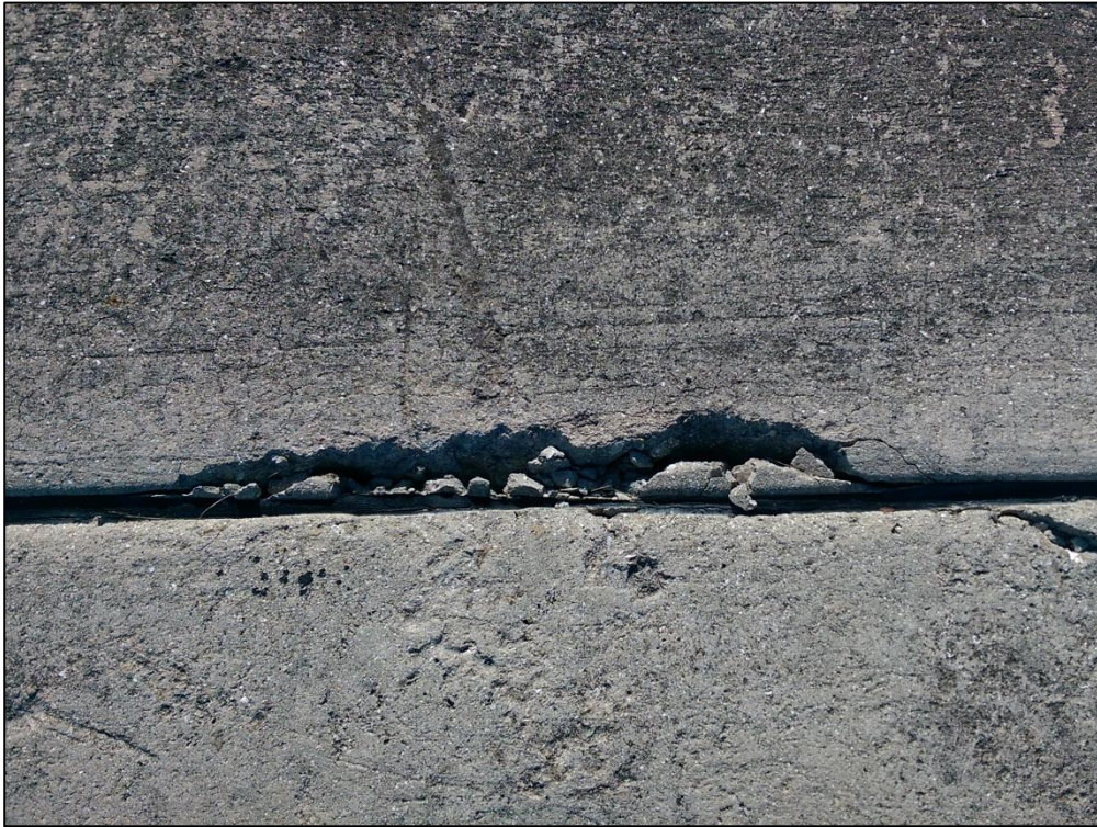
Apron North, Section 4320, Sample Unit 211 – Medium Severity (74) Joint Spalling
