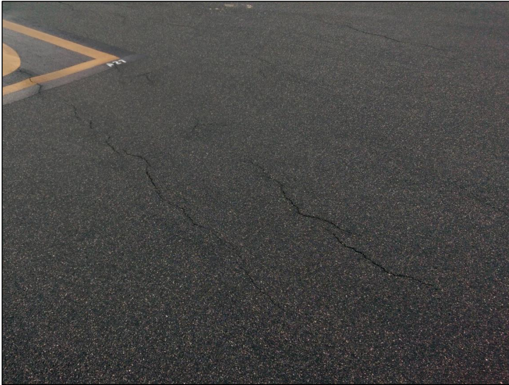
Taxiway A10, Section 107, Sample Unit 954 – Low Severity (48) Longitudinal and Transverse Cracking, Low Severity (56) Swelling, Low Severity (57) Weathering
