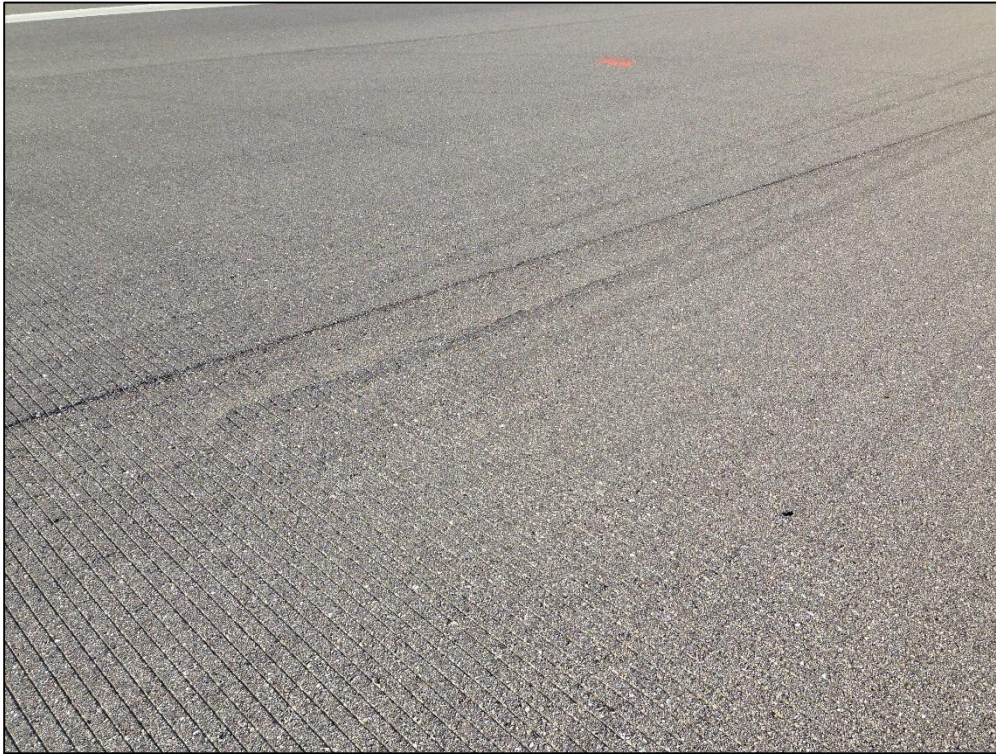
Runway 6-34, Section 6105, Sample Unit 538 – Low Severity (48) Longitudinal and Transverse Cracking, Low Severity (56) Swelling, Low Severity (57) Weathering
