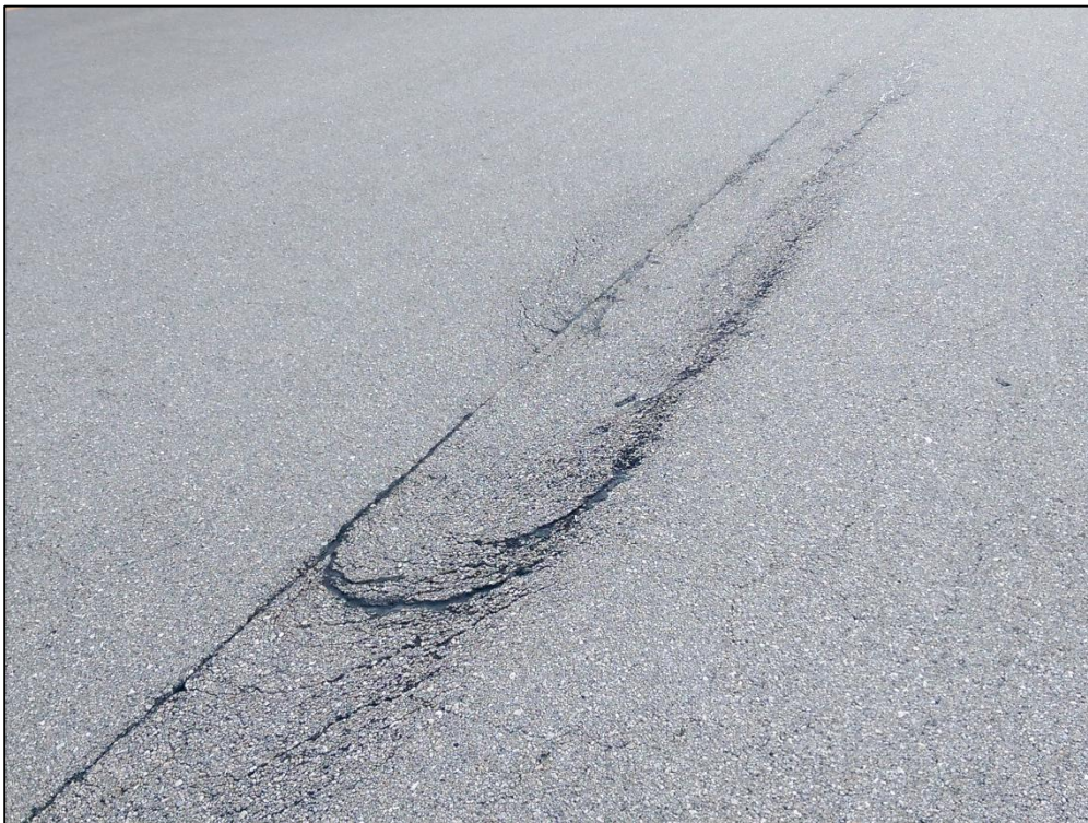
Taxiway Foxtrot, Section 250, Sample Unit 115 – (55) Slippage Cracking, Low Severity (57) Weathering
