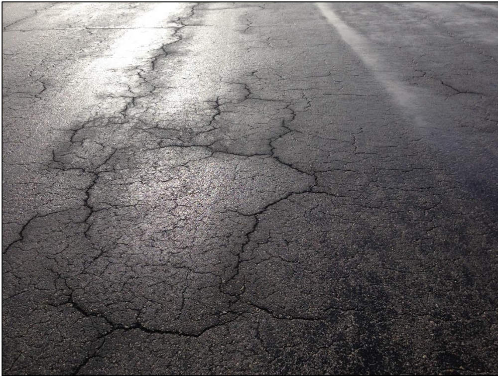
Apron FBO, Section 4205, Sample Unit 154 – Low Severity (43) Block Cracking, Low Severity (52) Raveling
