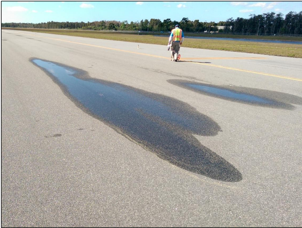
Taxiway Alpha, Section 109, Sample Unit 76 – Low Severity (52) Raveling, Low Severity (53) Rutting, Low Severity (57) Weathering
