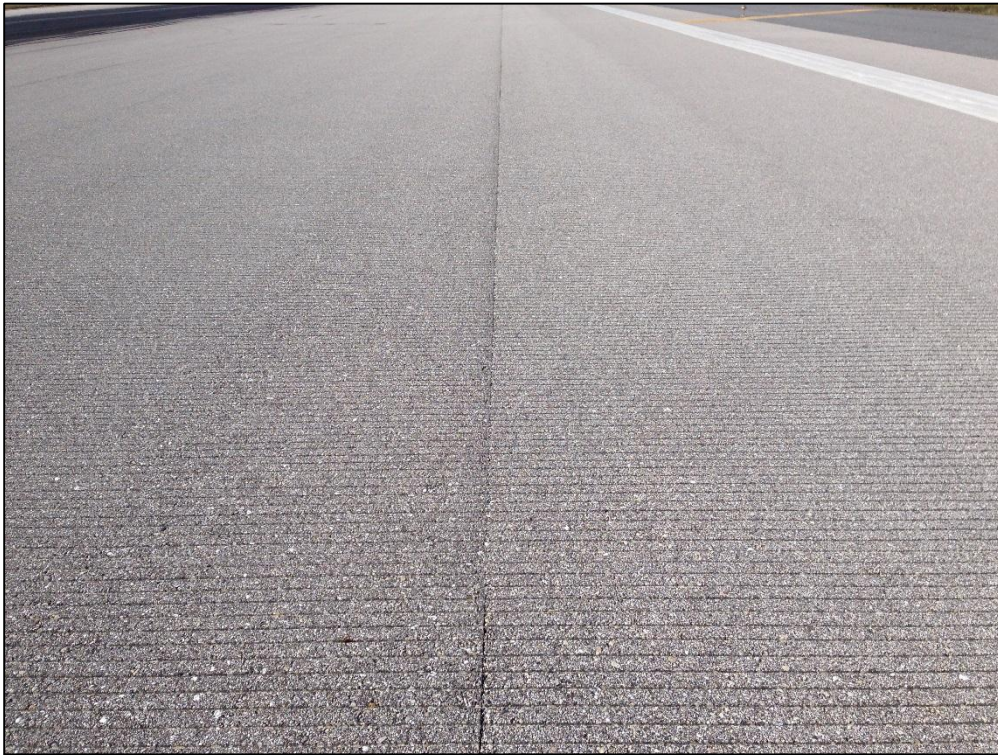
Runway 6-34, Section 6104, Sample Unit 294 – Low Severity (48) Longitudinal and Transverse Cracking, Low Severity (57) Weathering
