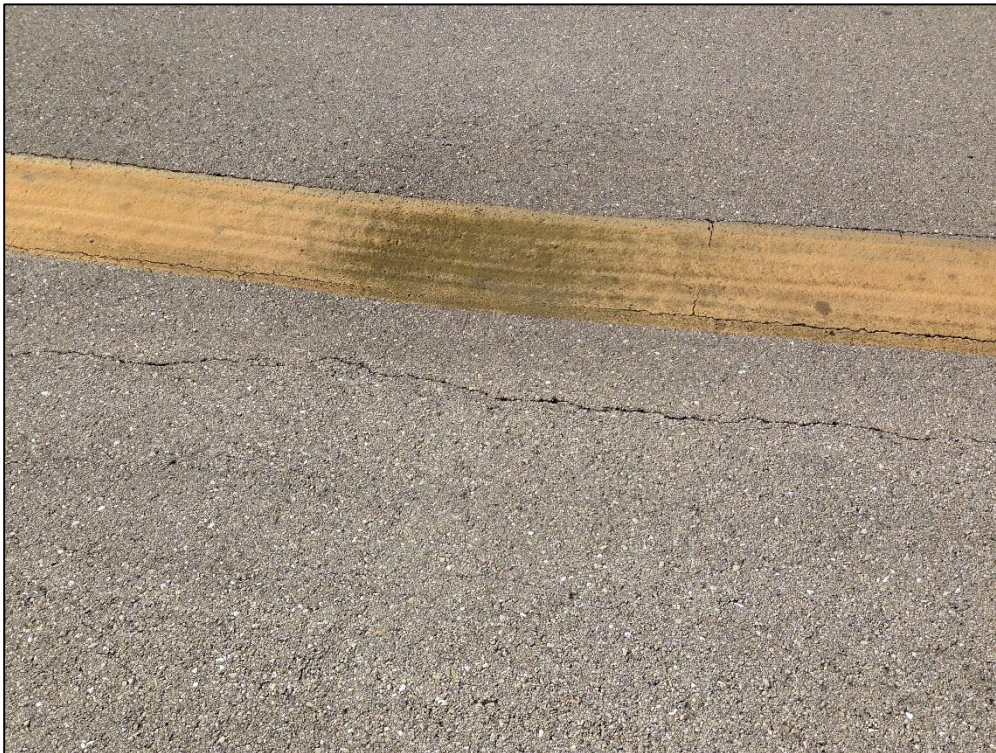
Apron South, Section 4425, Sample Unit 117 – Medium Severity (45) Depression, Low Severity (48) Longitudinal and Transverse Cracking, Medium Severity (57) Weathering
