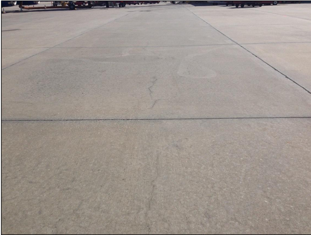
Apron South, Section 4410, Sample Unit 408 – (73) Shrinkage Cracks
