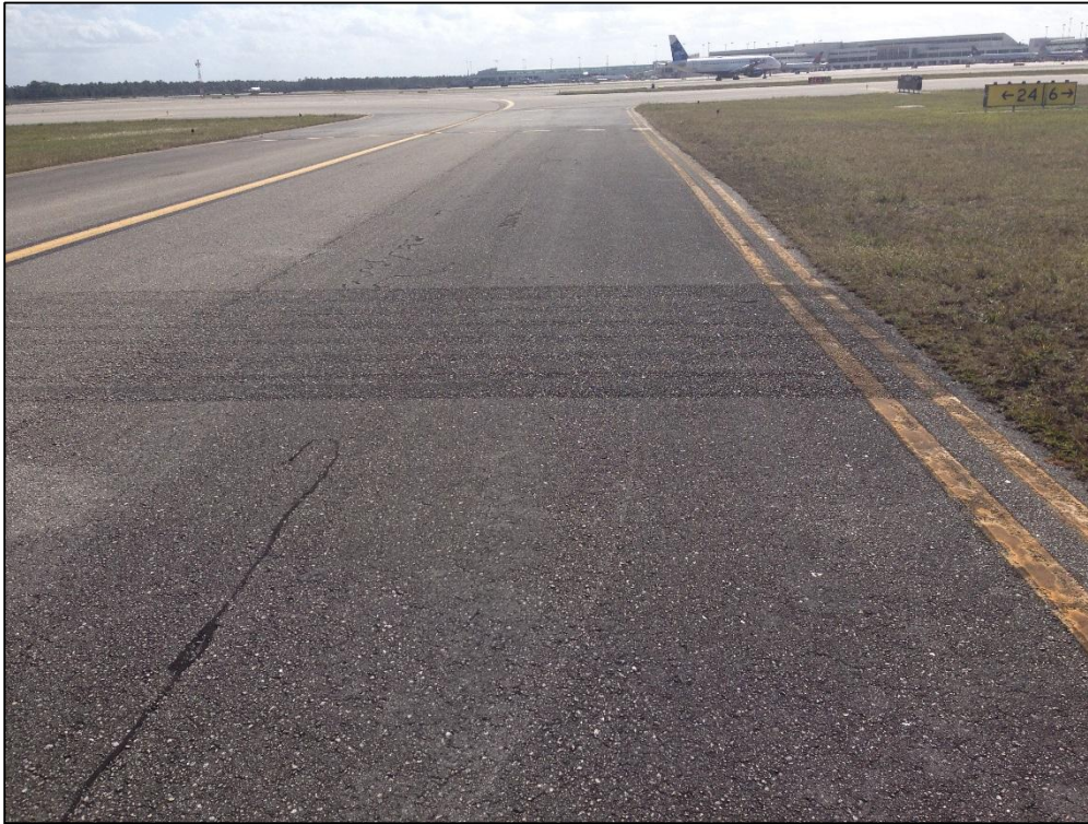
Taxiway A5, Section 555, Sample Unit 502 – Low Severity (48) Longitudinal and Transverse Cracking, Low Severity (52) Raveling, Medium Severity (57) Weathering
