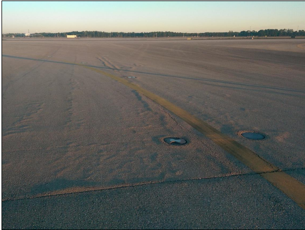
Taxiway F7, Section 750, Sample Unit 702 – Low and Medium Severity (48) Longitudinal and Transverse Cracking, Low Severity (56) Swelling, Low Severity (57) Weathering
