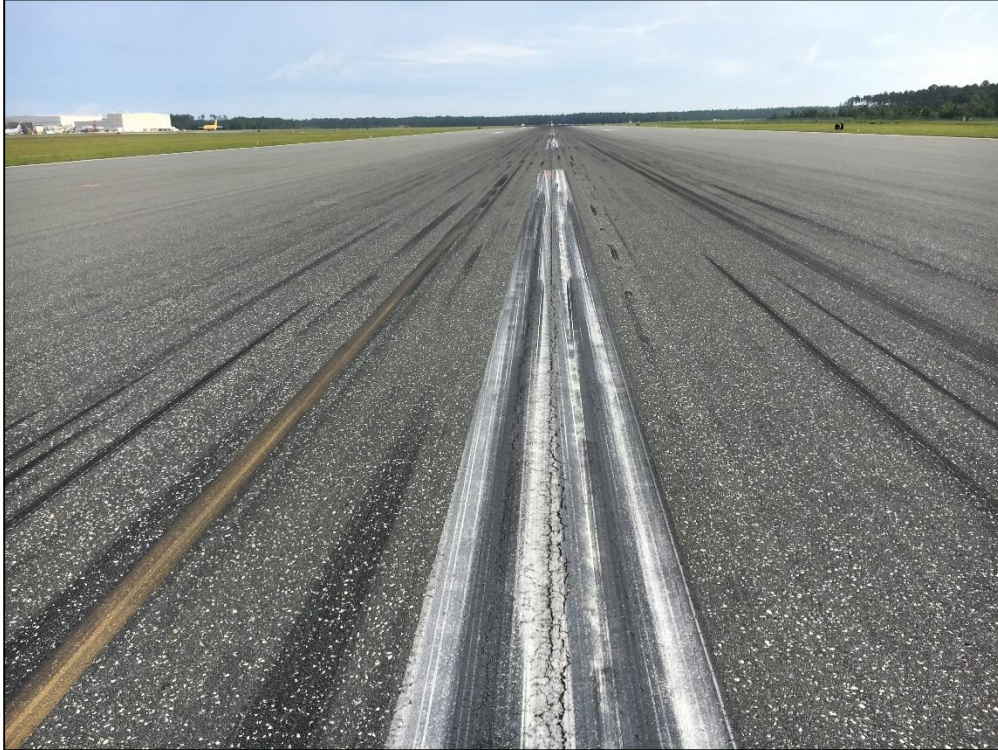
Runway 18L-36R, Section 6215, Sample Unit 538 - Low Severity (48) Longitudinal and Transverse Cracking, Low Severity (57) Weathering
