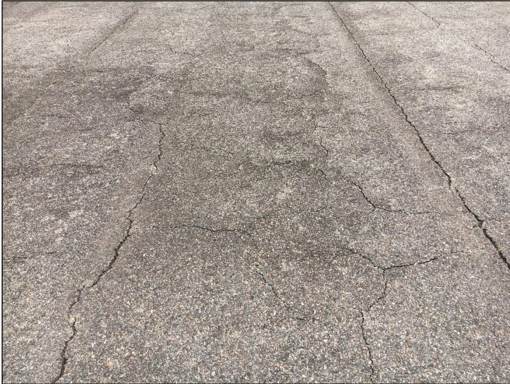
Runway 18R-36L, Section 6120, Sample Unit 169 - Medium Severity (43) Block Cracking, Medium Severity (52) Raveling, Low Severity (56) Swelling
