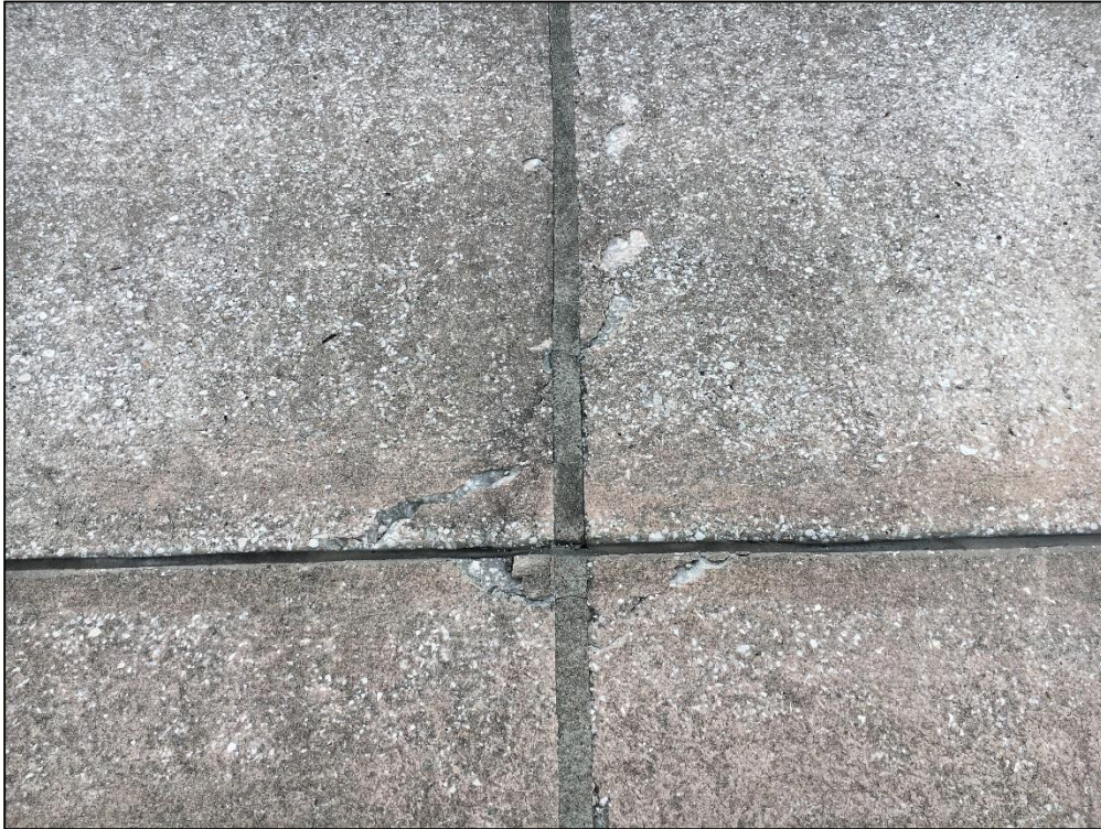
Taxiway D, Section 405, Sample Unit 468 - Low Severity (65) Joint Seal Damage, (73) Shrinkage Cracking, Low Severity (75) Corner Spall
