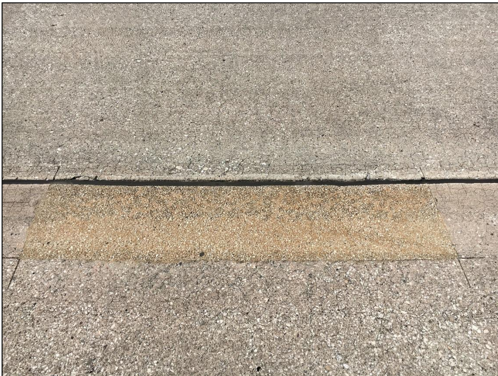
Runway 9R-27L, Section 6335, Sample Unit 382 - Low Severity (66) Small Patch, (73) Shrinkage Cracking
