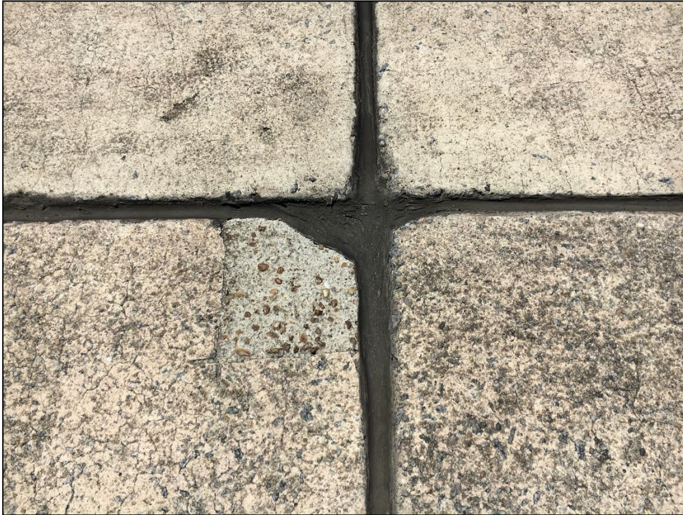
Taxiway B, Section 205, Sample Unit 177 - Medium Severity (66) Small Patch, (73) Shrinkage Cracking
