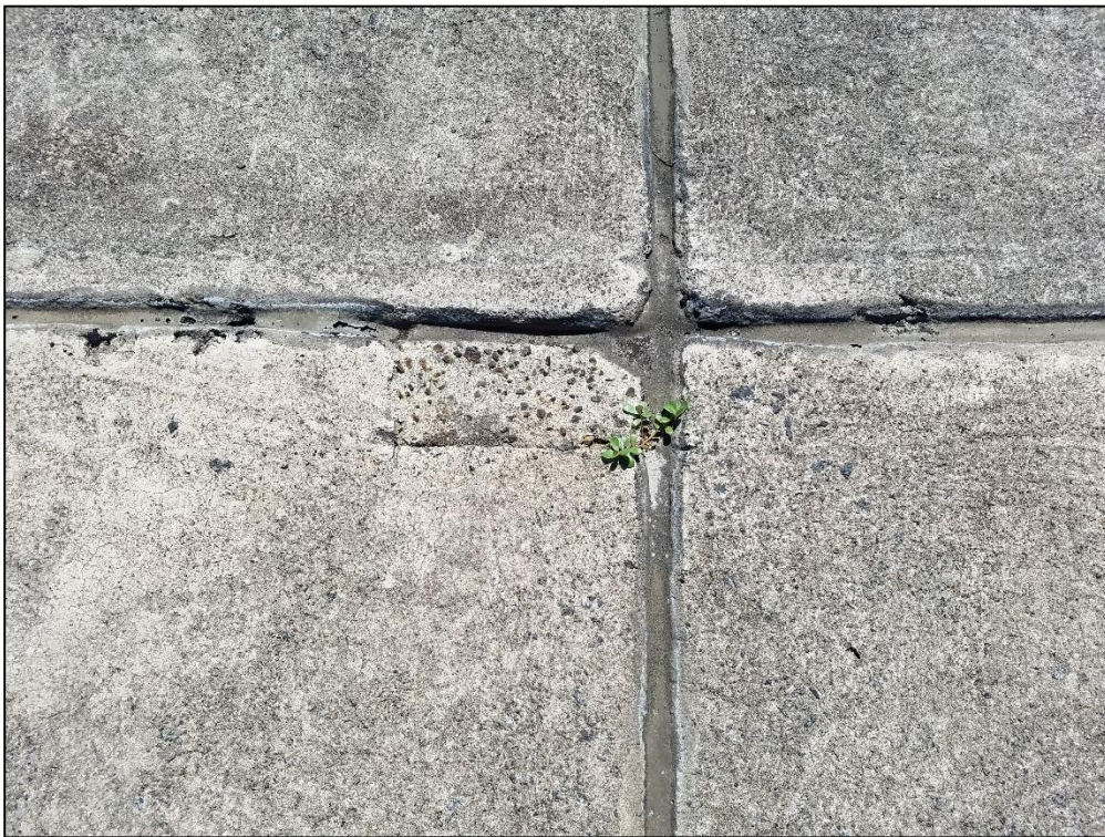
Taxiway C, Section 305, Sample Unit 117 - Low Severity (65) Joint Seal Damage, Medium Severity (66) Small Patch, (73) Shrinkage Cracking
