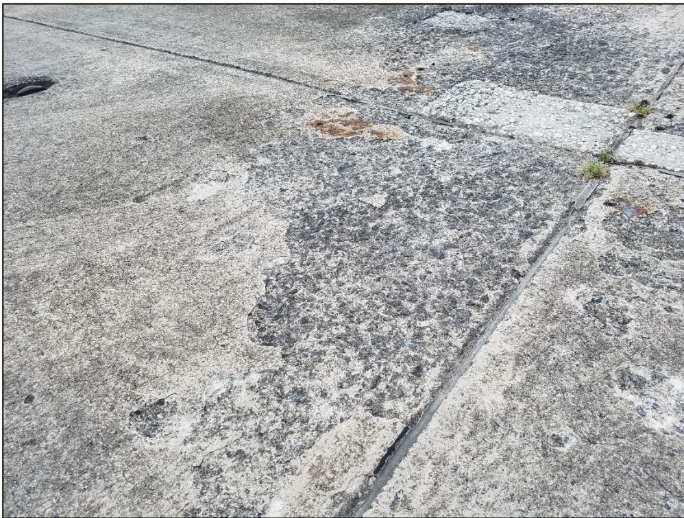
Apron N, Section 4125, Sample Unit 473 - Low Severity (65) Joint Seal Damage, Low Severity (66) Small Patch, Medium Severity (66) Small Patch, Medium Severity (70) Scaling
