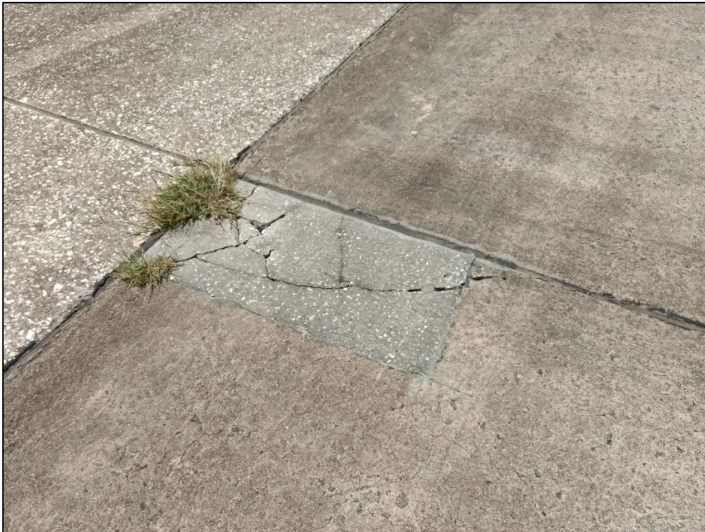
Apron W, Section 4270, Sample Unit 178 – Medium Severity (66) Small Patch, (73) Shrinkage Cracking
