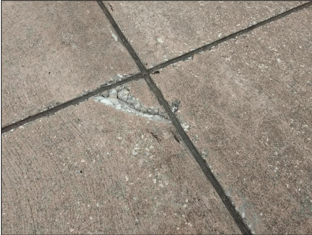
Taxiway A, Section 110, Sample Unit 266 - (73) Shrinkage Cracking, High Severity (75) Corner Spall
