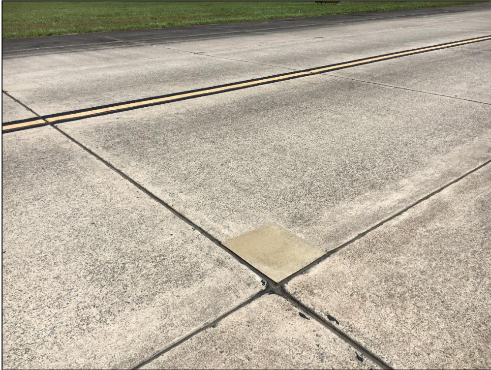
Taxiway A, Section 130, Sample Unit 131 - Low Severity (66) Small Patch, (73) Shrinkage Cracking
