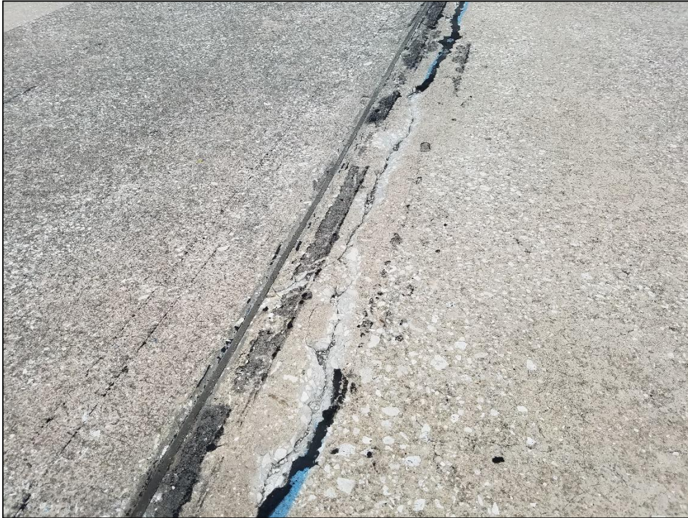
Apron N, Section 4120, Sample Unit 288 - Low Severity (65) Joint Seal Damage, Medium Severity (73) Joint Spall
