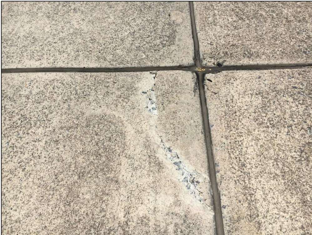
Taxiway A, Section 130, Sample Unit 158 - (73) Shrinkage Cracking, Medium Severity (75) Corner Spall
