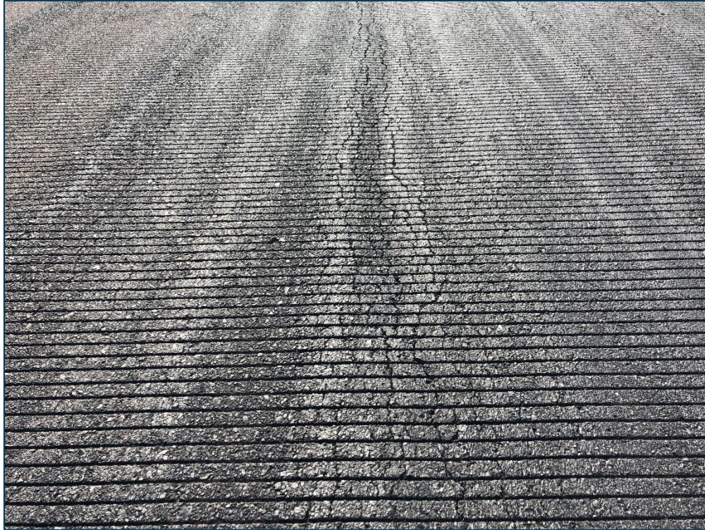
RW 18L-36R, Section 6185, Sample Unit 441 - Low Severity (41) Alligator Cracking and Low and Medium Severity (52) Raveling
