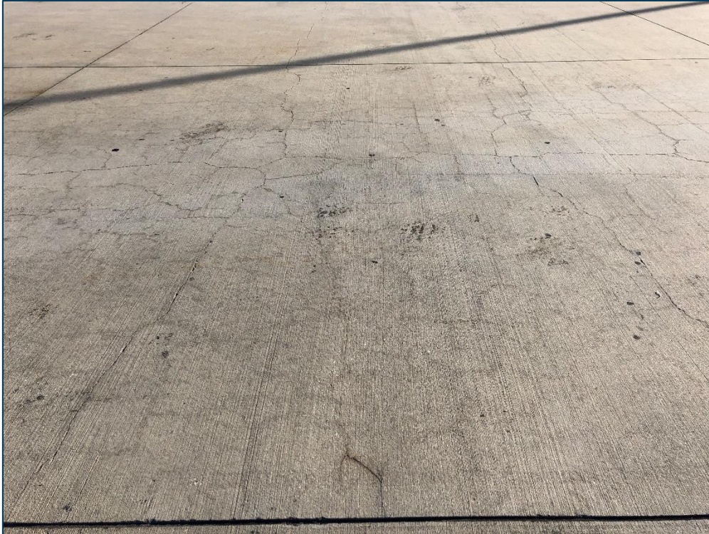
AP MAIN, Section 4198, Sample Unit 107 - Medium Severity (72) Shattered Slab
