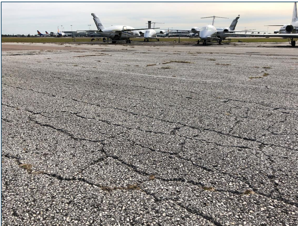
TWH, Section 810, Sample Unit 112 - Medium Severity (41) Alligator Cracking and Medium Severity (52) Raveling
