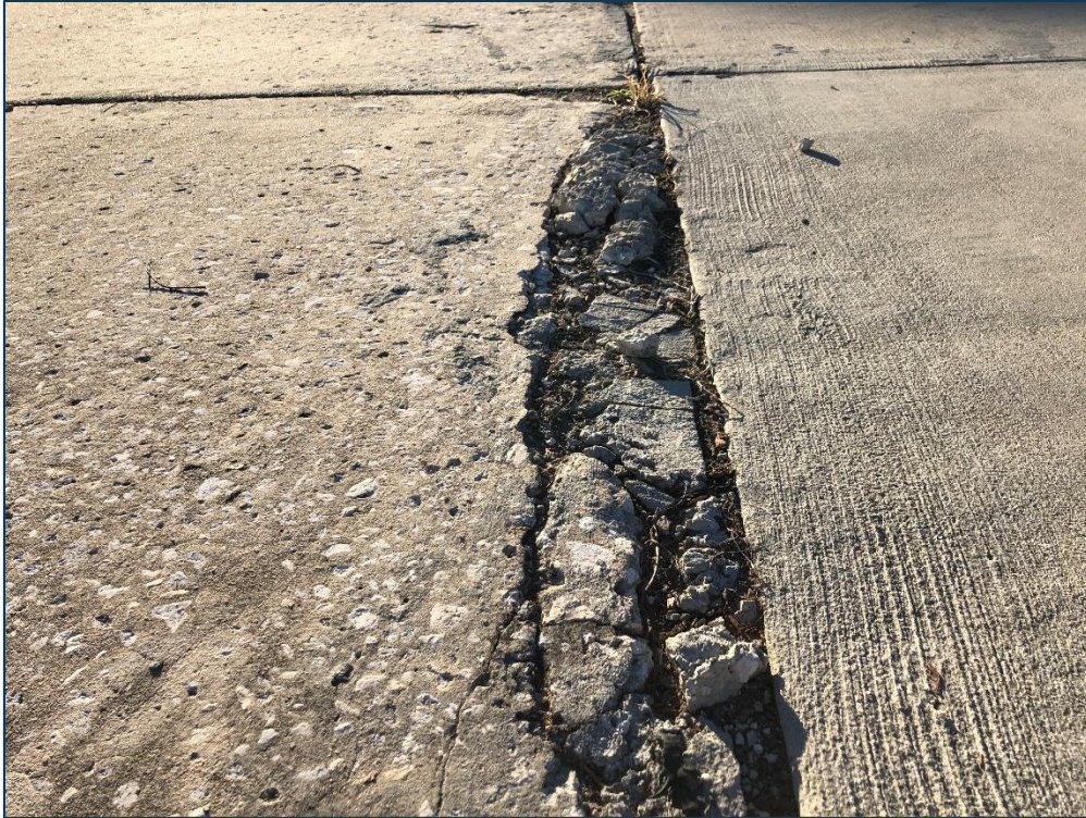
AP MAIN, Section 4175, Sample Unit 603 - High Severity (65) Joint Seal Damage and High Severity (74) Joint Spall
