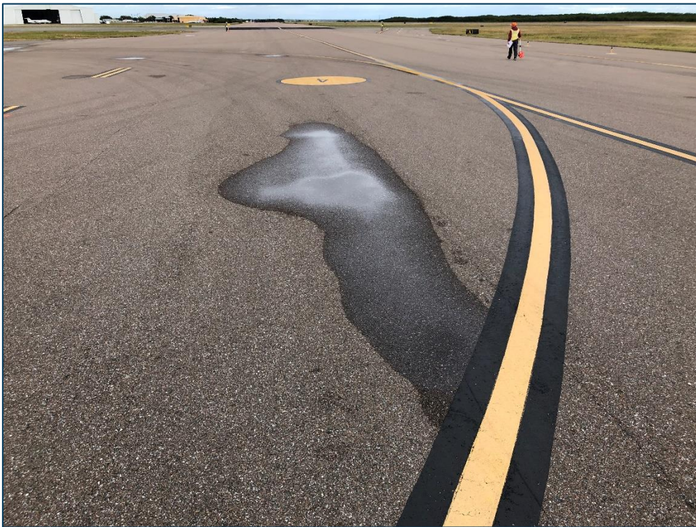
TWA, Section 115, Sample Unit 109 - Low Severity (48) Longitudinal & Transverse Cracking, Low Severity (53) Rutting, and Low Severity (57) Weathering
