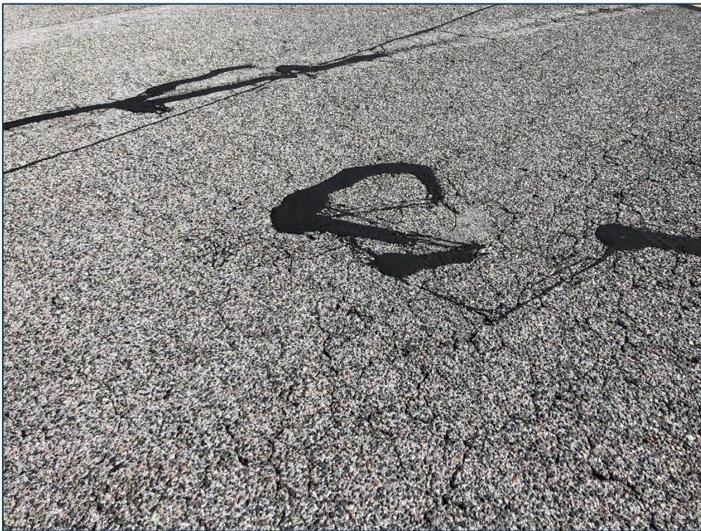
TW 9-27, Section 6345, Sample Unit 369 - Low Severity (41) Alligator Cracking and Low and Medium Severity (52) Raveling
