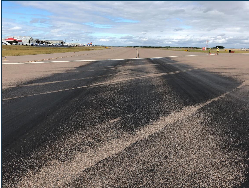
RW 4-22, Section 6225, Sample Unit 412 - (42) Bleeding and Low Severity (57) Weathering
