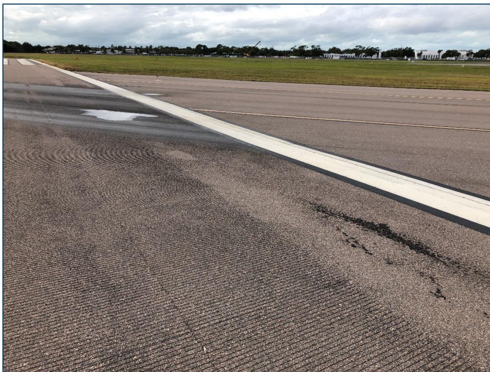
RW 4-22, Section 6230, Sample Unit 210 - (42) Bleeding, Low Severity (48) Longitudinal & Transverse Cracking, Low Severity (52) Raveling, Medium Severity (53) Rutting, and Low Severity (57) Weathering
