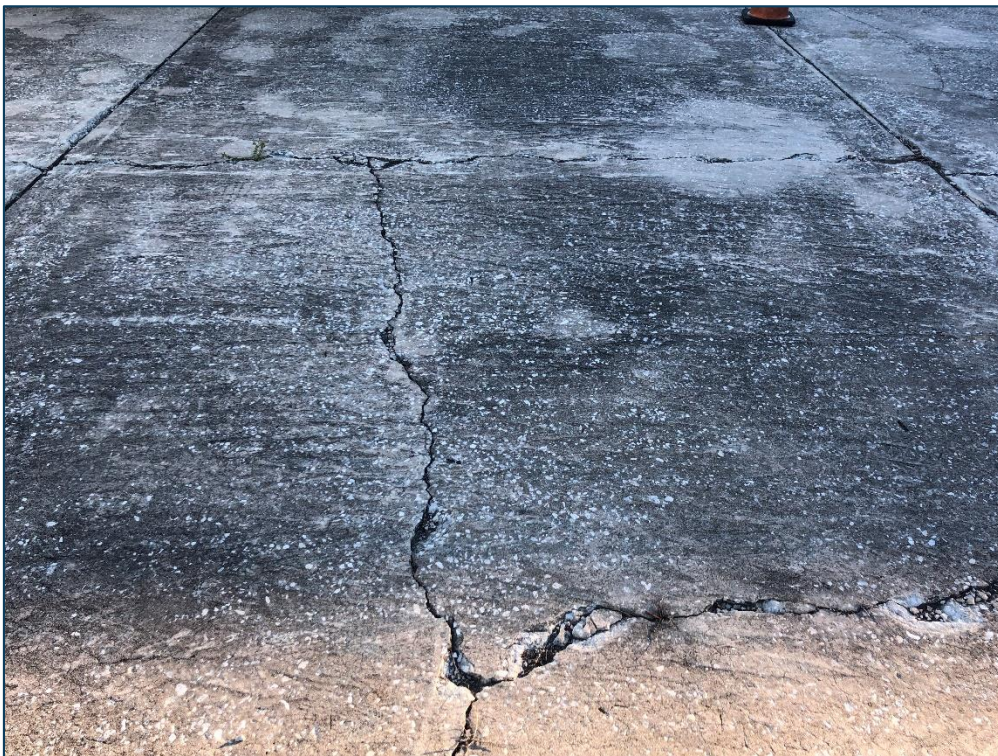
AP MAIN, Section 4175, Sample Unit 603 - High Severity (65) Joint Seal Damage and Medium Severity (72) Shattered Slab
