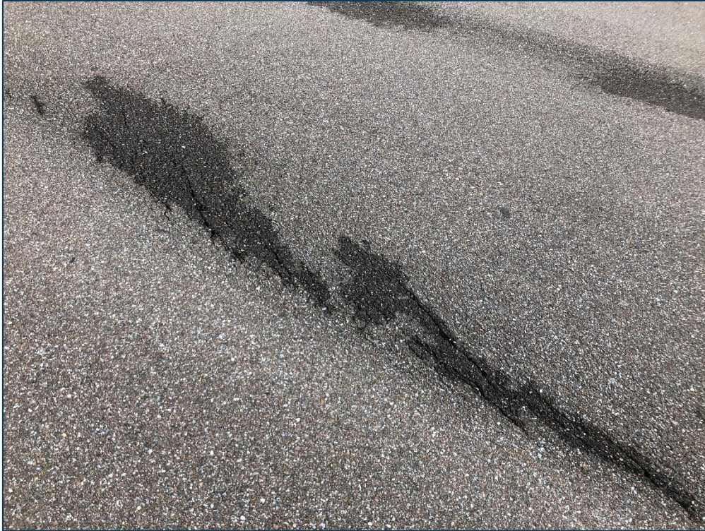
TWA, Section 115, Sample Unit 149 - (55) Slippage Cracking and Low Severity (57) Weathering
