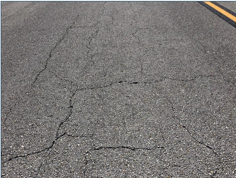
TW N, Section 1408, Sample Unit 208 - Low Severity (43) Block Cracking and Low Severity (52) Raveling
