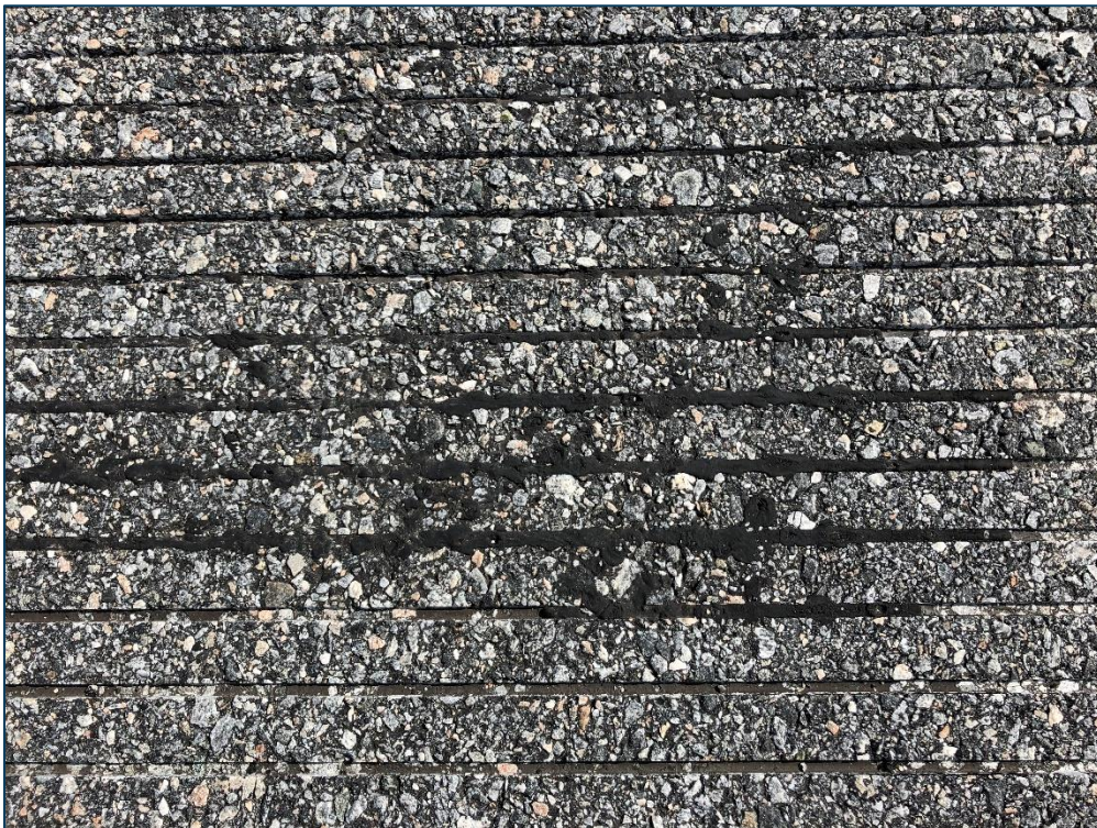
RW 7L-25R, Section 6160, Sample Unit 408 - (42) Bleeding, Low Severity (57) Weathering, and Medium Severity (57) Weathering
