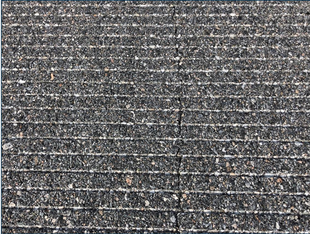
RW 7L-25R, Section 6130, Sample Unit 390 - Low Severity (48) Longitudinal & Transverse Cracking, Low Severity (57) Weathering, and Medium Severity (57) Weathering
