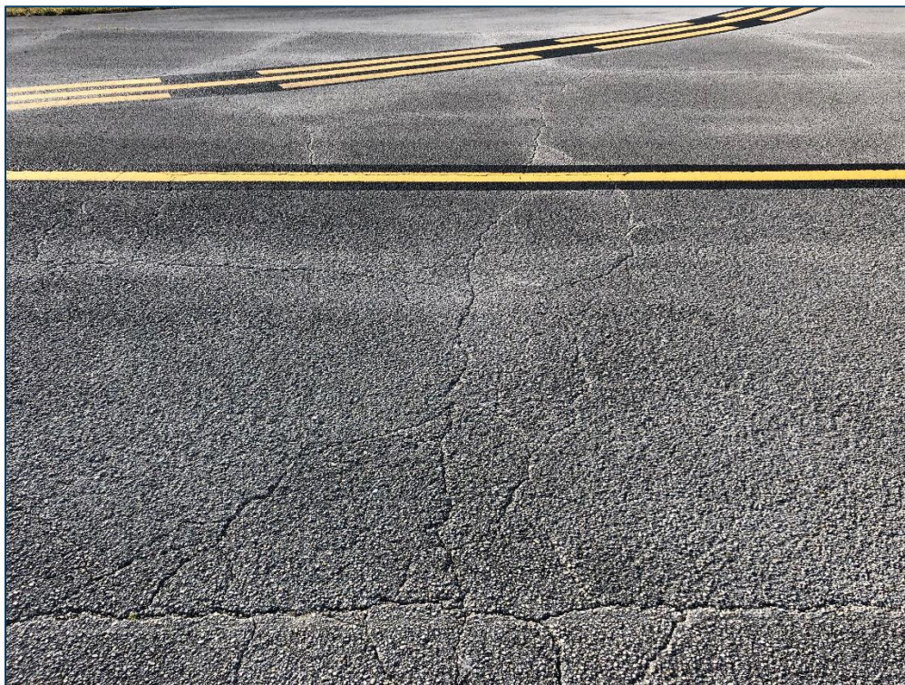
TW S, Section 1905, Sample Unit 114 - Low Severity (41) Alligator Cracking, Low Severity (52) Raveling, and Medium Severity (52) Raveling
