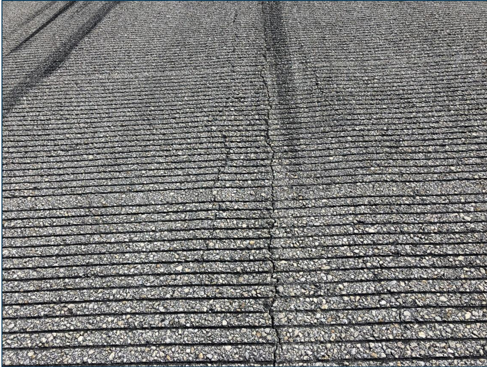
RW 16-34, Section 6215, Sample Unit 374 - Low Severity (48) Longitudinal & Transverse Cracking, Low Severity (52) Raveling, and Low Severity (56) Swelling
