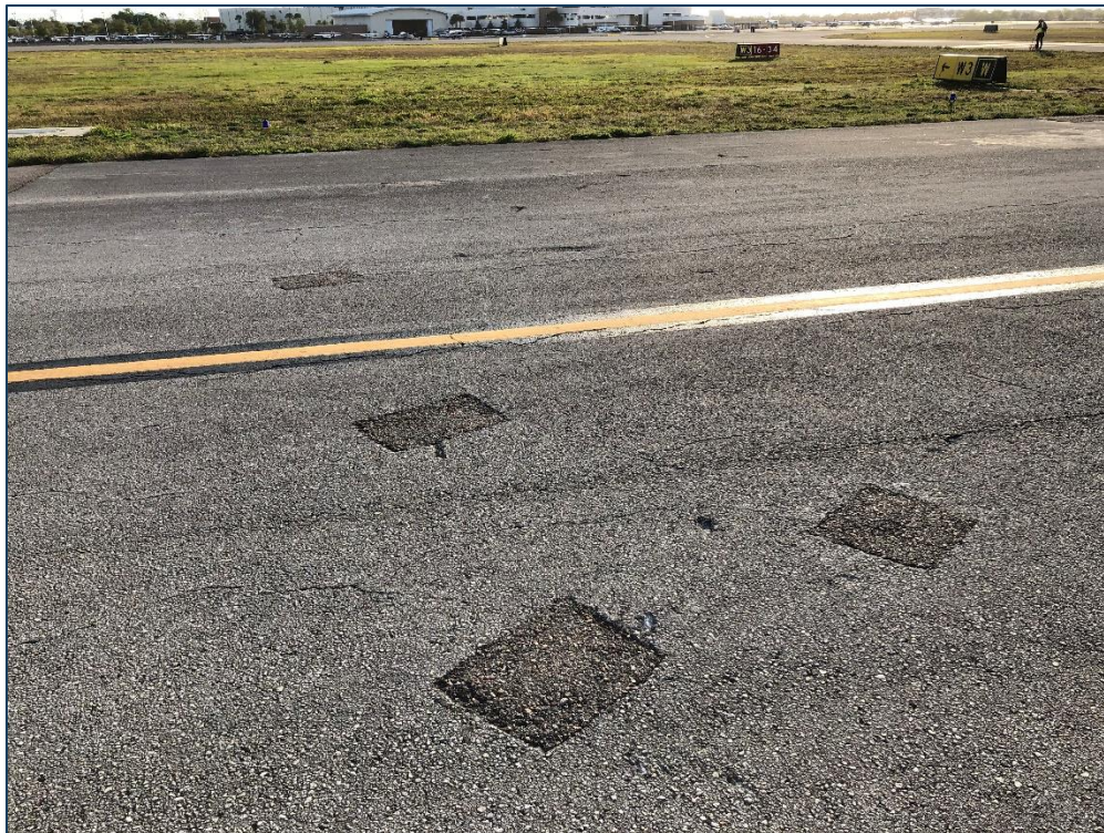
TW W, Section 2340, Sample Unit 309 - Low Severity (48) Longitudinal & Transverse Cracking, Low Severity (50) Patching, Low Severity (52) Raveling, and Medium Severity (57) Weathering
