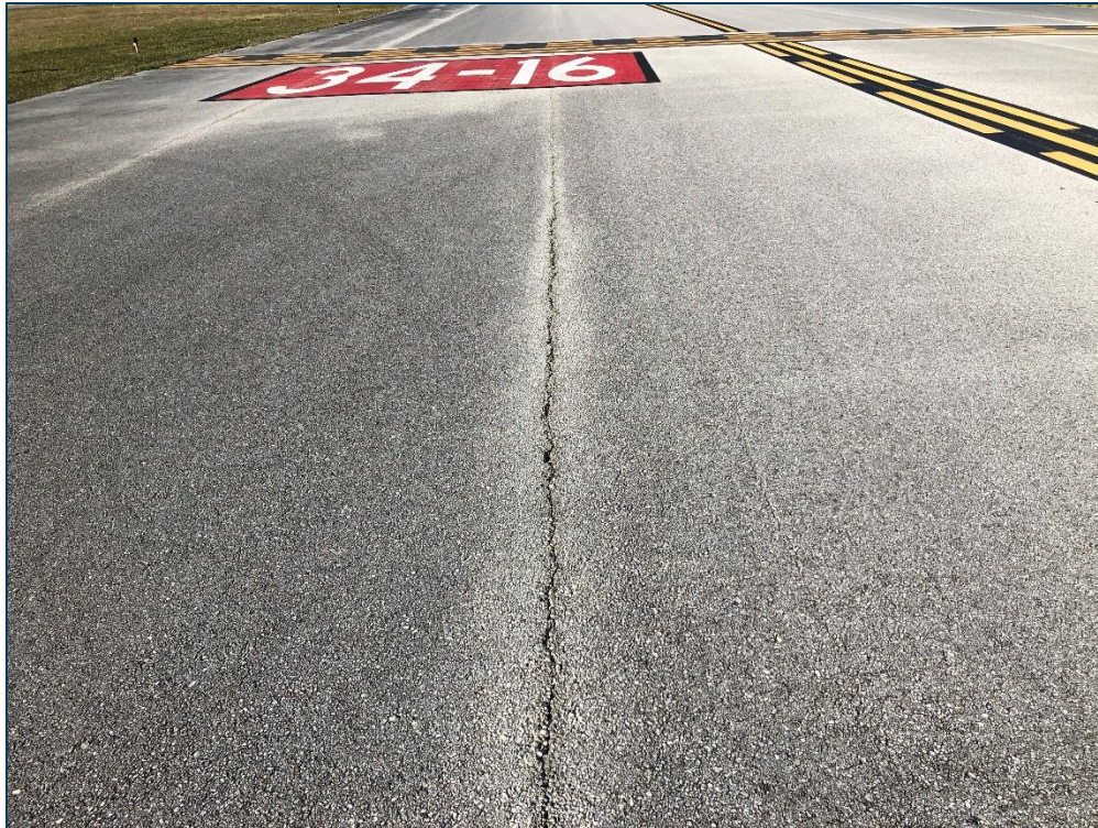
TW P, Section 835, Sample Unit 505 - Low Severity (48) Longitudinal & Transverse Cracking, Medium Severity (48) Longitudinal & Transverse Cracking, Low Severity (52) Raveling, and Low Severity (57) Weathering
