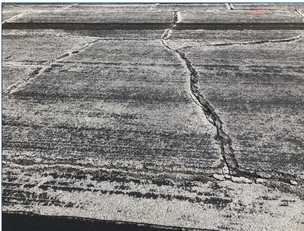
AP NE, Section 4215, Sample Unit 162 - Medium Severity (43) Block Cracking, High Severity (43) Block Cracking, and Low Severity (52) Raveling
