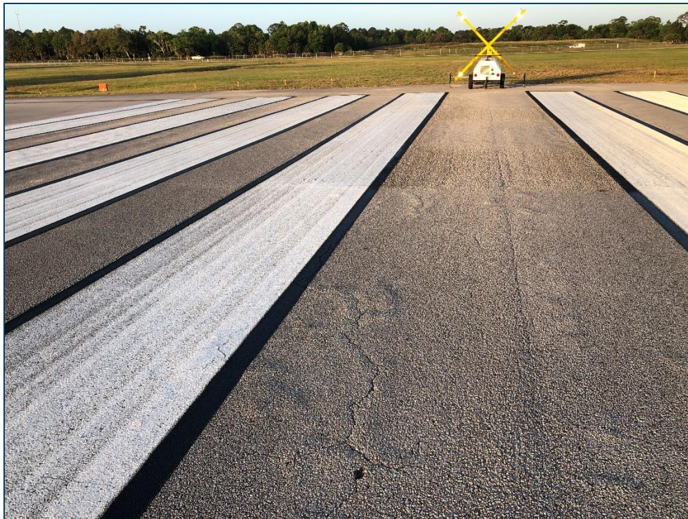
RW 7R-25L, Section 6305, Sample Unit 101 - Low Severity (48) Longitudinal & Transverse Cracking, Medium Severity (48) Longitudinal & Transverse Cracking, Low Severity (52) Raveling, Medium Severity (52) Raveling, and Low Severity (56) Swelling
