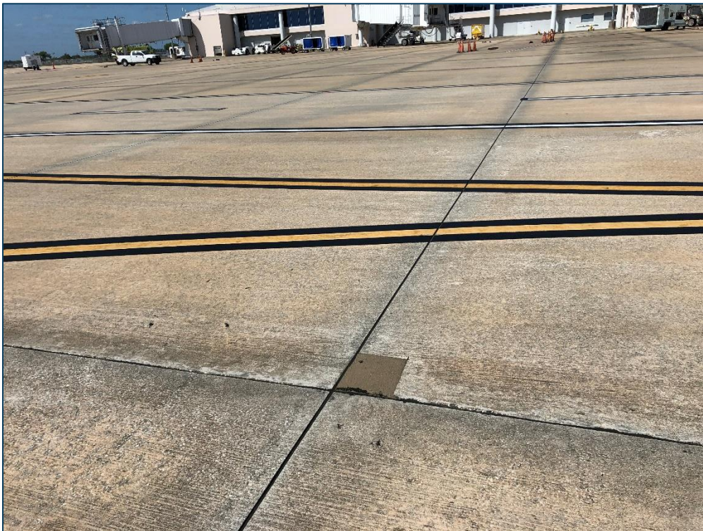
AP TERM, Section 4105, Sample Unit 707 - Low Severity (66) Small Patch
