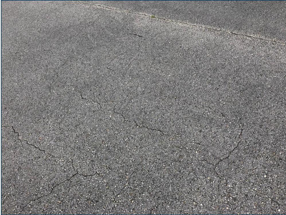
TW E, Section 560, Sample Unit 156 - Low Severity (48) Longitudinal & Transverse Cracking, Low Severity (52) Raveling, and Low Severity (57) Weathering
