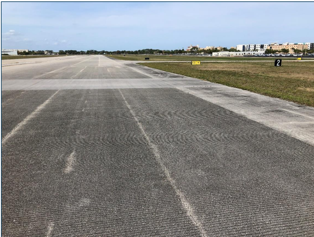
RW 16-34, Section 6220, Sample Unit 576 - Low Severity (48) Longitudinal & Transverse Cracking, Medium Severity (48) Longitudinal & Transverse Cracking, Low Severity (50) Patching, Low Severity (52) Raveling, and Low Severity (56) Swelling
