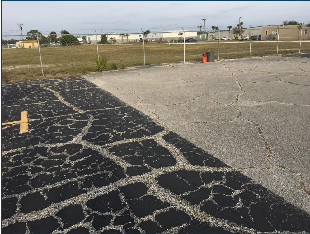
AP NOVA, Section 4305, Sample Unit 155 - Medium Severity (43) Block Cracking, Low Severity (52) Raveling, and High Severity (52) Raveling
