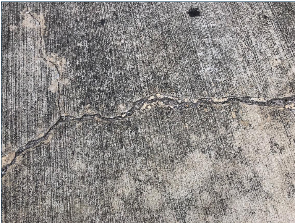
AP N TERM, Section 4140, Sample Unit 401 - Medium Severity (63) Linear Cracking and (73) Shrinkage Cracking
