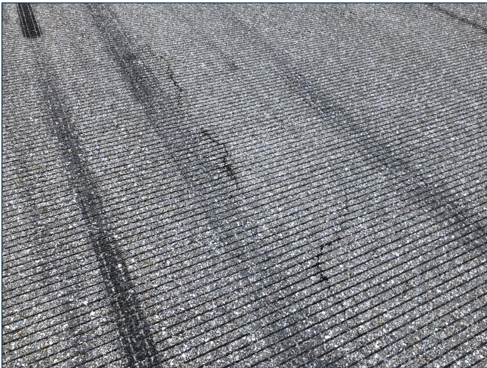
RW 14-32, Section 6305, Sample Unit 186 - Low Severity (48) Longitudinal & Transverse Cracking, Low Severity (52) Raveling, and Low Severity (57) Weathering
