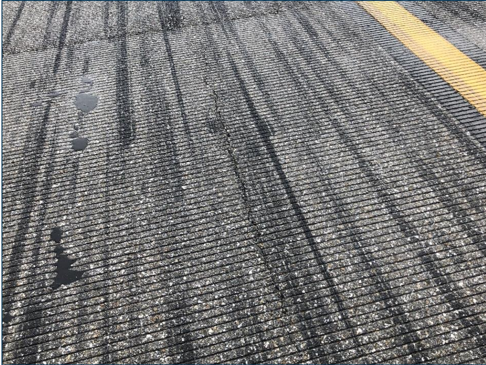
RW 14-32, Section 6305, Sample Unit 149 - (42) Bleeding, Low Severity (48) Longitudinal & Transverse Cracking, Low Severity (52) Raveling, and Low Severity (57) Weathering
