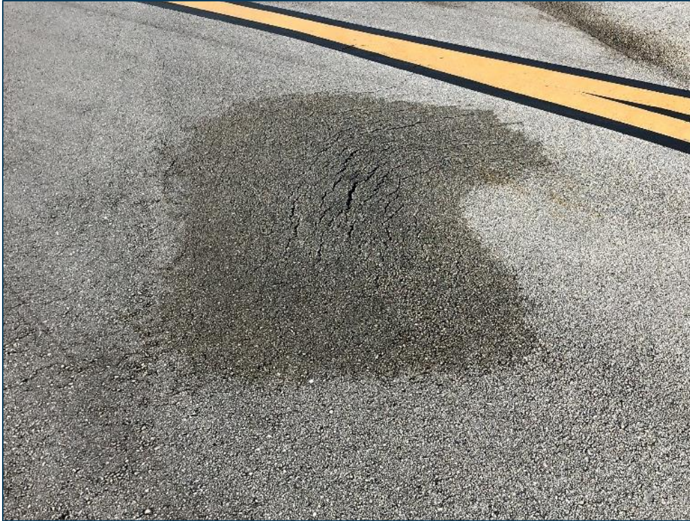
TW F, Section 605, Sample Unit 110 - Low Severity (52) Raveling, (55) Slippage Cracking, and Low Severity (57) Weathering
