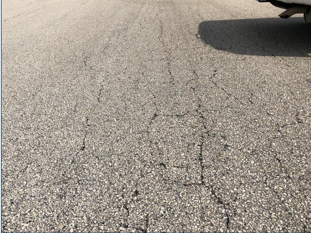
TW B, Section 220, Sample Unit 165 – Low and Medium Severity (41) Alligator Cracking, Low Severity (52) Raveling, Low Severity (53) Rutting, and Medium Severity (57) Weathering
