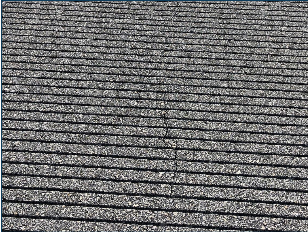
RW 10L-28R, Section 6105, Sample Unit 445 - Low Severity (48) Longitudinal & Transverse Cracking and Low Severity (57) Weathering
