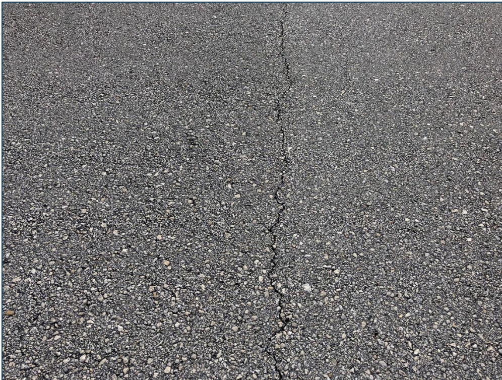
TW L, Section 1075, Sample Unit 216 - Low Severity (48) Longitudinal & Transverse Cracking, Low and Medium Severity (57) Weathering
