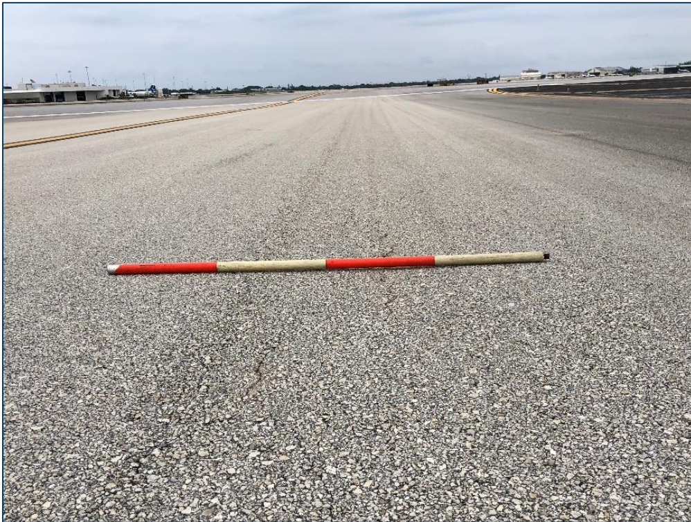
TW C, Section 312, Sample Unit 161 - Low Severity (48) Longitudinal & Transverse Cracking, Low Severity (53) Rutting, Low and Medium Severity (57) Weathering
