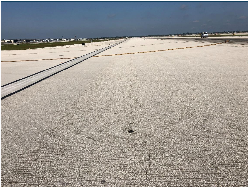
RW 10L-28R, Section 6110, Sample Unit 604 - Low Severity (48) Longitudinal & Transverse Cracking and Low Severity (57) Weathering
