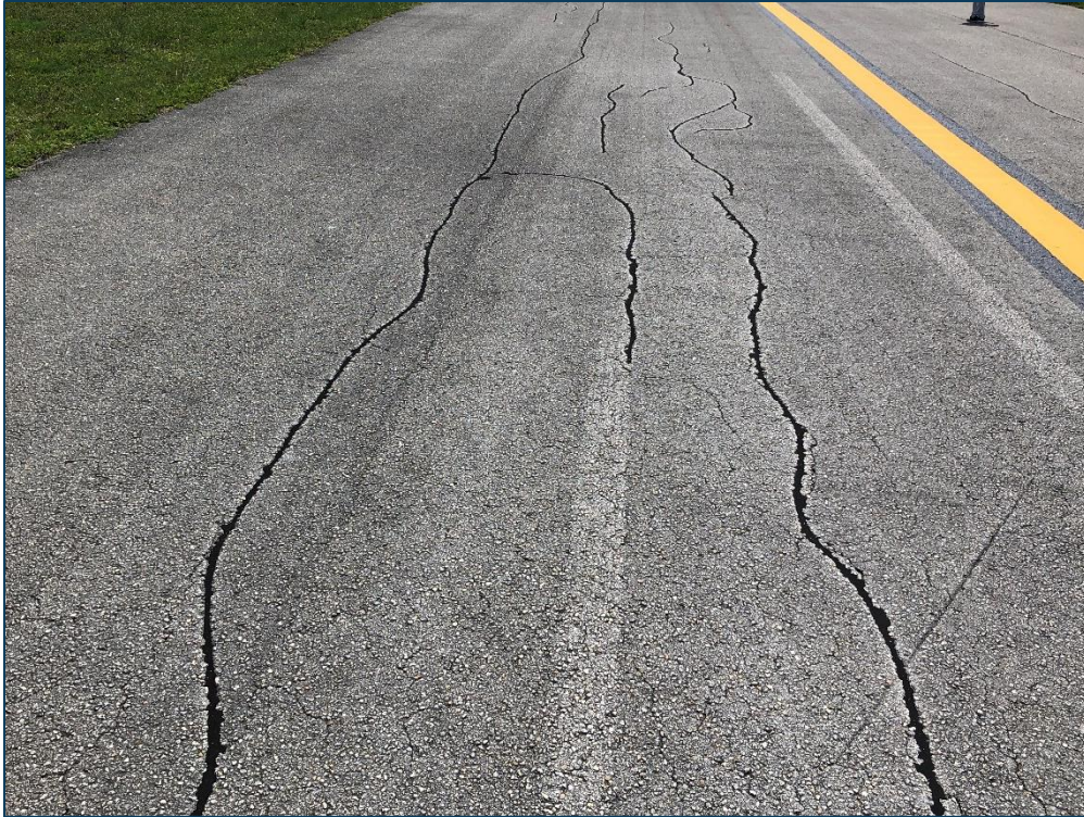
TW R, Section 1805, Sample Unit 215 - Low Severity (48) Longitudinal & Transverse Cracking, Low Severity (52) Raveling, and Low Severity (53) Rutting
