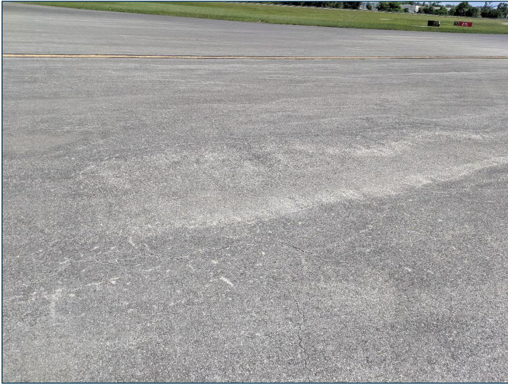
TW Y, Section 2620, Sample Unit 158 - Severity (45) Depression, Low Severity (48) Longitudinal & Transverse Cracking, Low Severity (52) Raveling, and Medium Severity (57) Weathering
