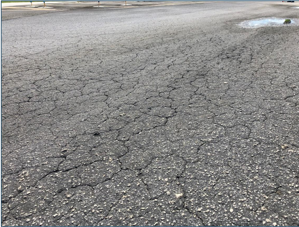
TW P, Section 1650, Sample Unit 102 - Low Severity (41) Alligator Cracking, Medium Severity (41) Alligator Cracking, Low Severity (52) Raveling, and Low Severity (53) Rutting
