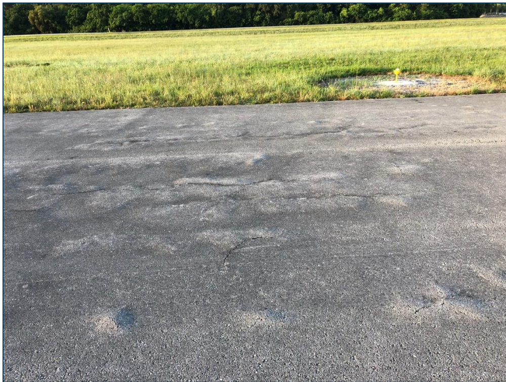
RW 9R-27L, Section 6410, Sample Unit 171 - Low Severity (48) Longitudinal & Transverse Cracking, Medium Severity (48) Longitudinal & Transverse Cracking, Low Severity (52) Raveling, Medium Severity (52) Raveling, Low Severity (56) Swelling, and Medium Severity (56) Swelling
