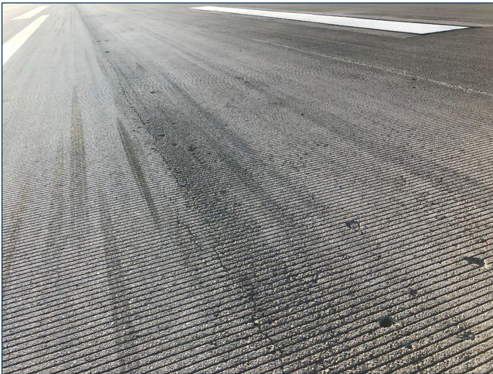
RW 9L-27R, Section 6115, Sample Unit 355 - Severity (48) Longitudinal & Transverse Cracking, Medium Severity (48) Longitudinal & Transverse Cracking, Low Severity (56) Swelling, Low Severity (57) Weathering, and Medium Severity (57) Weathering
