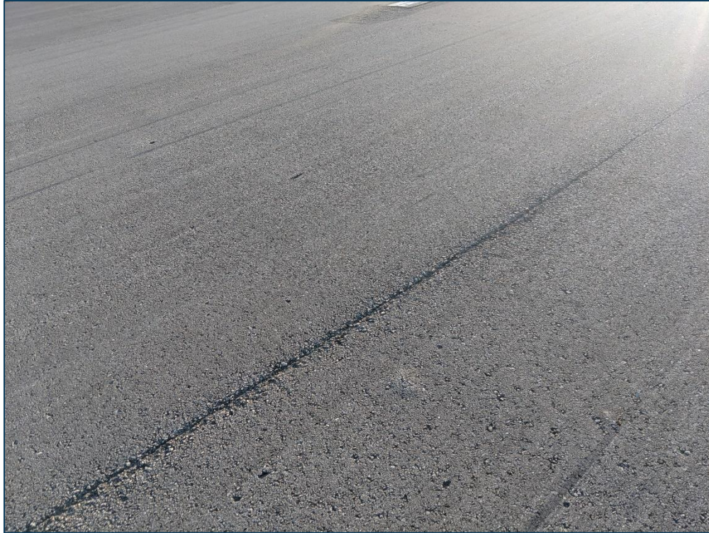
RW 9R-27L, Section 6405, Sample Unit 159 - Medium Severity (48) Longitudinal & Transverse Cracking, Low Severity (52) Raveling, and Medium Severity (52) Raveling
