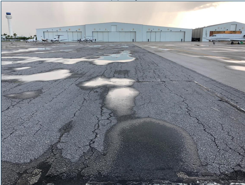
AP T-HANG, Section 4507, Sample Unit 258 - Low Severity (41) Alligator Cracking, Medium Severity (43) Block Cracking, Low Severity (45) Depression, and Medium Severity (52) Raveling
