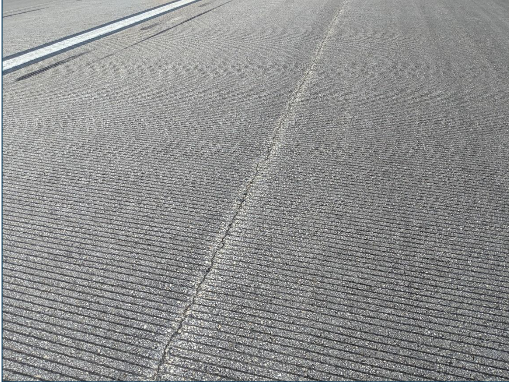
RW 12-30, Section 6205, Sample Unit 308 - Low Severity (48) Longitudinal & Transverse Cracking, Medium Severity (48) Longitudinal & Transverse Cracking, and Medium Severity (57) Weathering
