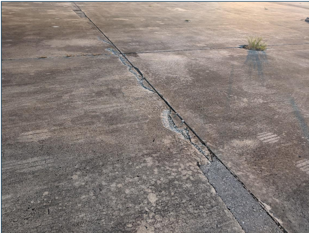
AP CENTER, Section 4110, Sample Unit 309 - Medium Severity (65) Joint Seal Damage, Medium Severity (66) Small Patch, (73) Shrinkage Cracking, and High Severity (74) Joint Spall
