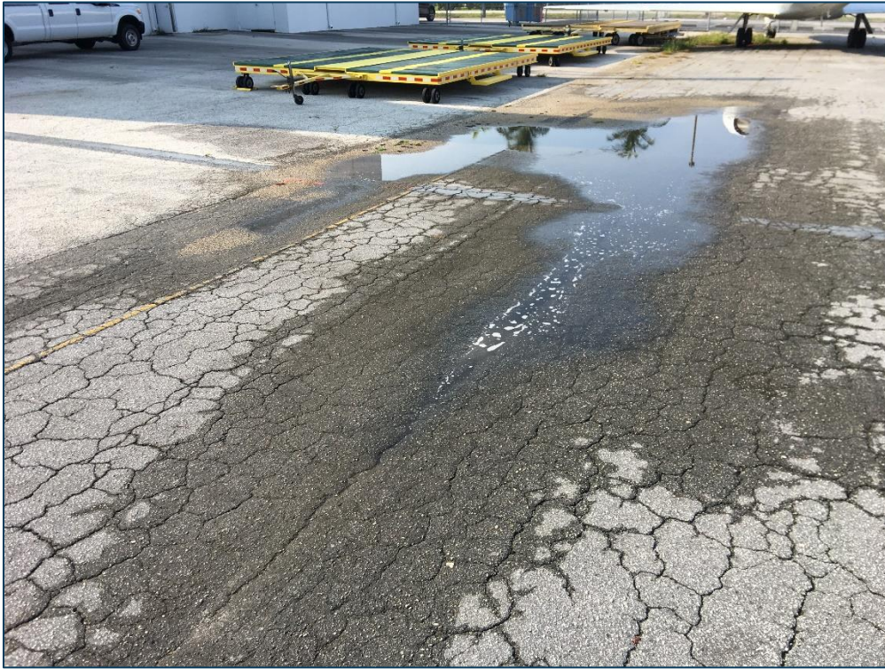
AP E, Section 4231, Sample Unit 152 - Medium Severity (41) Alligator Cracking, Low Severity (52) Raveling, and Medium Severity (53) Rutting
