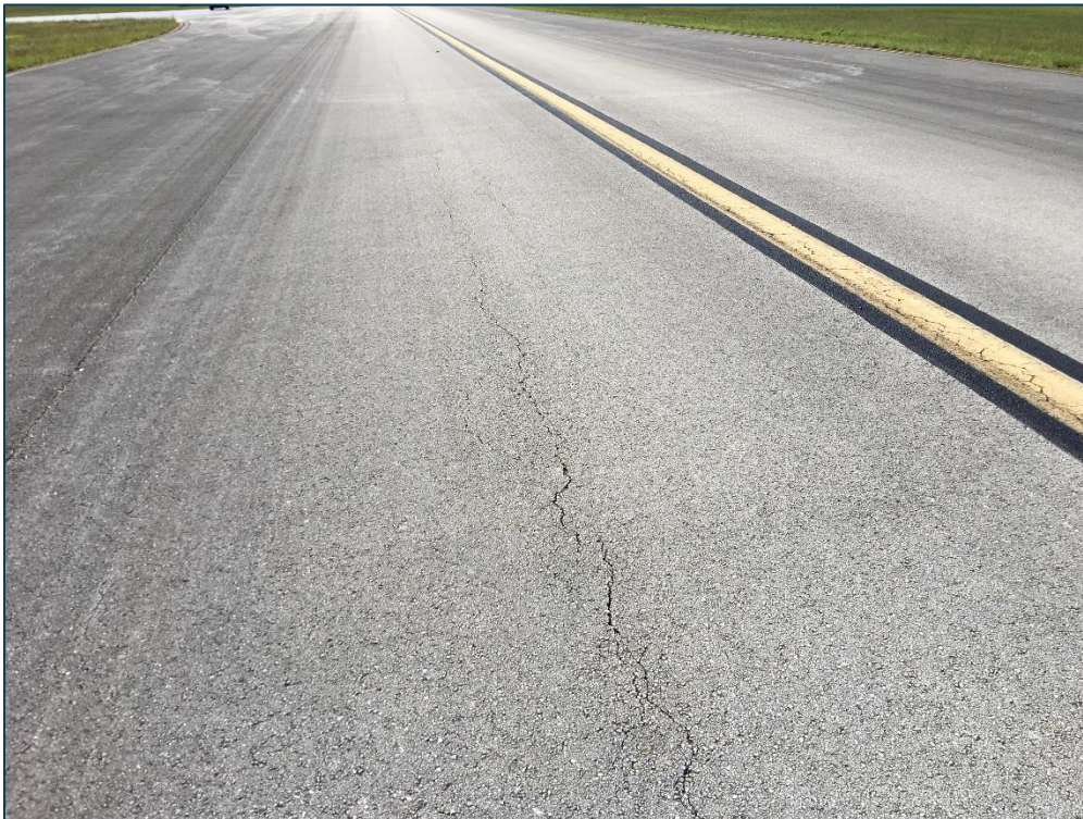
TW T, Section 2005, Sample Unit 119 - Low Severity (48) Longitudinal & Transverse Cracking, Medium Severity (48) Longitudinal & Transverse Cracking, Low Severity (52) Raveling, and Medium Severity (57) Weathering
