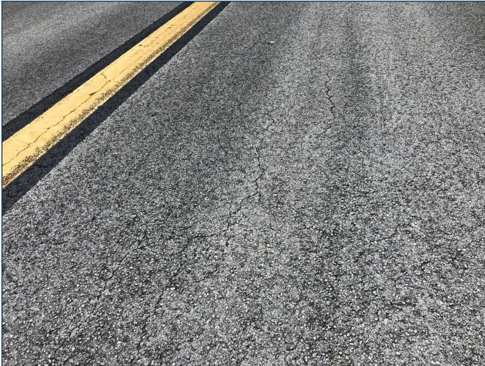
TW G, Section 720, Sample Unit 115 - Low Severity (48) Longitudinal & Transverse Cracking, Low Severity (52) Raveling, and Medium Severity (52) Raveling
