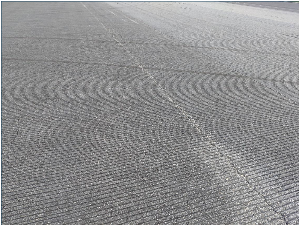
RW 12-30, Section 6205, Sample Unit 381 - Low Severity (48) Longitudinal & Transverse Cracking, Medium Severity (48) Longitudinal & Transverse Cracking, and Medium Severity (57) Weathering
