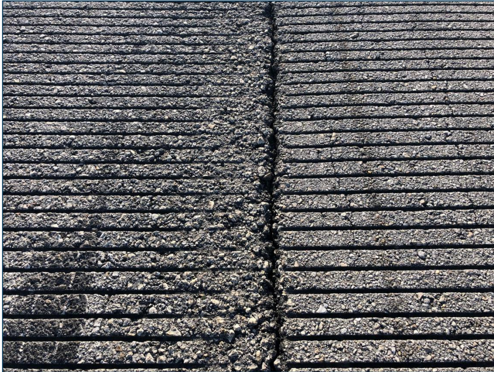
RW 9L-27R, Section 6115, Sample Unit 330 - Low Severity (48) Longitudinal & Transverse Cracking, Medium Severity (48) Longitudinal & Transverse Cracking, Low Severity (57) Weathering, and Medium Severity (57) Weathering
