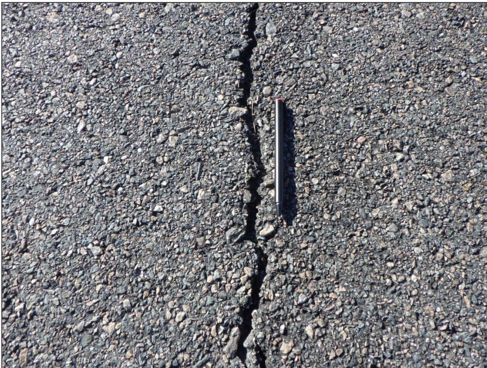
RW 9R-27L, Section 6315, Sample Unit 346 - Longitudinal & Transverse Cracking
