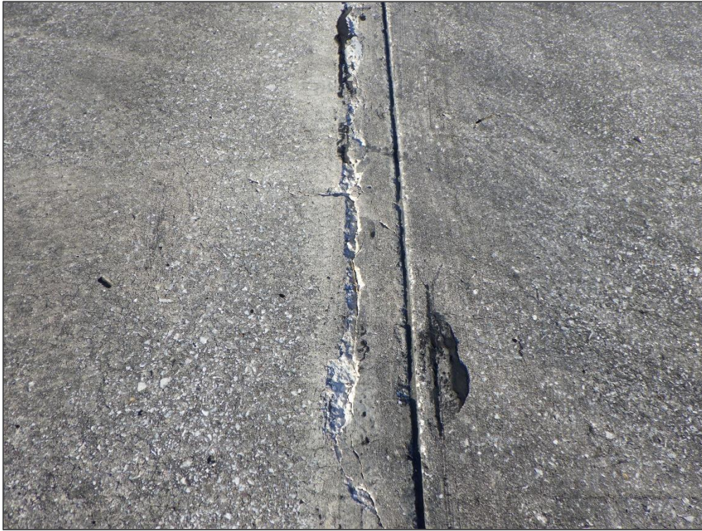
AP N, Section 4120, Sample Unit 288 - Joint Spall
