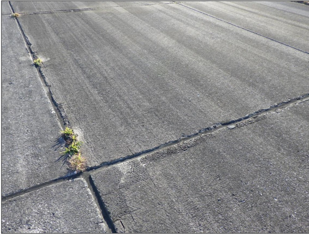
RW 9R-27L, Section 6340, Sample Unit 780 – Joint Seal Damage and Patching
