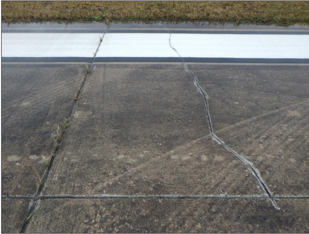
RW 18L-36R, Section 6240, Sample Unit 853 - Linear Cracking
