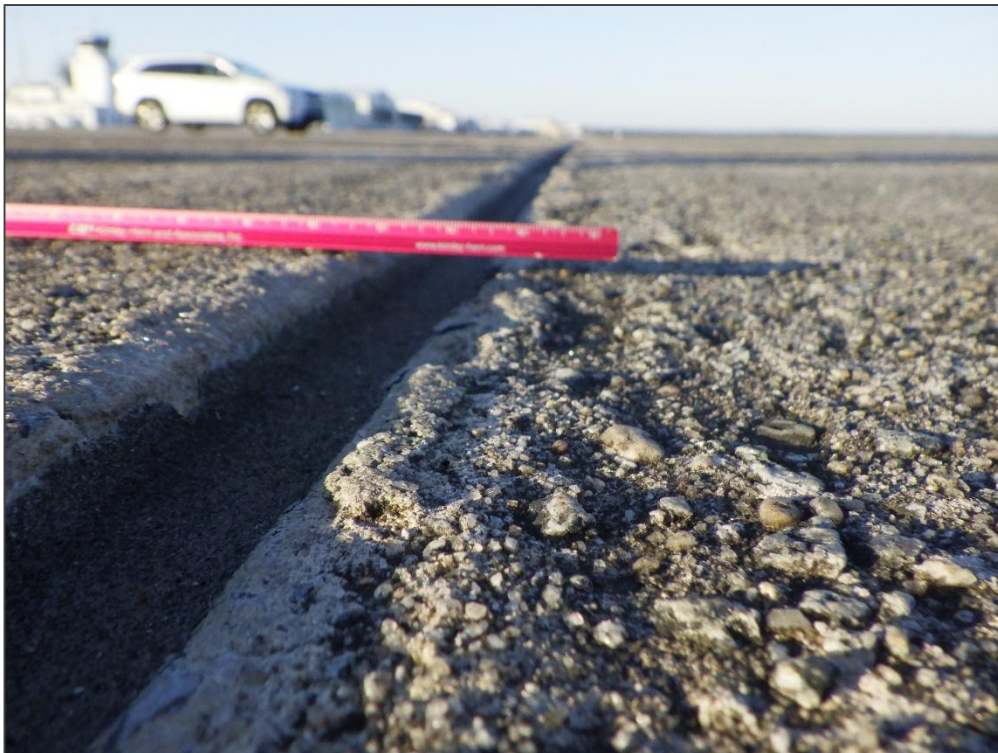
TW C, Section 305, Sample Unit 109 - Faulting
