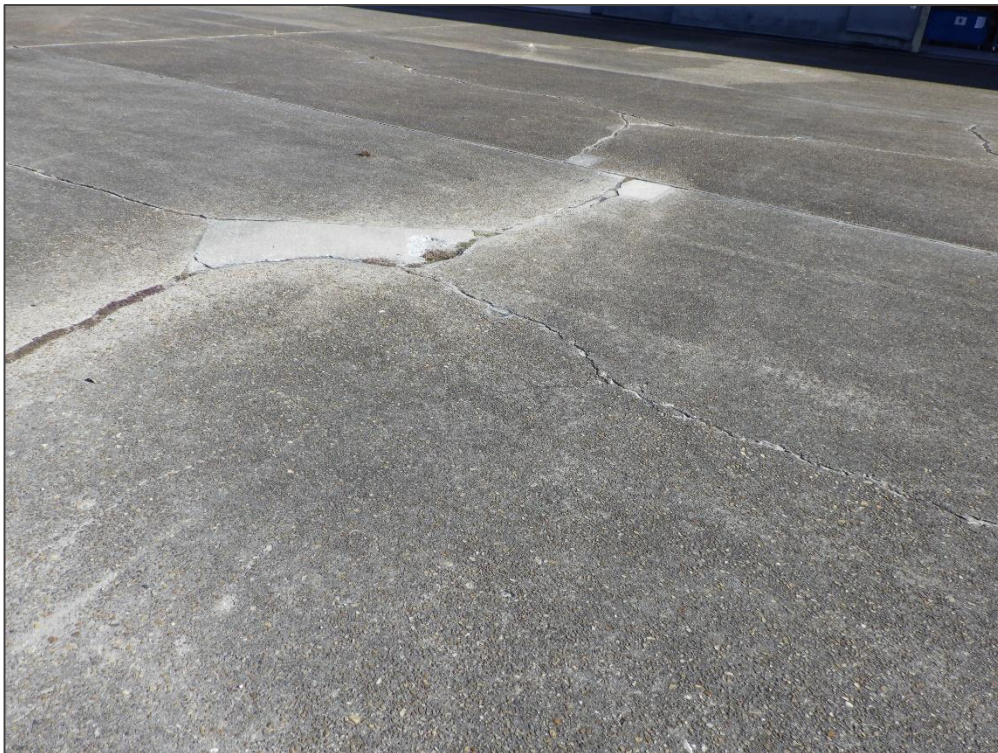
AP W, Section 4225, Sample Unit 101 - Shattered Slab
