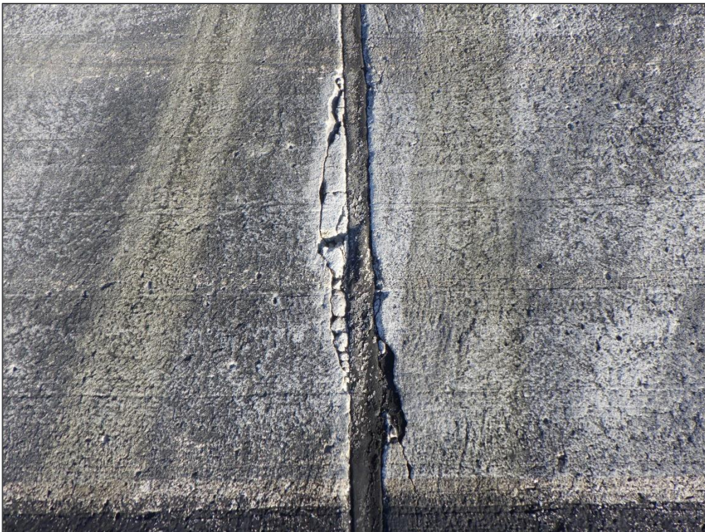
RW 9R-27L, Section 6335, Sample Unit 384 - Joint Spall
