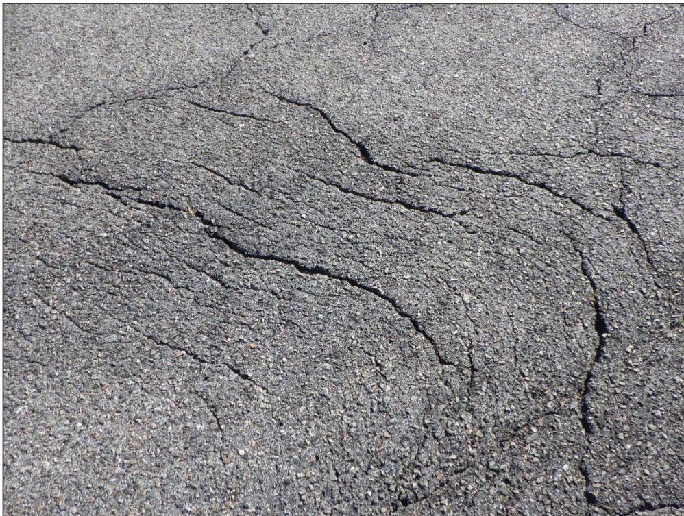
RW 18R-36L, Section 6115, Sample Unit 313 - Slippage Cracking
