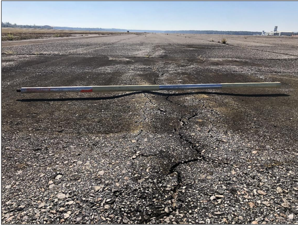
RW 18R-36L, Section 6120, Sample Unit 116 - Longitudinal & Transverse Cracking and Swelling
