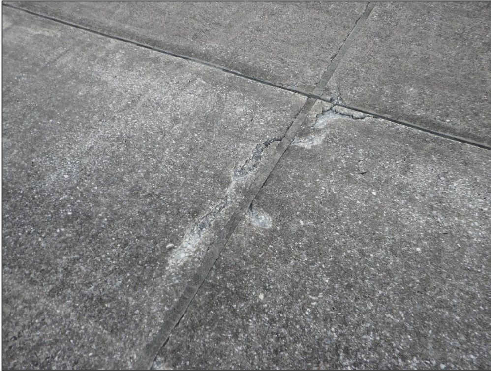
TW D, Section 405, Sample Unit 468 - Joint Spall
