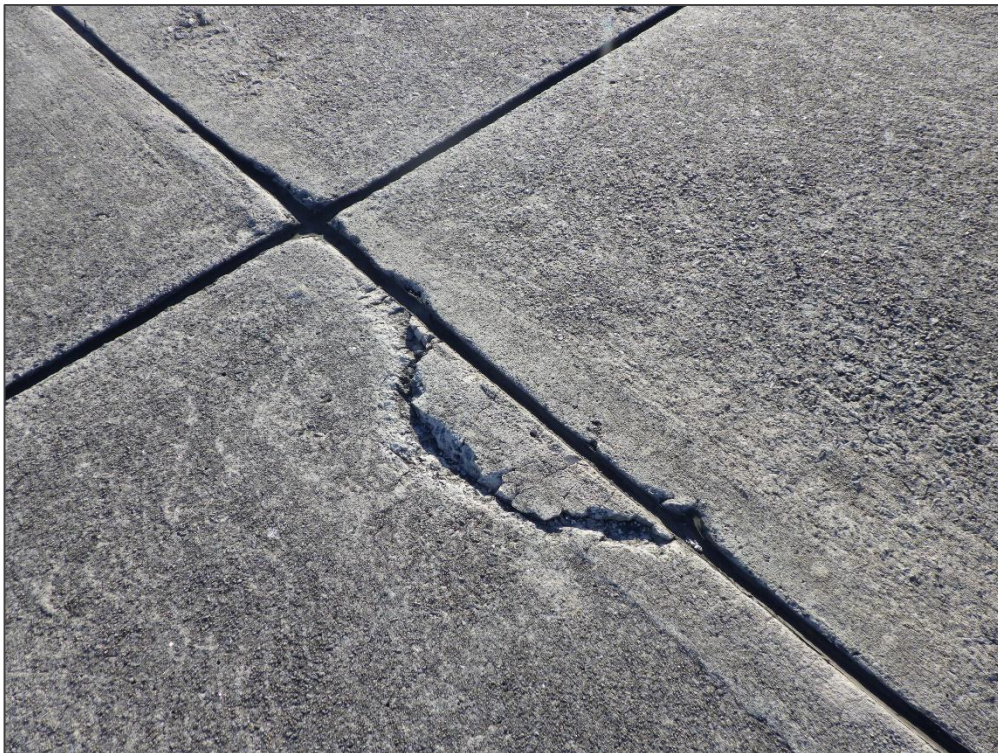
TW A, Section 130, Sample Unit 176 - Joint Spall
