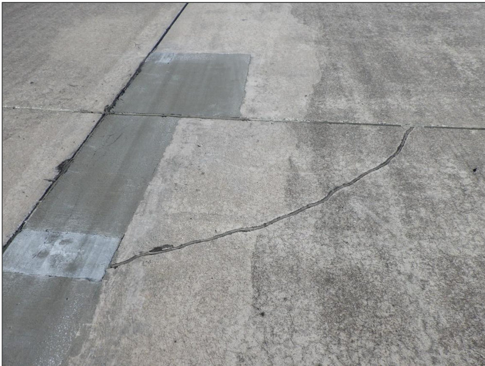
TW A, Section 105, Sample Unit 309 - Corner Break and Large Patch/Utility Cut
