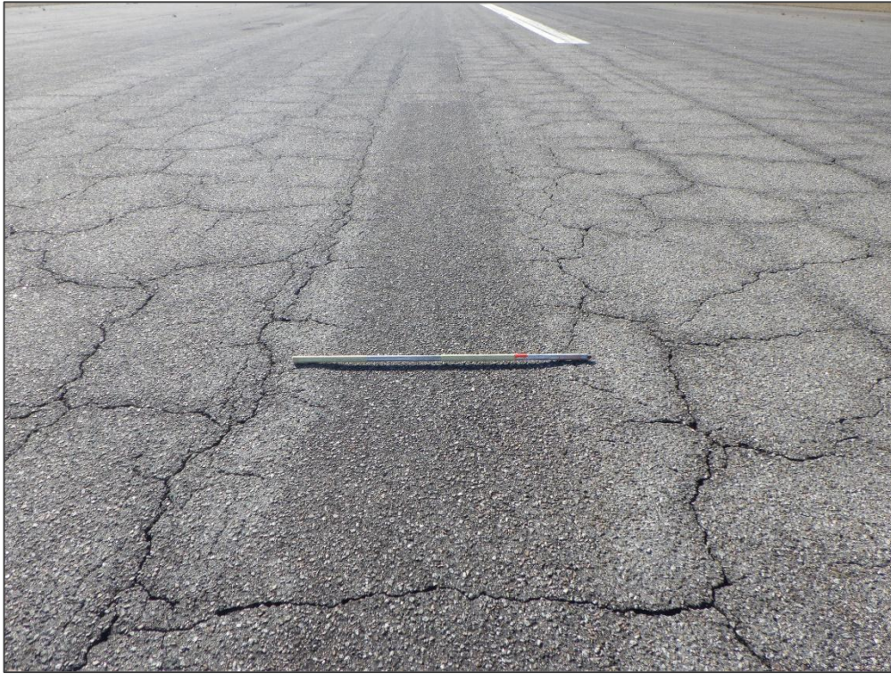
RW 18R-36L, Section 6115, Sample Unit 229 - Block Cracking and Rutting
