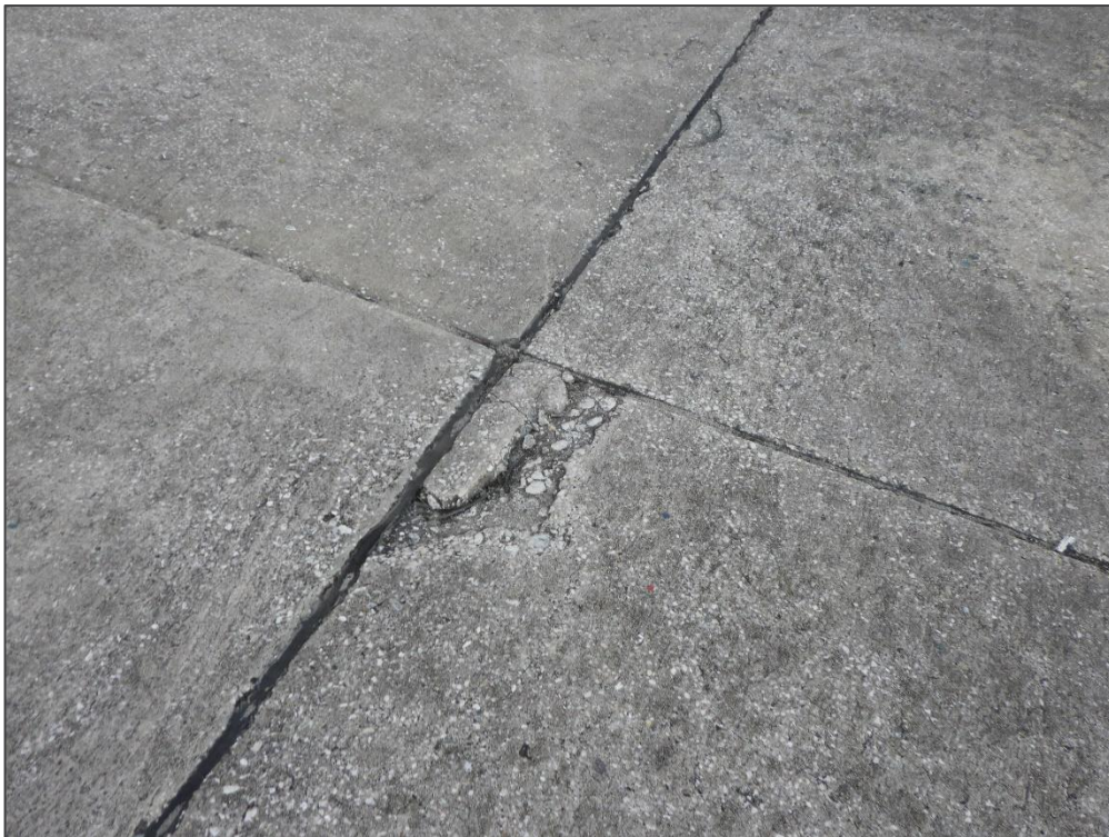
AP N, Section 4110, Sample Unit 408 – Corner Spall
