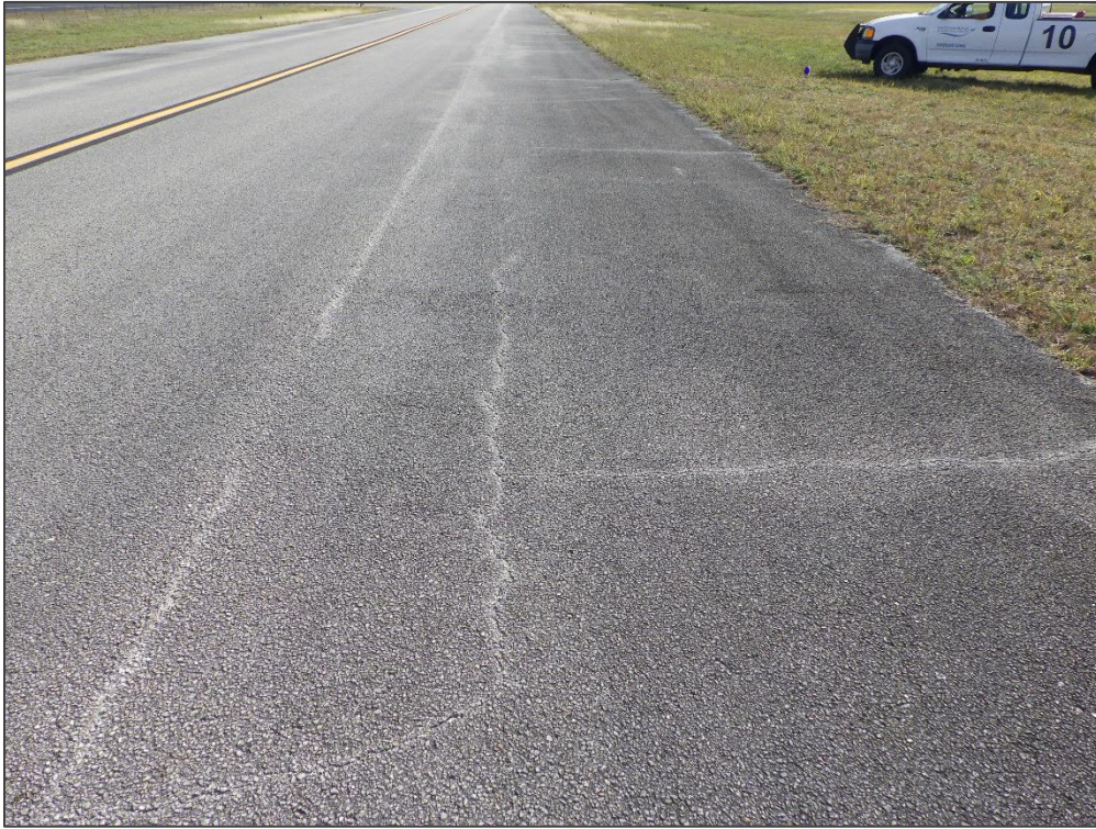
TW E, Section 515, Sample Unit 141 – Longitudinal & Transverse Cracking
