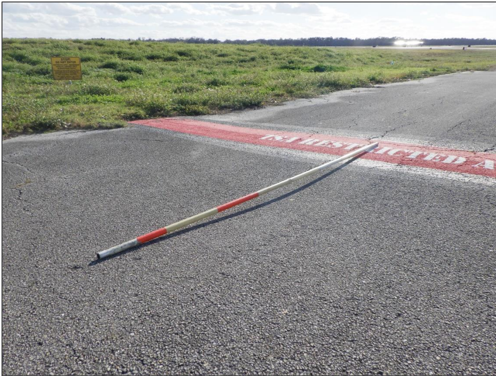
TW S, Section 1950, Sample Unit 213 – Depression and Longitudinal & Transverse Cracking
