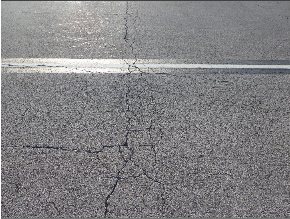
AP GA, Section 4215, Sample Unit 164 – Alligator Cracking
