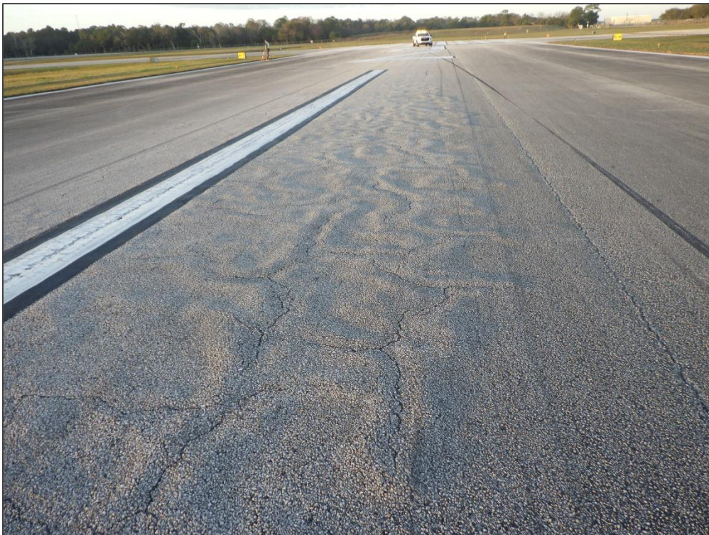
RW 7R-25L, Section 6305, Sample Unit 109 – Block Cracking and Swelling
