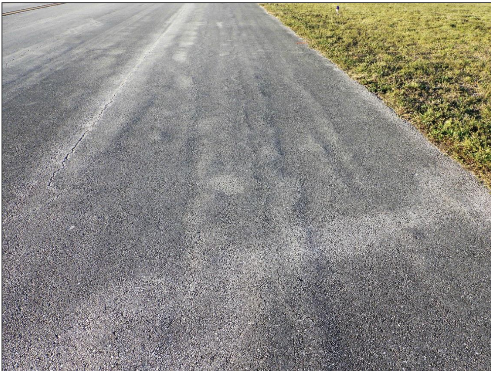
TW W, Section 2340, Sample Unit 309 – Longitudinal & Transverse Cracking and Swelling
