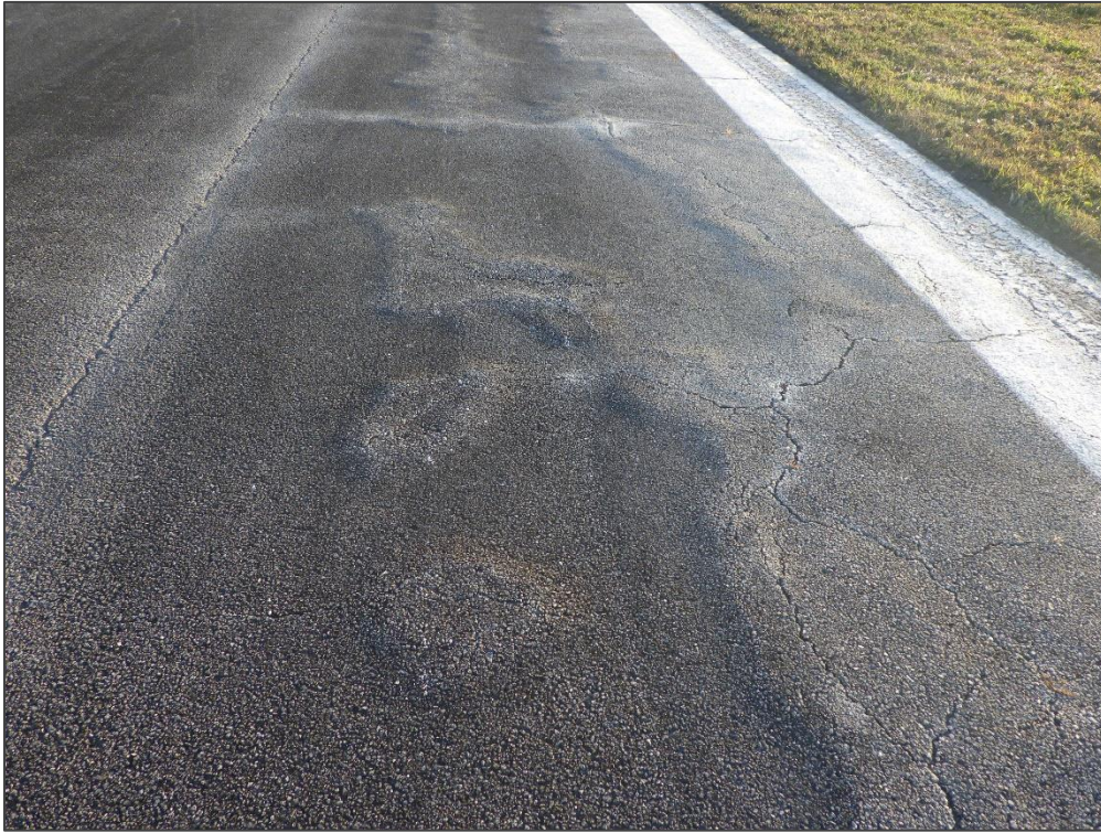
RW 7R-25L, Section 6305, Sample Unit 117 – Longitudinal & Transverse Cracking, Swelling
