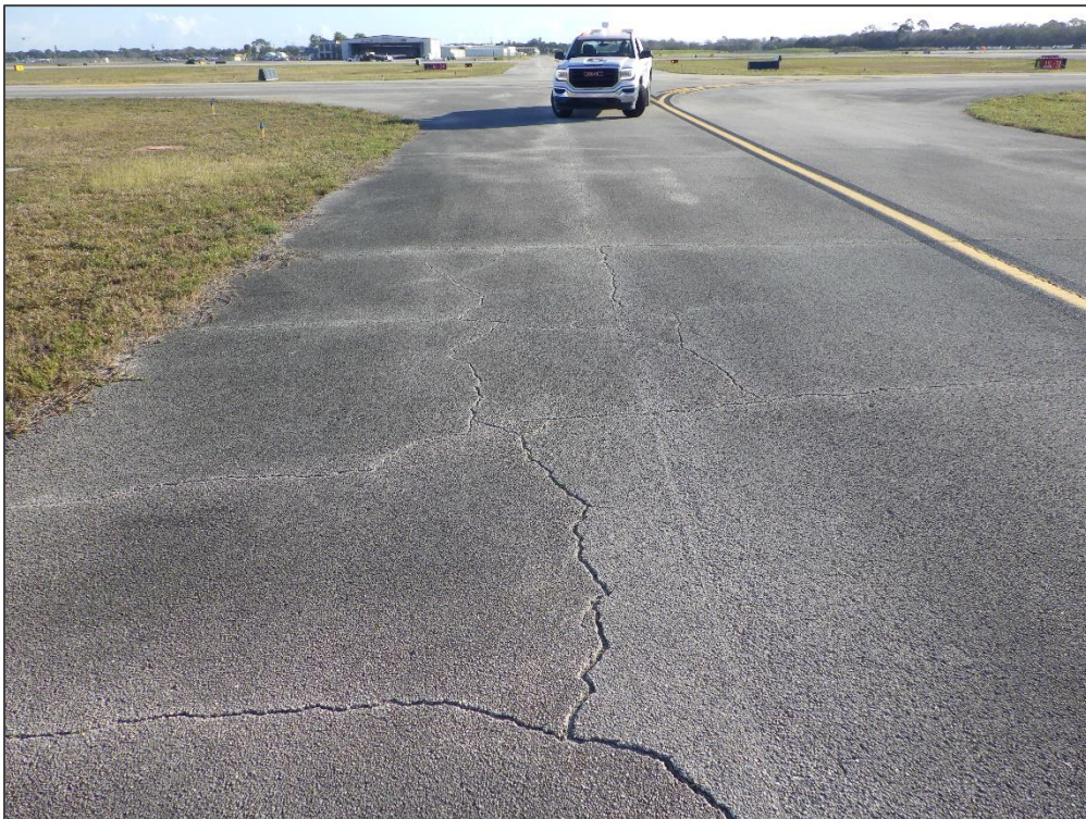
TW S, Section 1905, Sample Unit 104 – Block Cracking
