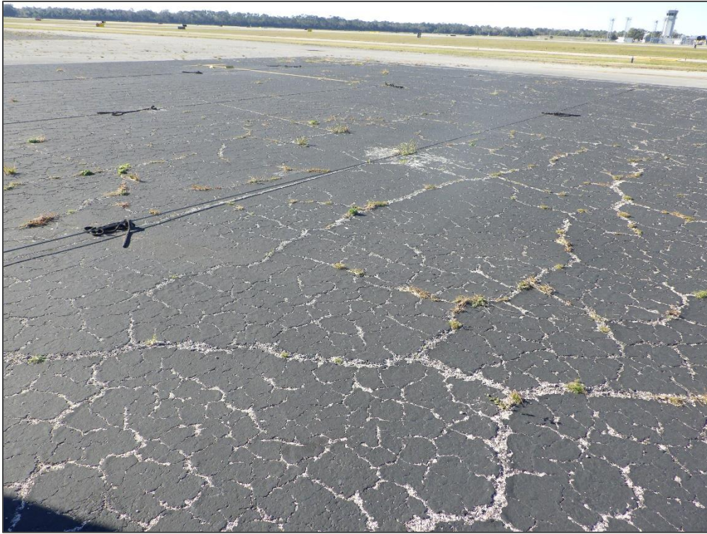
AP NOVA, Section 4305, Sample Unit 101 – Block Cracking and Raveling
