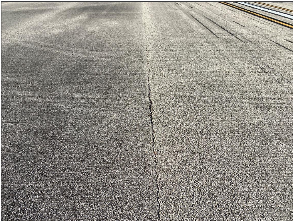
RW 16-34, Section 6205, Sample Unit 329 – Longitudinal & Transverse Cracking and Raveling
