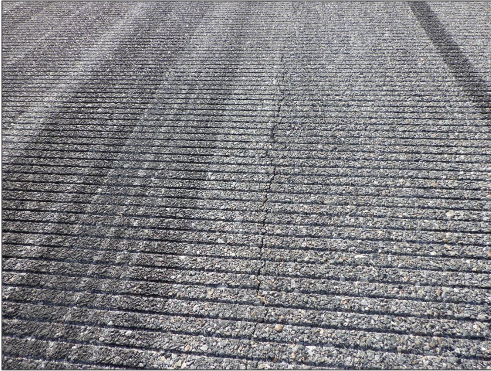
RW 7L-25R, Section 6160, Sample Unit 408 – Longitudinal & Transverse Cracking
