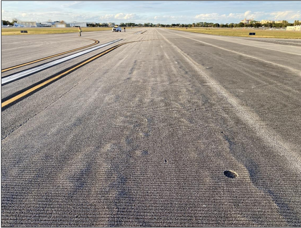
RW 16-34, Section 6215, Sample Unit 379 – Longitudinal & Transverse Cracking and Swelling
