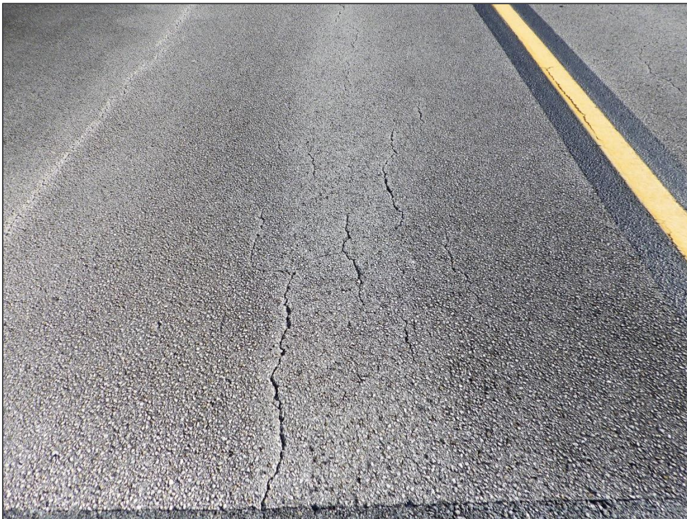
TW E, Section 512, Sample Unit 117 – Alligator Cracking
