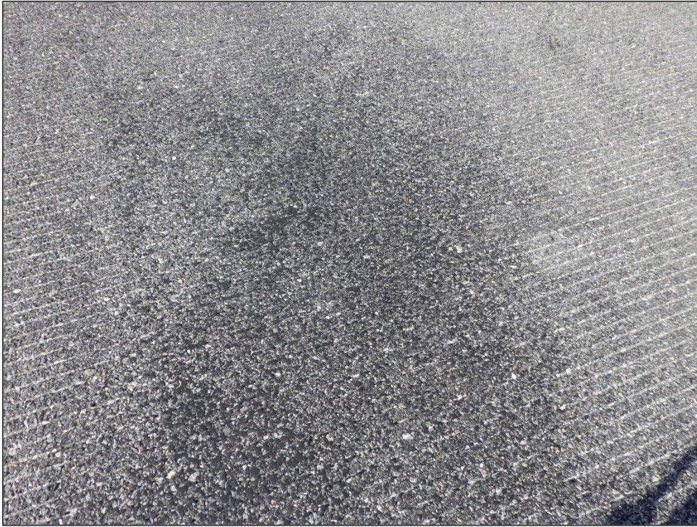
RW 7L-25R, Section 6130, Sample Unit 376 – Bleeding
