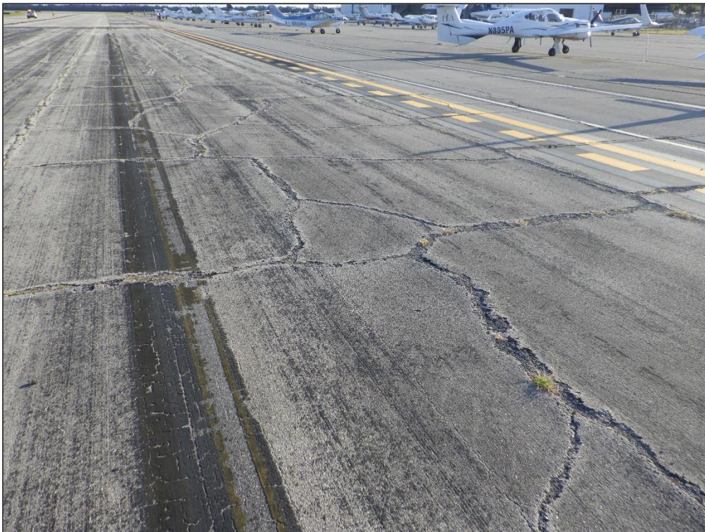
AP GA, Section 4220, Sample Unit 161 – Block Cracking
