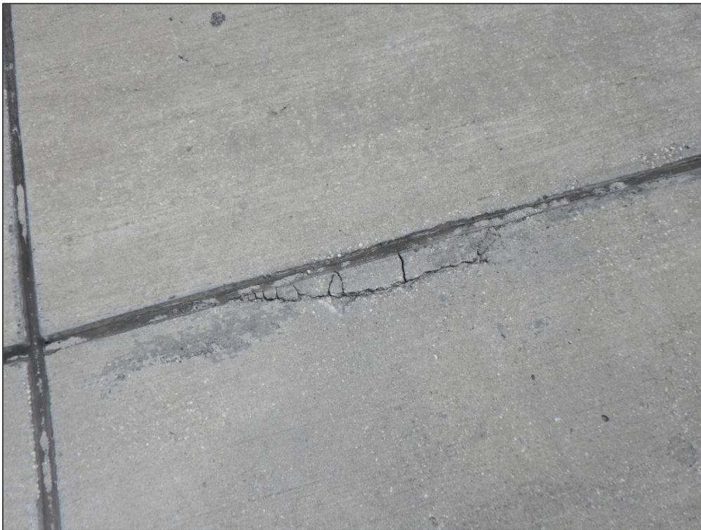
AP TERM 4, Section 4430, Sample Unit 268 – Joint Spall
