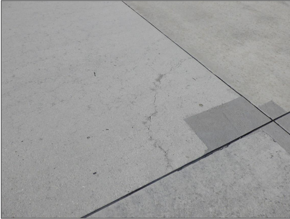
TW J, Section 905, Sample Unit 121 – Corner Break and Small Patch
