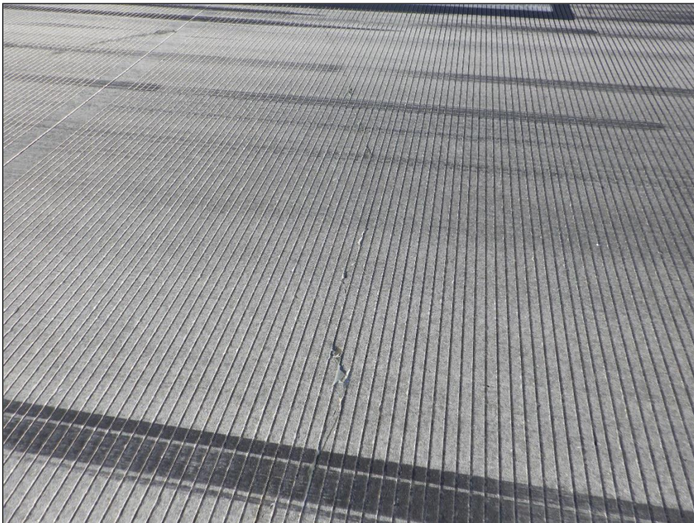
RW 10R-28L, Section 6205, Sample Unit 355 – Linear Cracking
