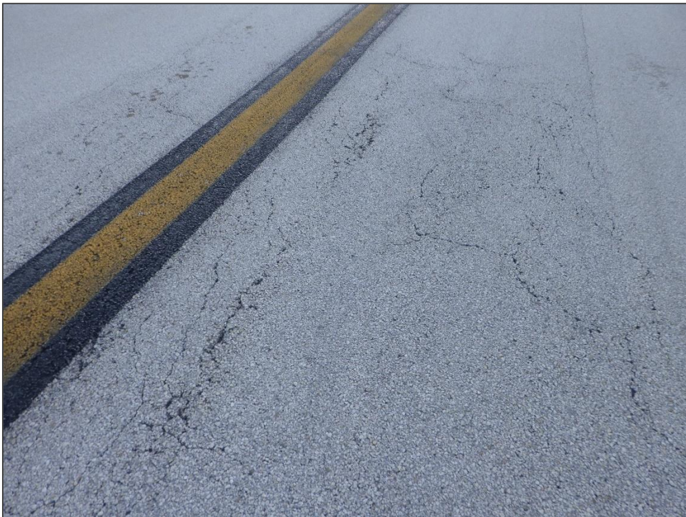
TW T, Section 2005, Sample Unit 100 – Alligator Cracking
