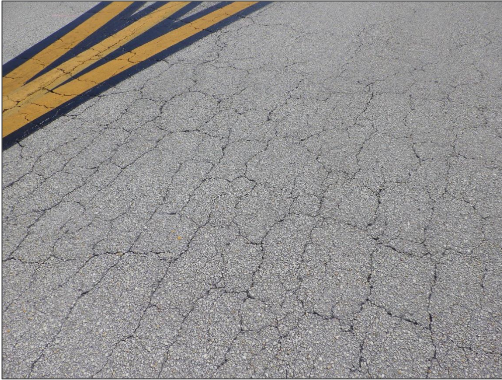
TW T6, Section 2055, Sample Unit 545 – Alligator Cracking
