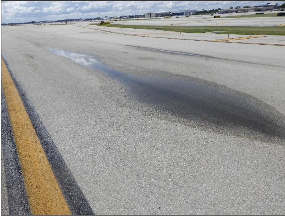
TW T, Section 2000, Sample Unit 409 – Rutting
