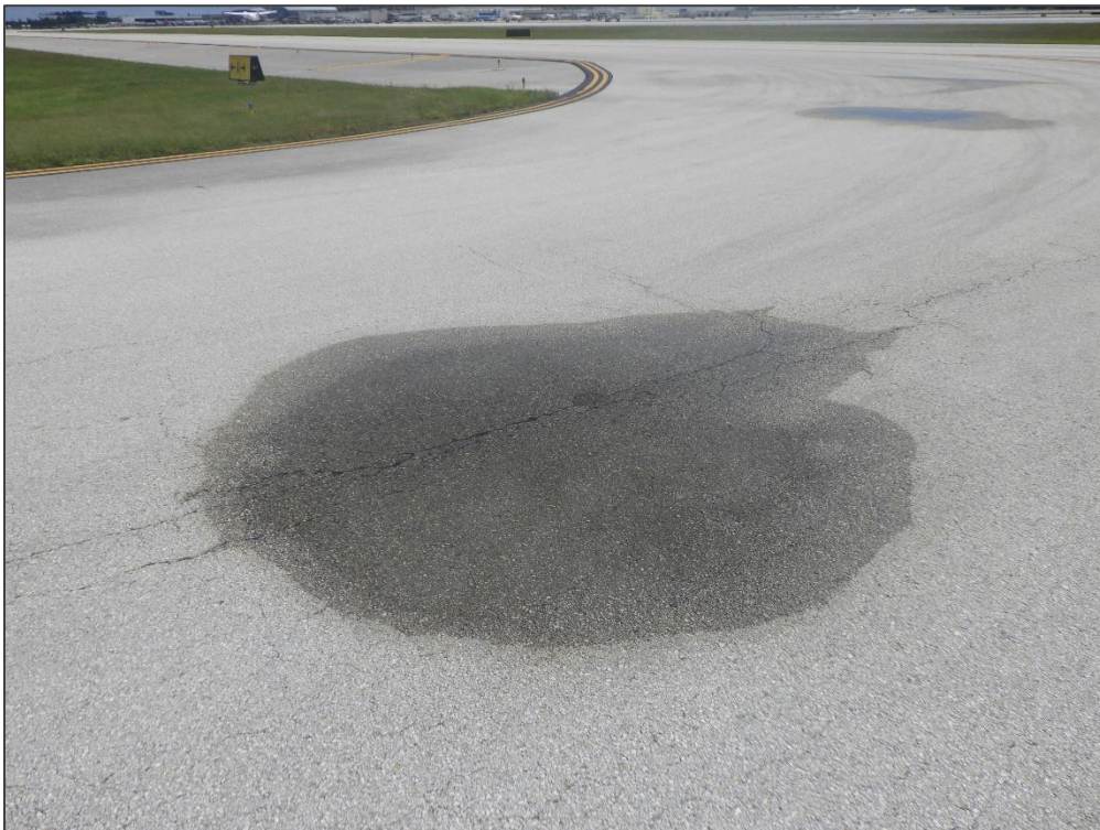
TW A, Section 126, Sample Unit 101 – Depression and Longitudinal & Transverse Cracking
