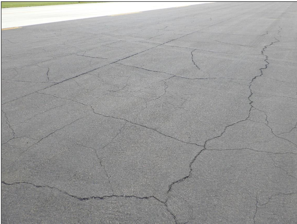
TW E, Section 524, Sample Unit 811 – Block Cracking
