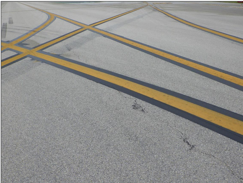
TW B, Section 230, Sample Unit 391 – Longitudinal & Transverse Cracking
