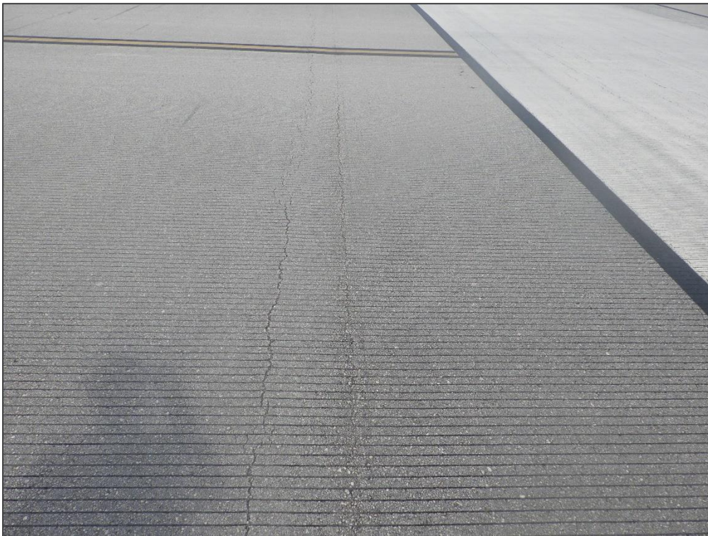
RW 13-31, Section 6210, Sample Unit 120 – Longitudinal & Transverse Cracking
