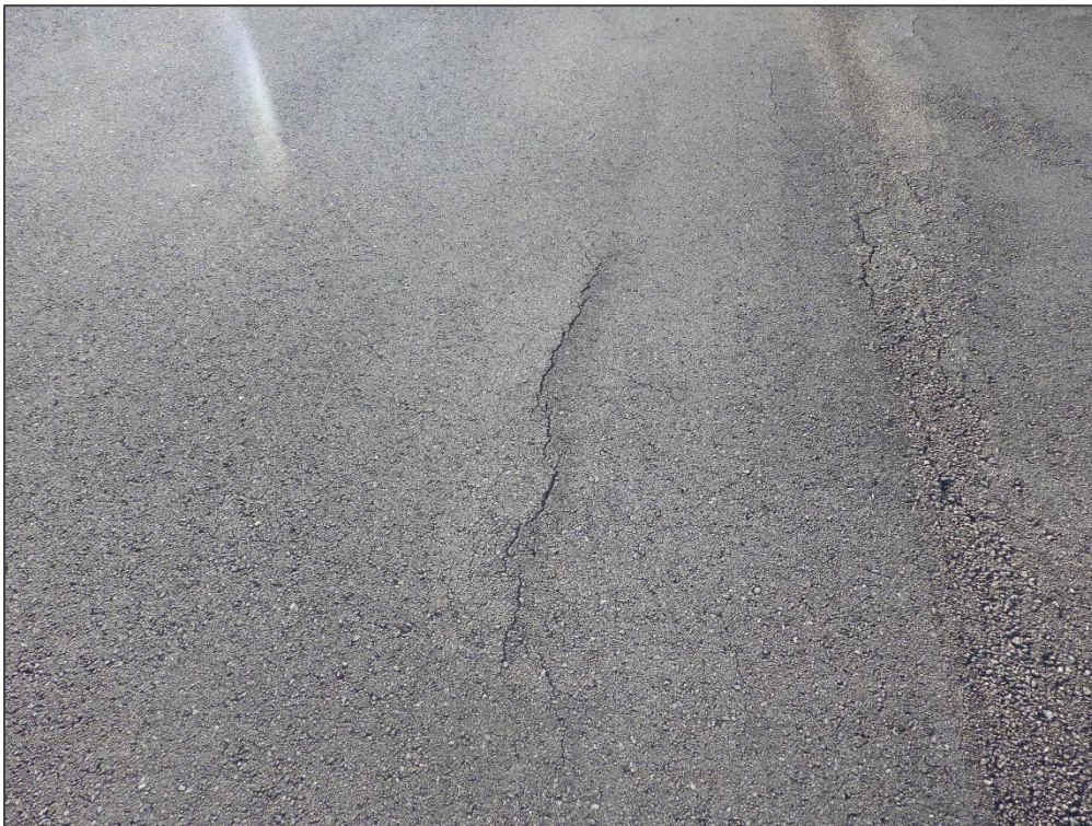
TW B, Section 210, Sample Unit 140 – Longitudinal & Transverse Cracking and Swelling
