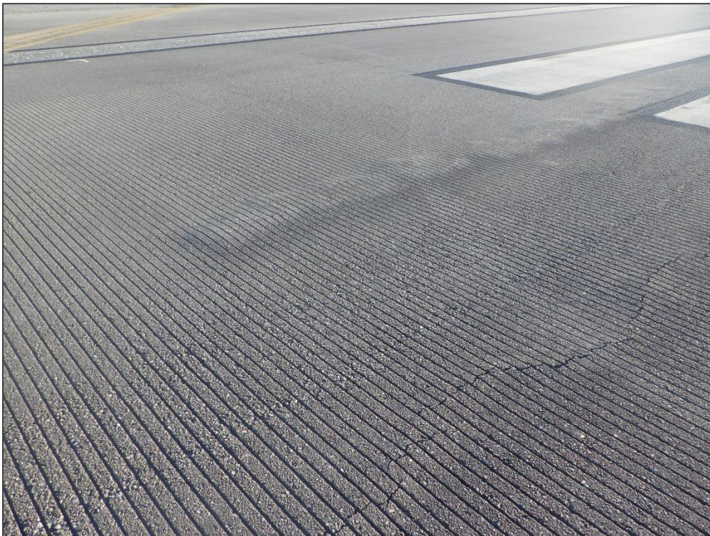
RW 9-27, Section 6105, Sample Unit 387 – Longitudinal & Transverse Cracking and Swelling
