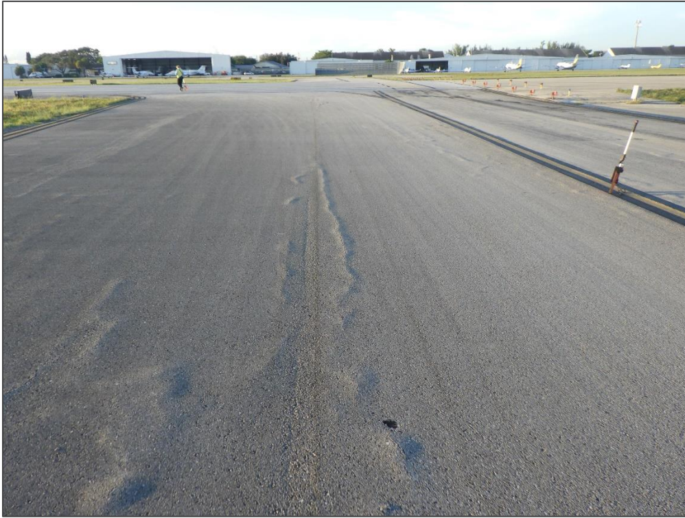
TW L, Section 1210, Sample Unit 101 – Longitudinal & Transverse Cracking and Swelling
