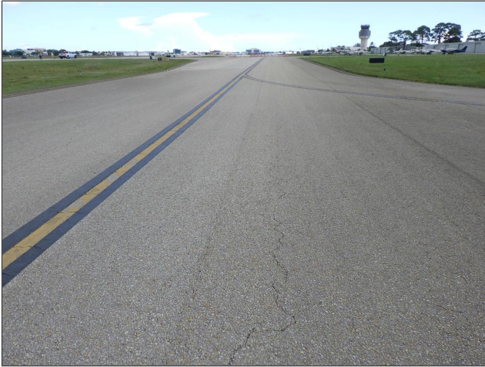
TW E, Section 520, Sample Unit 107 – Longitudinal & Transverse Cracking
