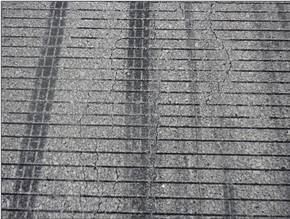
RW 9-27, Section 6105, Sample Unit 347 – Alligator Cracking
