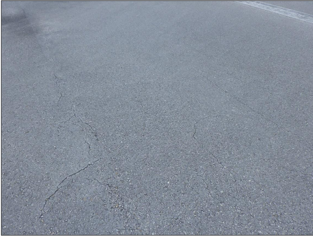
TW C, Section 320, Sample Unit 314 – Longitudinal & Transverse Cracking
