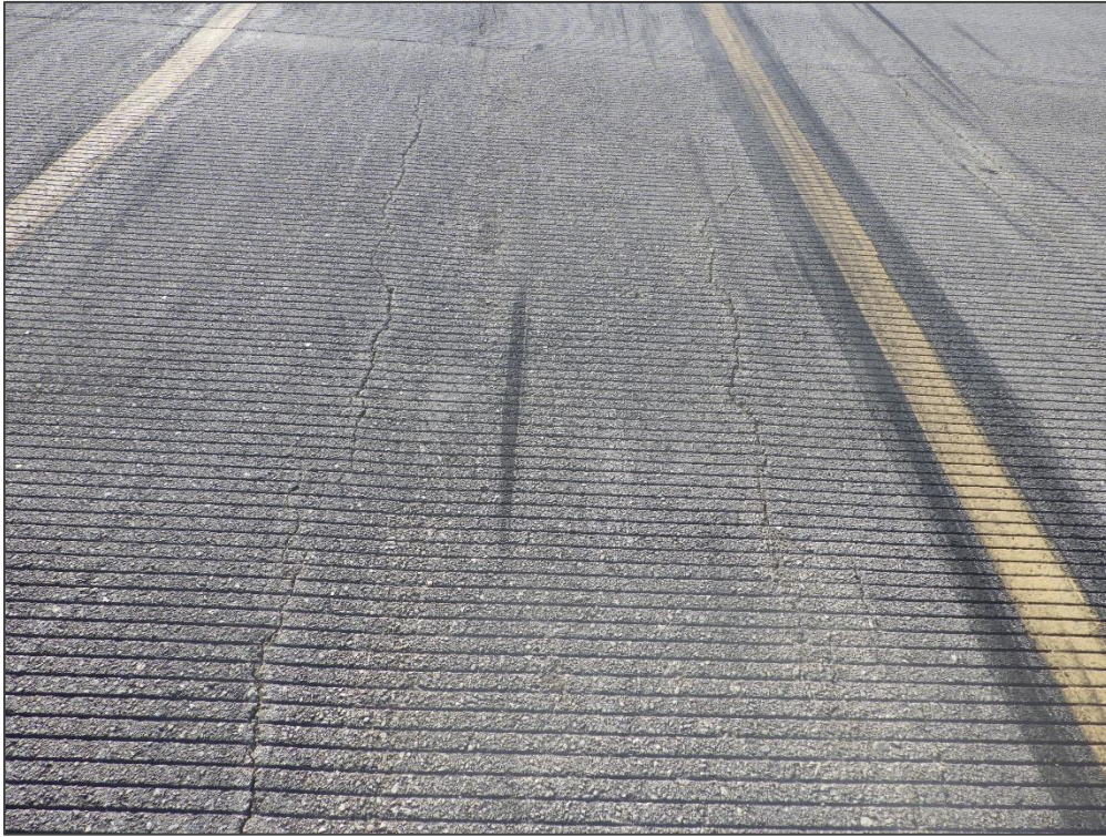
RW 13-31, Section 6205, Sample Unit 165 – Longitudinal & Transverse Cracking
