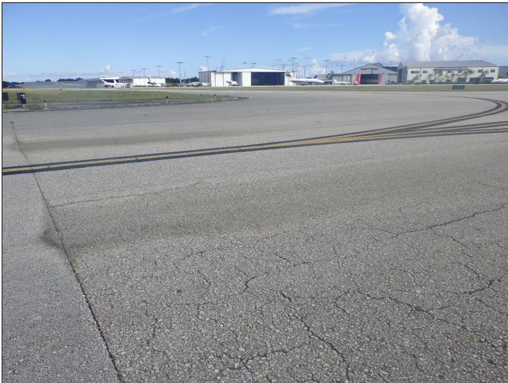
TW D, Section 414, Sample Unit 112 – Block Cracking and Rutting
