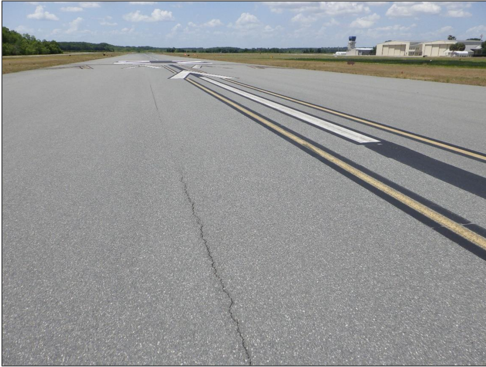
RW 4-22, Section 6205, Sample Unit 301 – Longitudinal & Transverse Cracking
