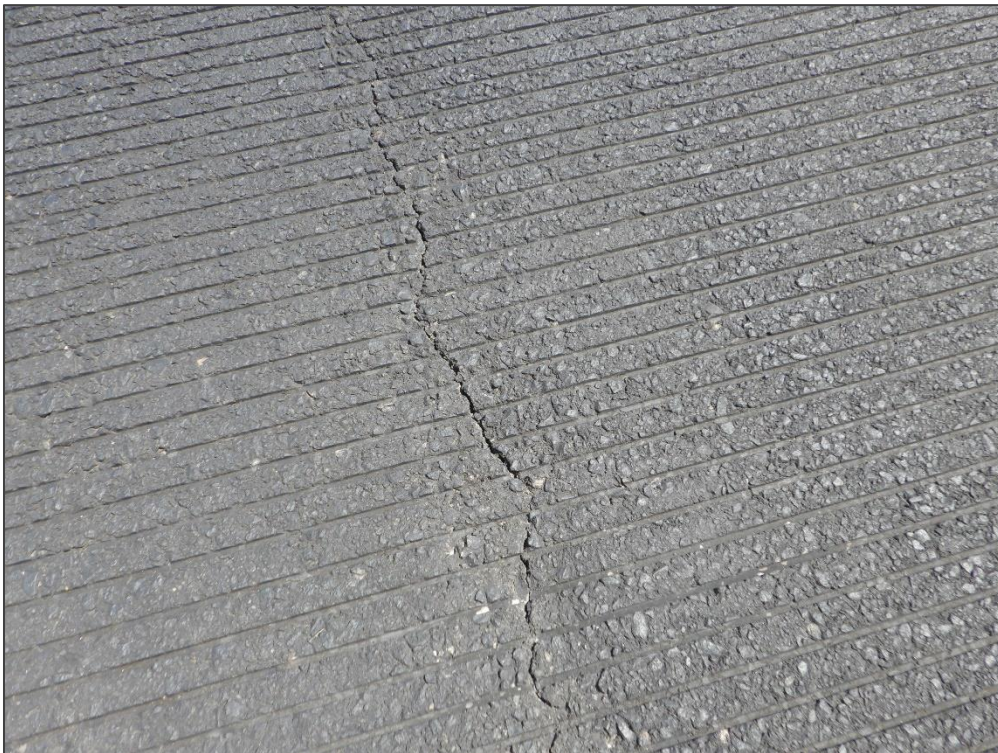
RW 13-31, Section 6125, Sample Unit 303 -- Longitudinal & Transverse Cracking
