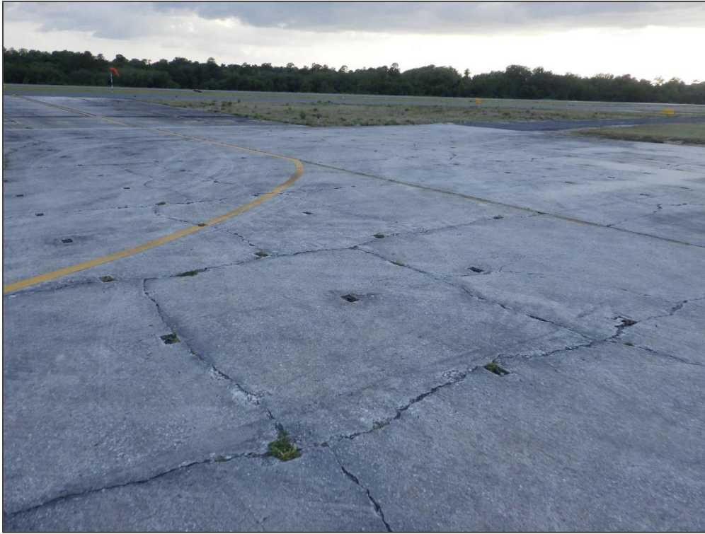
AP N, Section 4140, Sample Unit 602 – Shattered Slab
