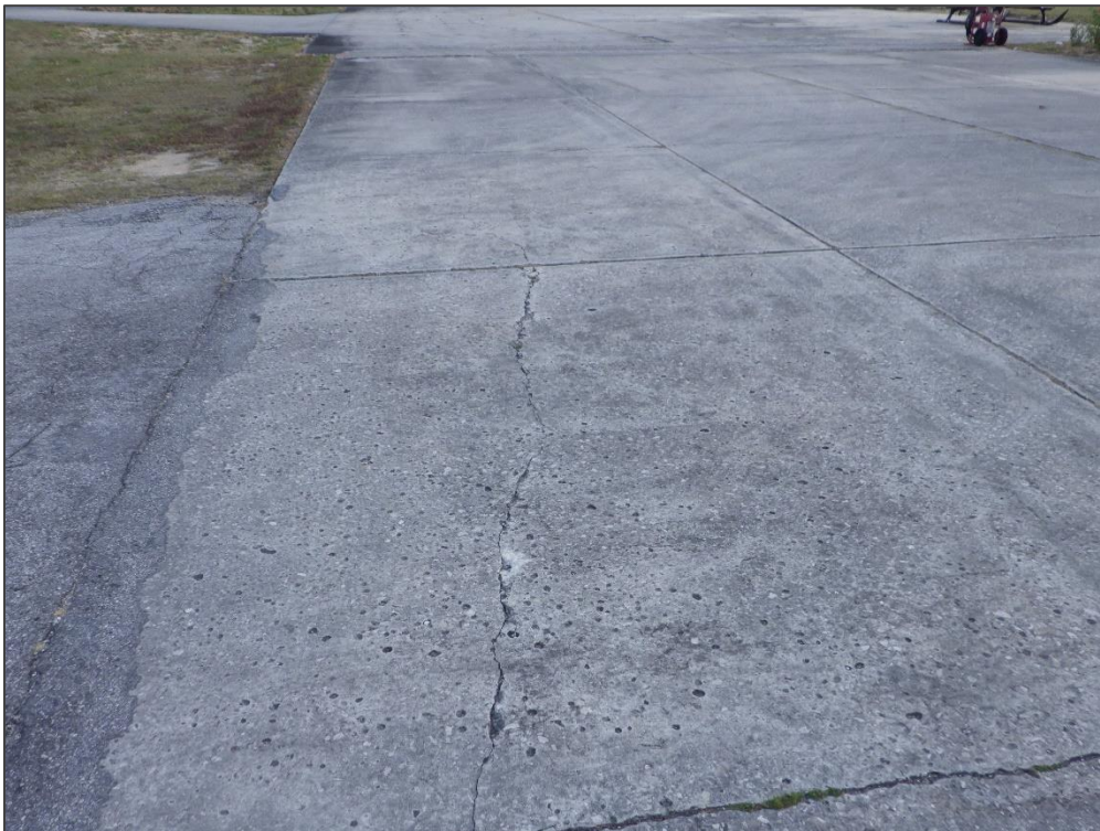
AP N, Section 4135, Sample Unit 604 – Linear Cracking
