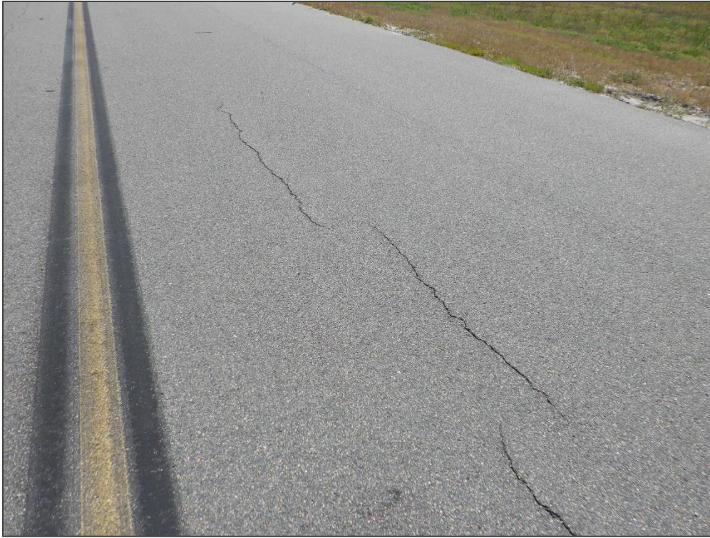
TW K, Section 700, Sample Unit 111 – Longitudinal & Transverse Cracking
