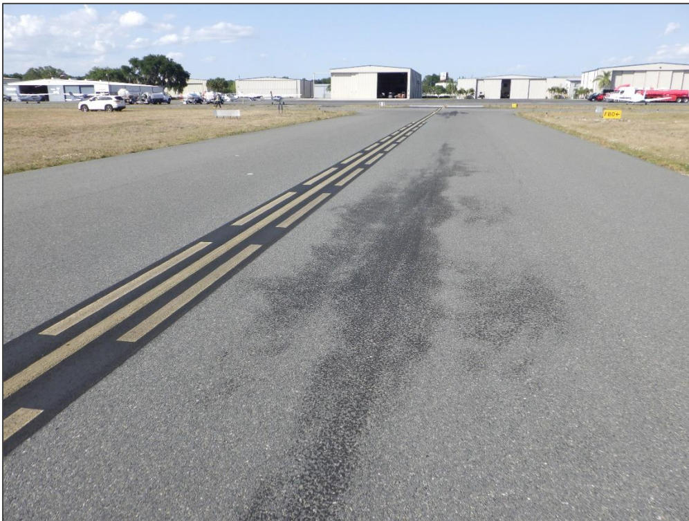
TW D, Section 400, Sample Unit 252 - Bleeding
