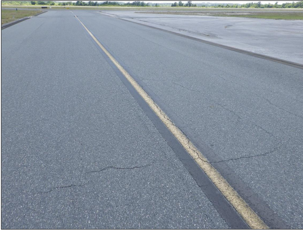
TW B, Section 200, Sample Unit 109 -- Longitudinal & Transverse Cracking
