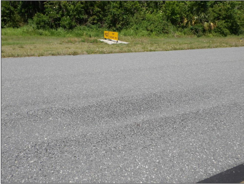
TW A, Section 100, Sample Unit 255 – Bleeding
