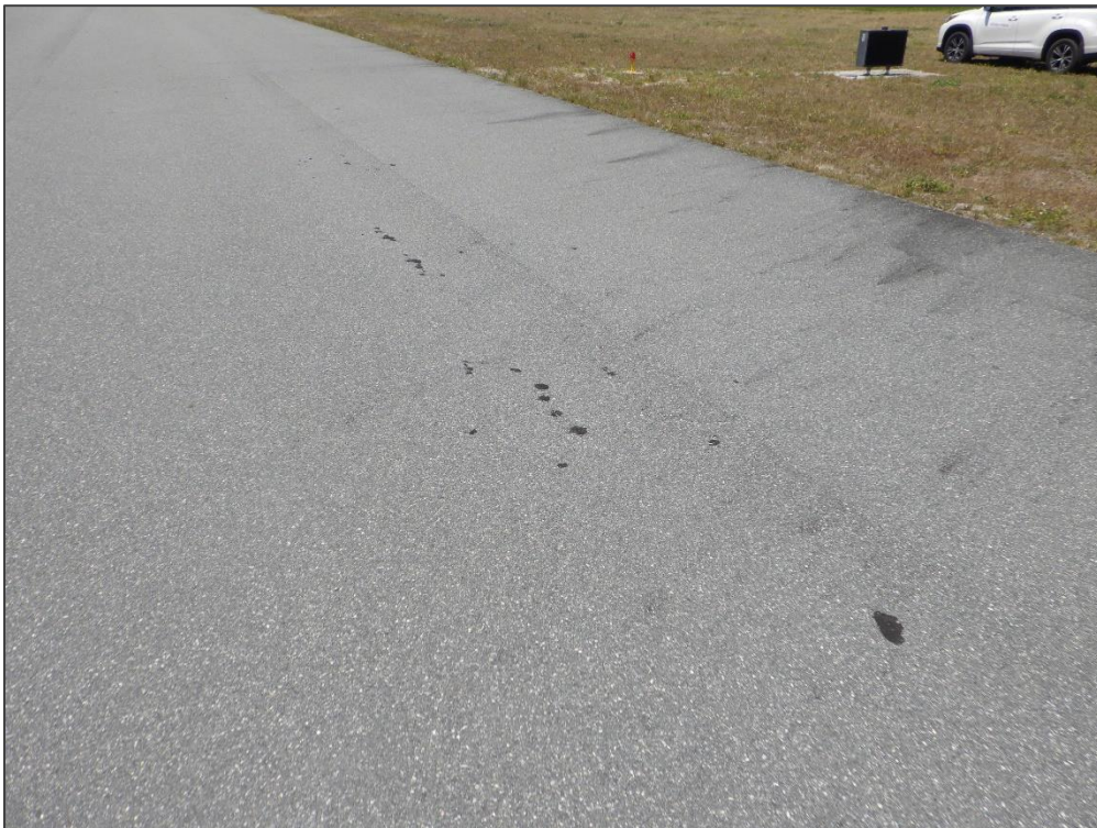
RW 4-22, Section 6210, Sample Unit 500 — Bleeding
