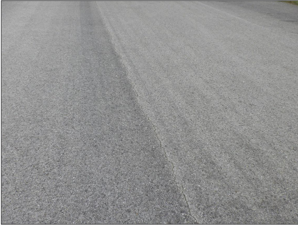
TW G, Section 722, Sample Unit 131 – Longitudinal & Transverse Cracking
