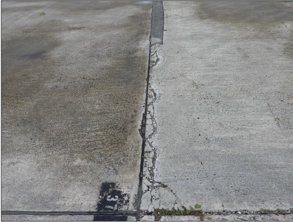
AP CENTER, Section 4110, Sample Unit 309 – Joint Seal Damage, Small Patch, and Joint Spall
