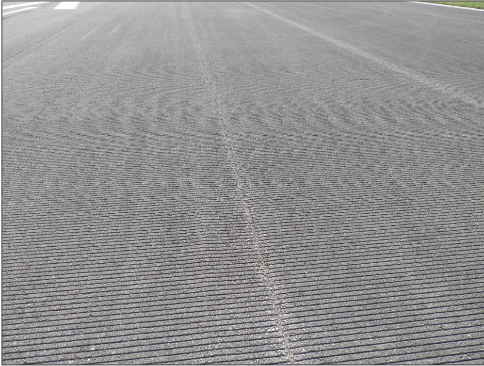
RW 12-30, Section 6205, Sample Unit 308 – Longitudinal & Transverse Cracking
