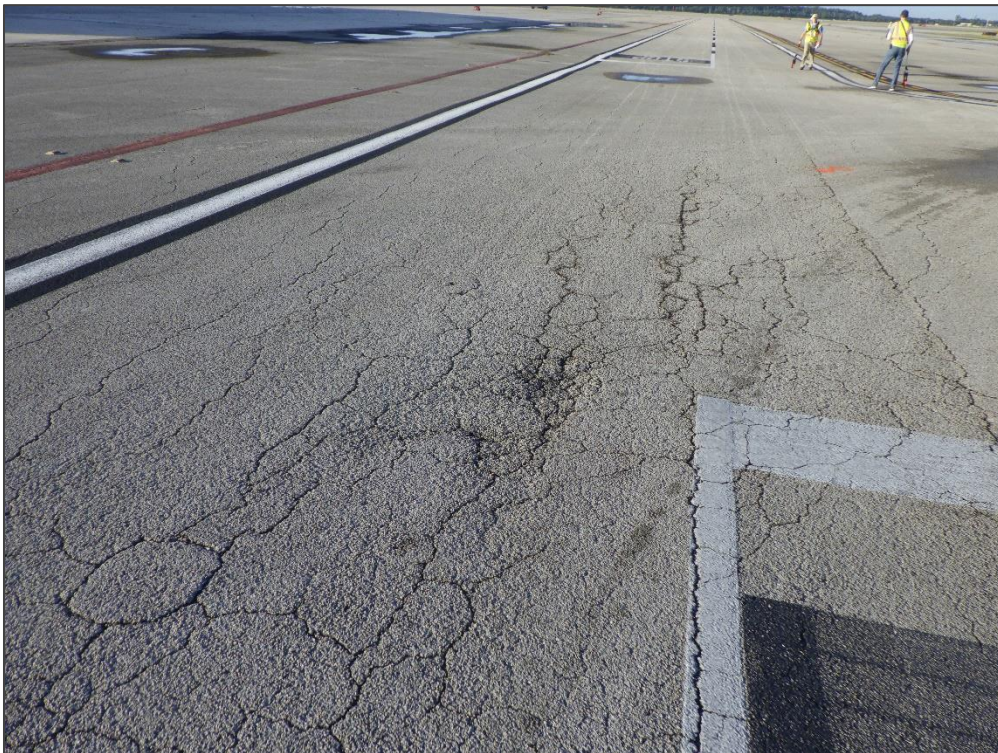
AP CENTER, Section 4105, Sample Unit 164 – Alligator Cracking
