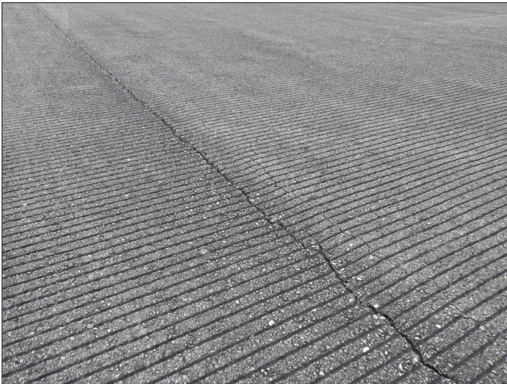
RW 12-30, Section 6205, Sample Unit 393 – Longitudinal & Transverse Cracking and Swelling
