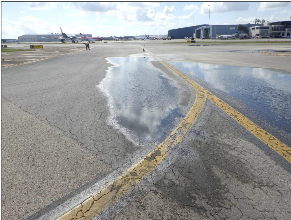
TW N6, Section 1440, Sample Unit 102 – Alligator Cracking and Rutting
