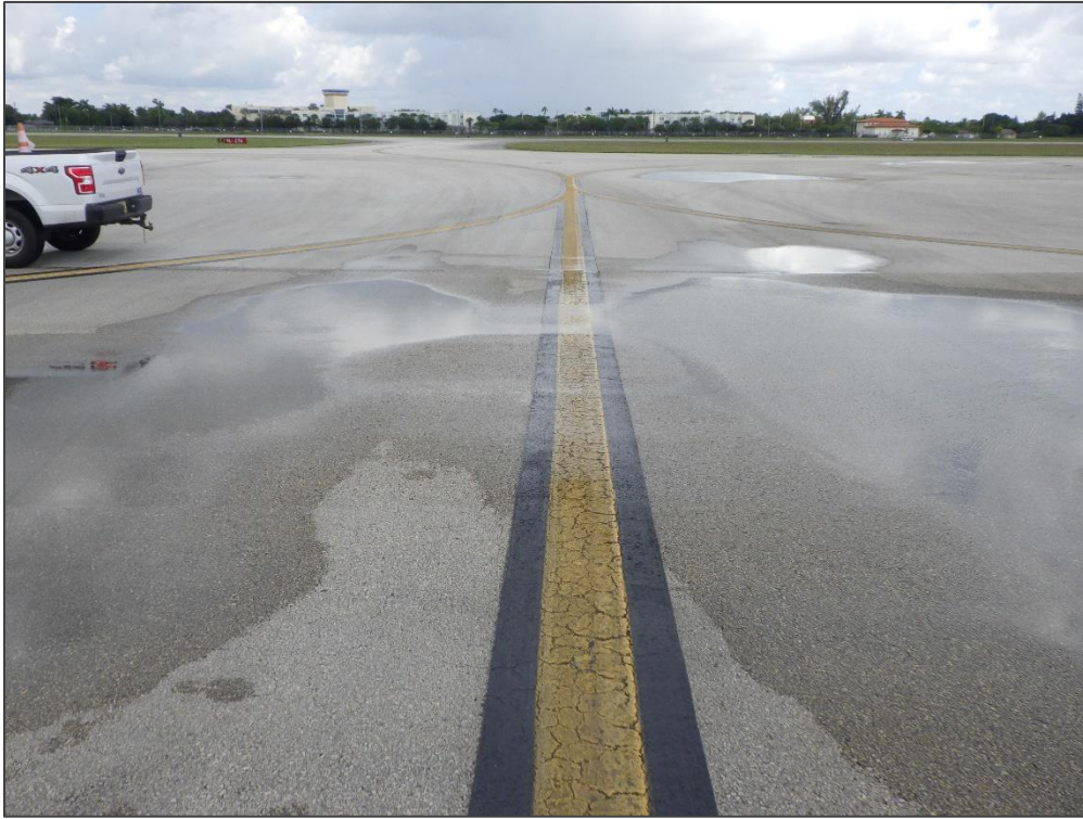
TW P, Section 1640, Sample Unit 327 – Rutting
