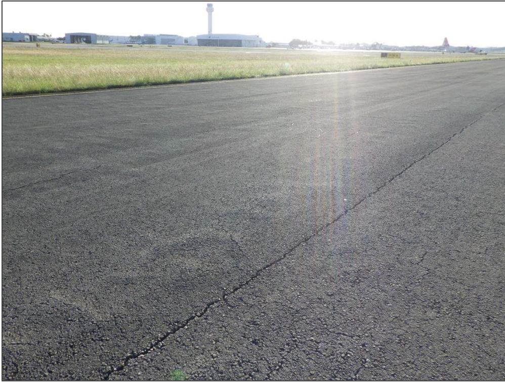
TW T, Section 2005, Sample Unit 144 – Longitudinal & Transverse Cracking and Swelling
