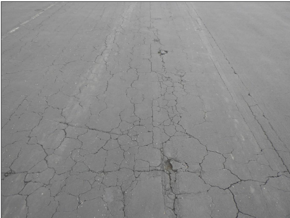
AP SE, Section 4507, Sample Unit 259 – Alligator Cracking
