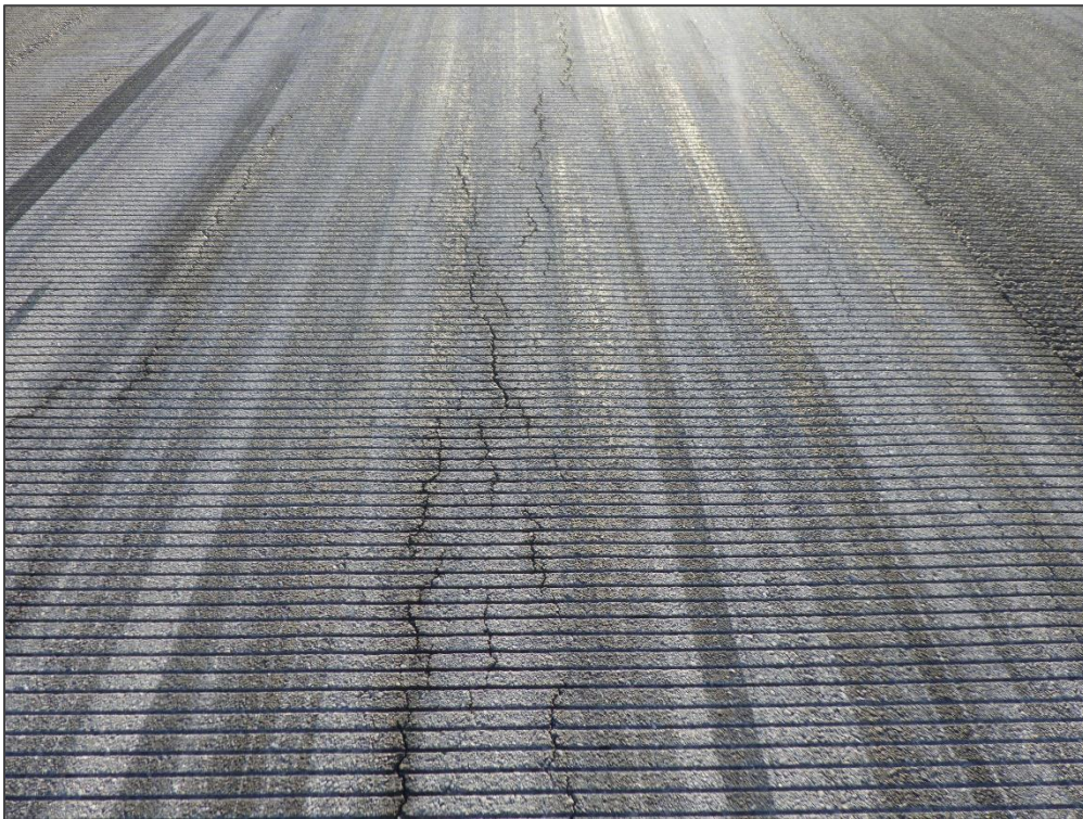
RW 9L-27R, Section 6115, Sample Unit 370 – Alligator Cracking
