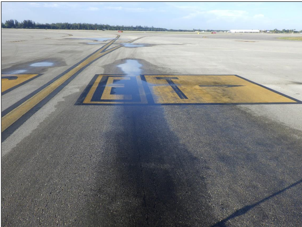
TW E, Section 515, Sample Unit 556 – Rutting
