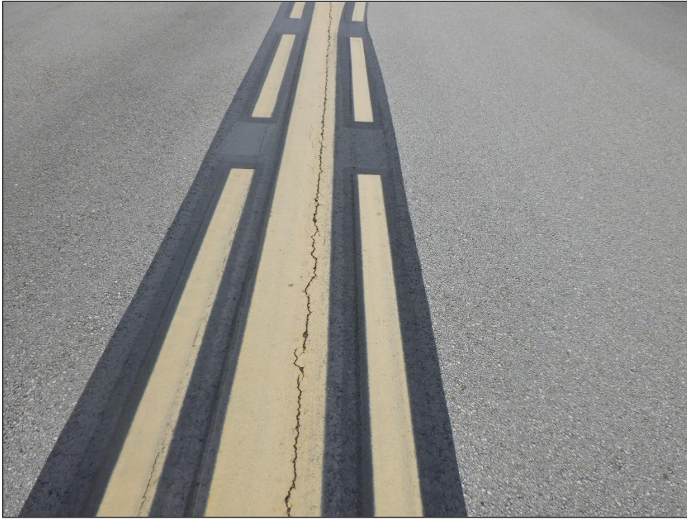
TW A, Section 125, Sample Unit 394 – Longitudinal & Transverse Cracking
