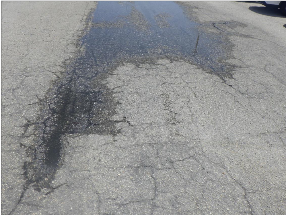
AP SW GA, Section 4305, Sample Unit 370 – Alligator Cracking
