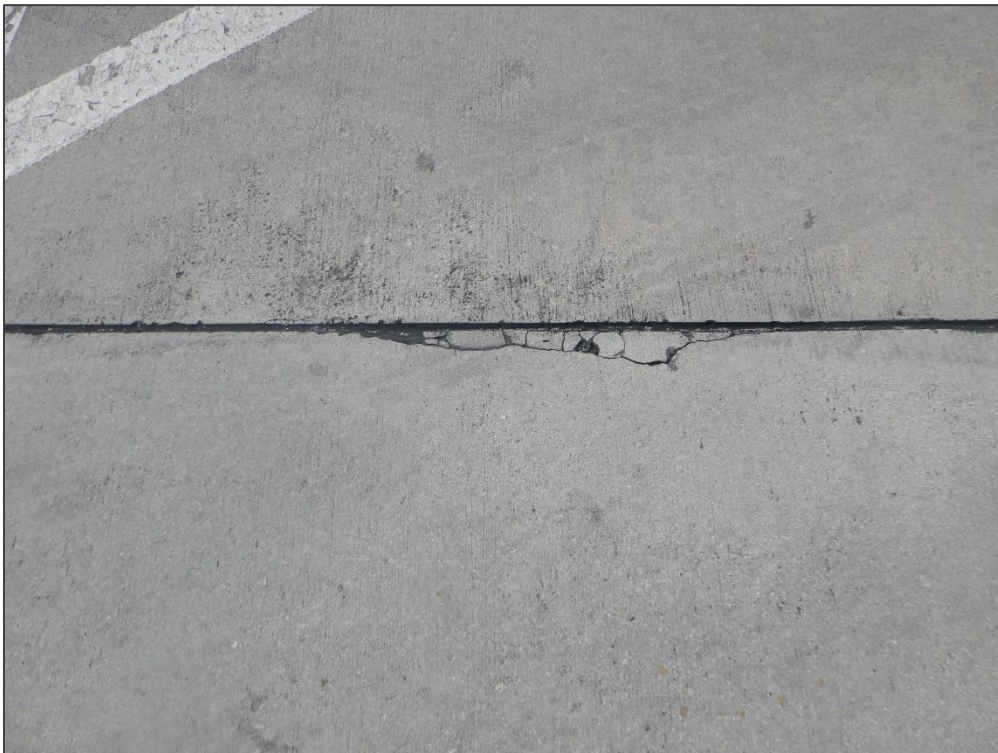
AP N TERM, Section 4115, Sample Unit 152 – Joint Spall
