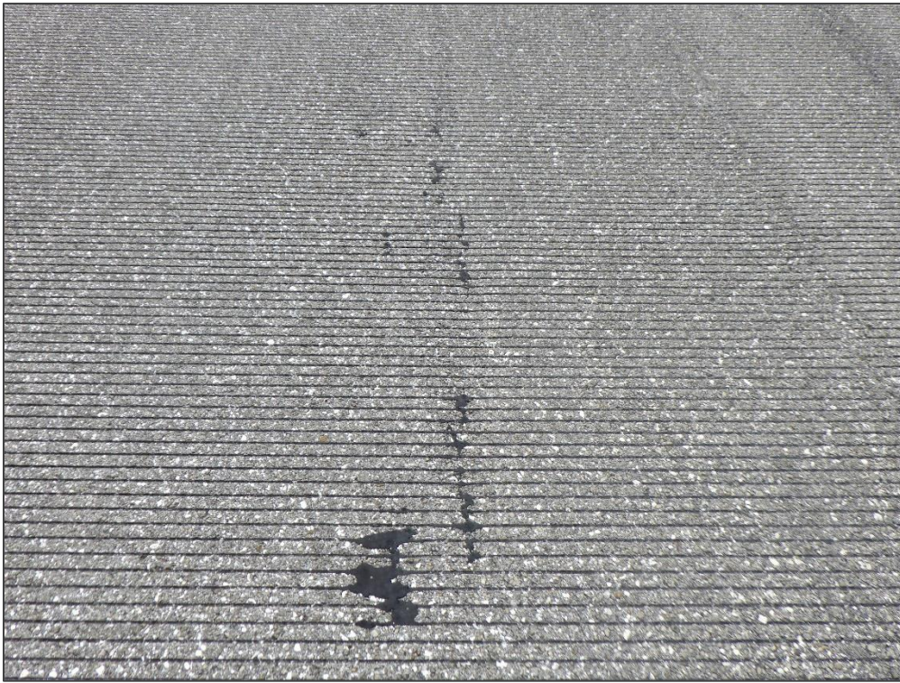
RW 14-32, Section 6305, Sample Unit 149 – Bleeding and Longitudinal & Transverse Cracking
