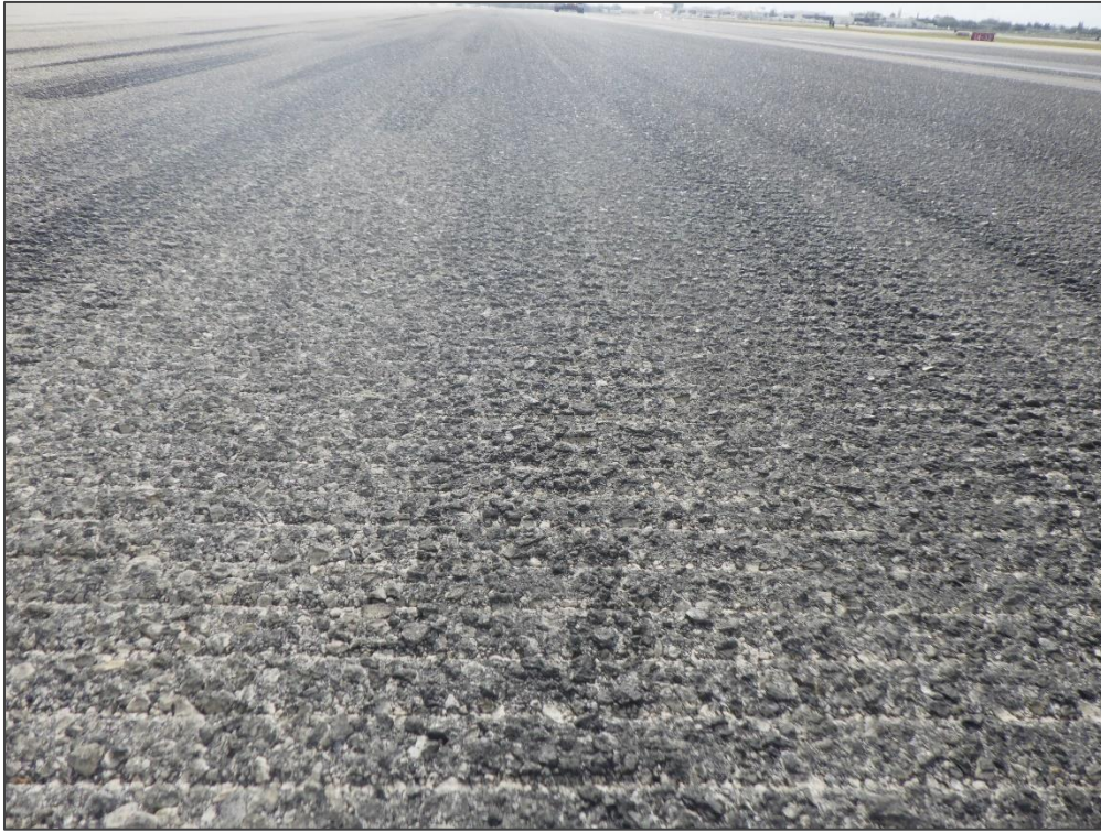
RW 10L-28R, Section 6105, Sample Unit 357 – Raveling
