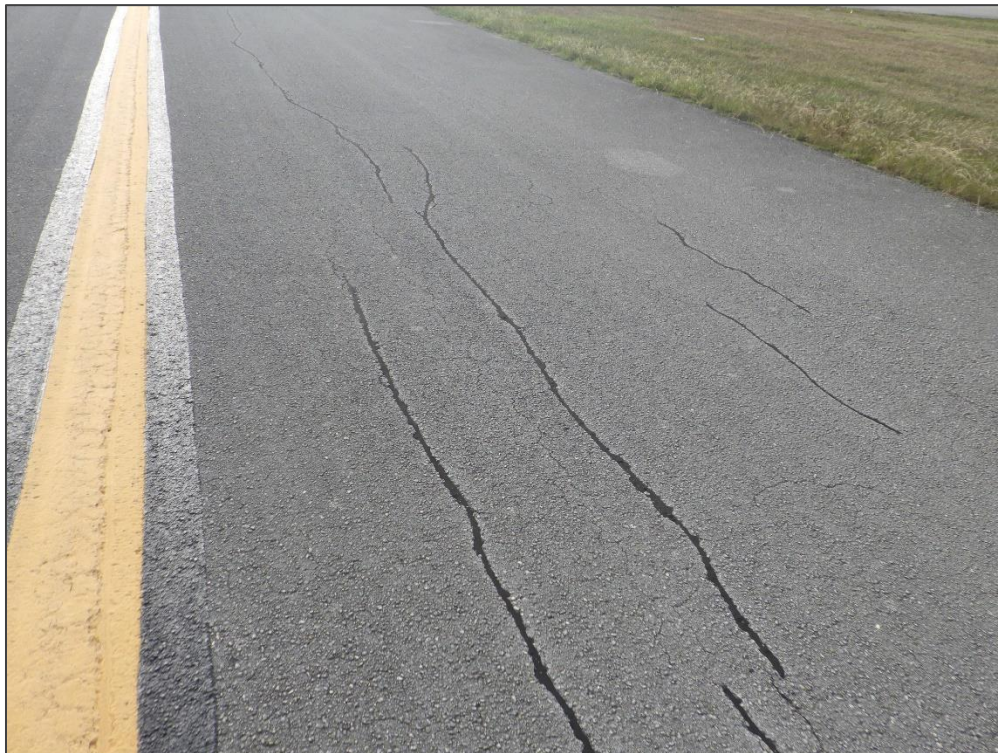
TW R, Section 1805, Sample Unit 215 – Longitudinal & Transverse Cracking
