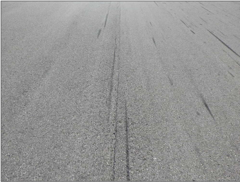
RW 10R-28L, Section 6210, Sample Unit 108 – Longitudinal & Transverse Cracking
