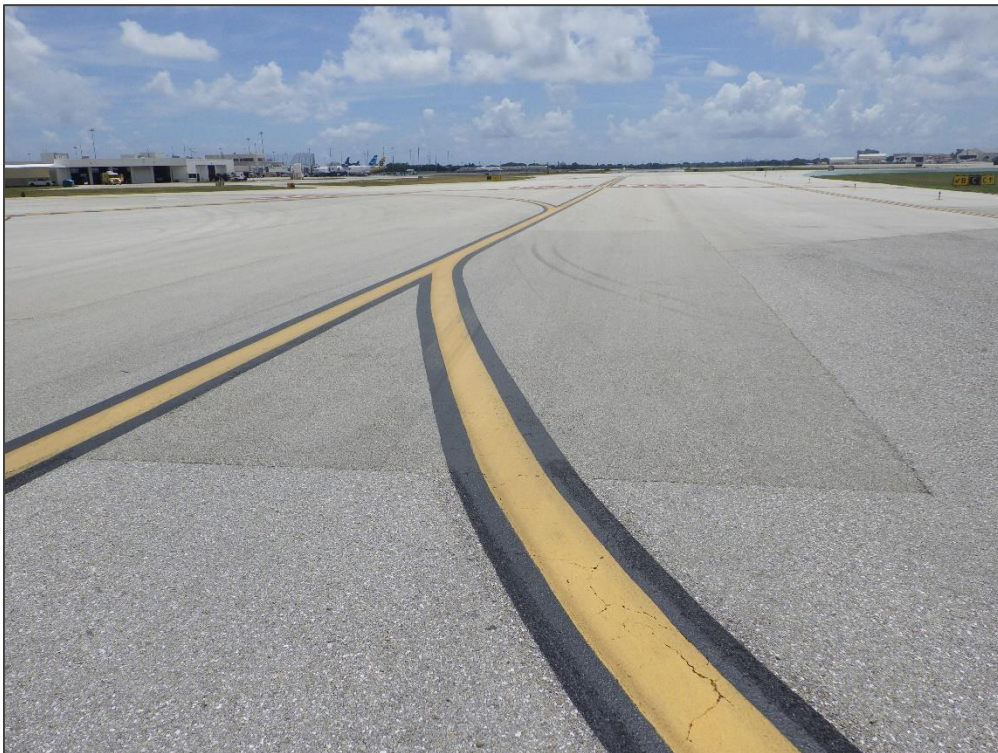
TW C, Section 314, Sample Unit 172 – Patching
