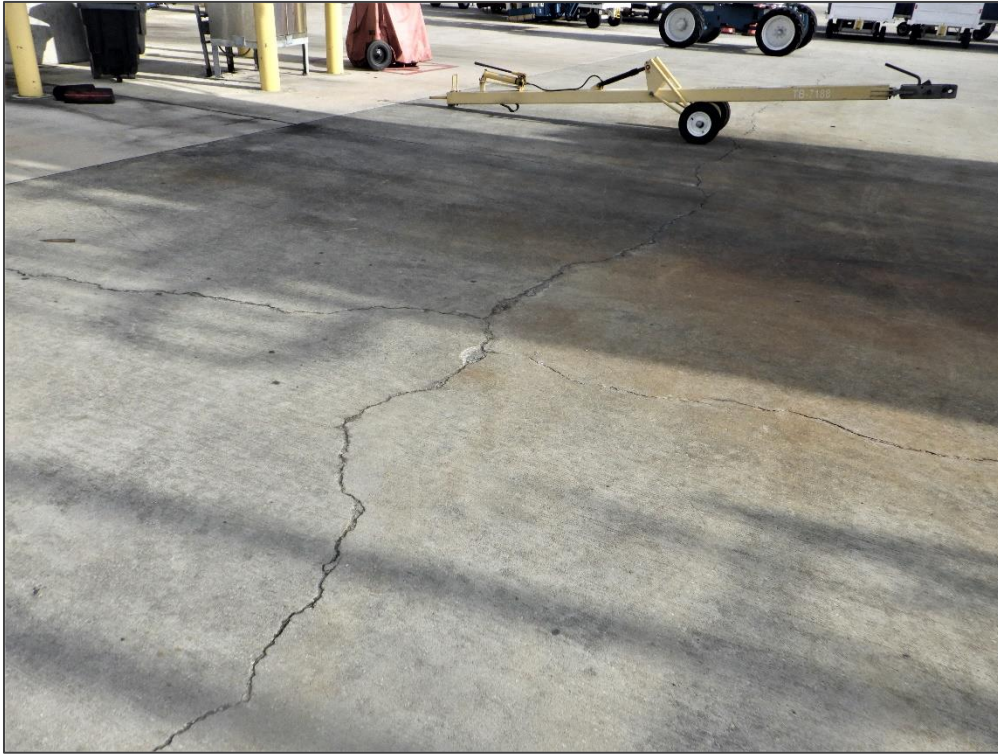
AP N TERM, Section 4140, Sample Unit 401 – Shattered Slab
