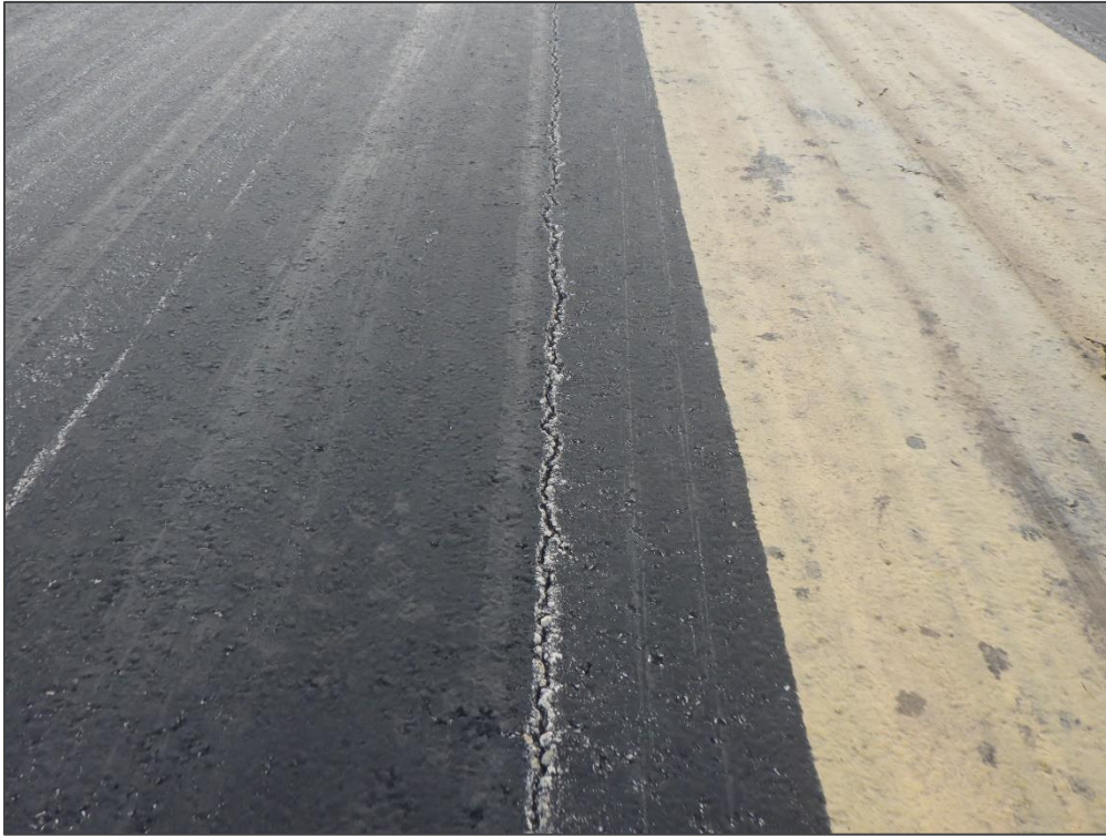
TW L, Section 1005, Sample Unit 402 – Longitudinal & Transverse Cracking
