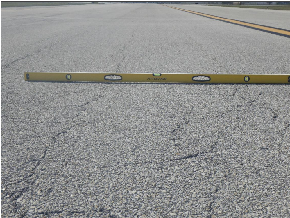
TW B, Section 220, Sample Unit 155 – Rutting
