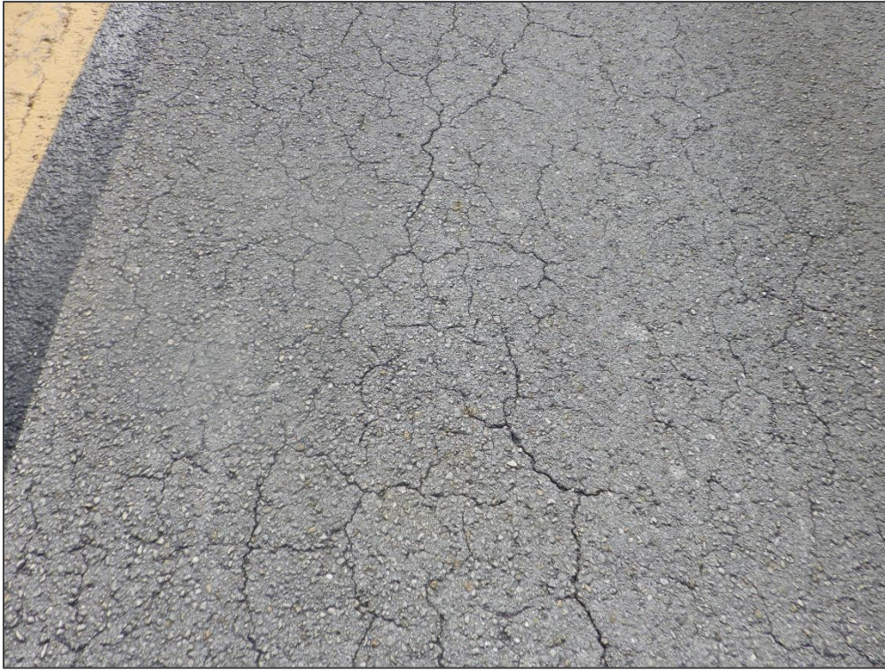
TW R, Section 1805, Sample Unit 225 – Alligator Cracking
