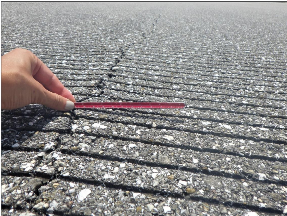
RW 14-32, Section 6305, Sample Unit 186 – Longitudinal & Transverse Cracking and Swelling
