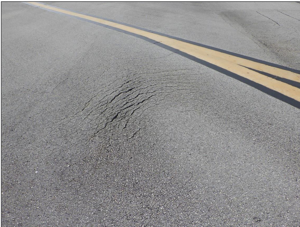
TW F, Section 605, Sample Unit 110 – Slippage Cracking
