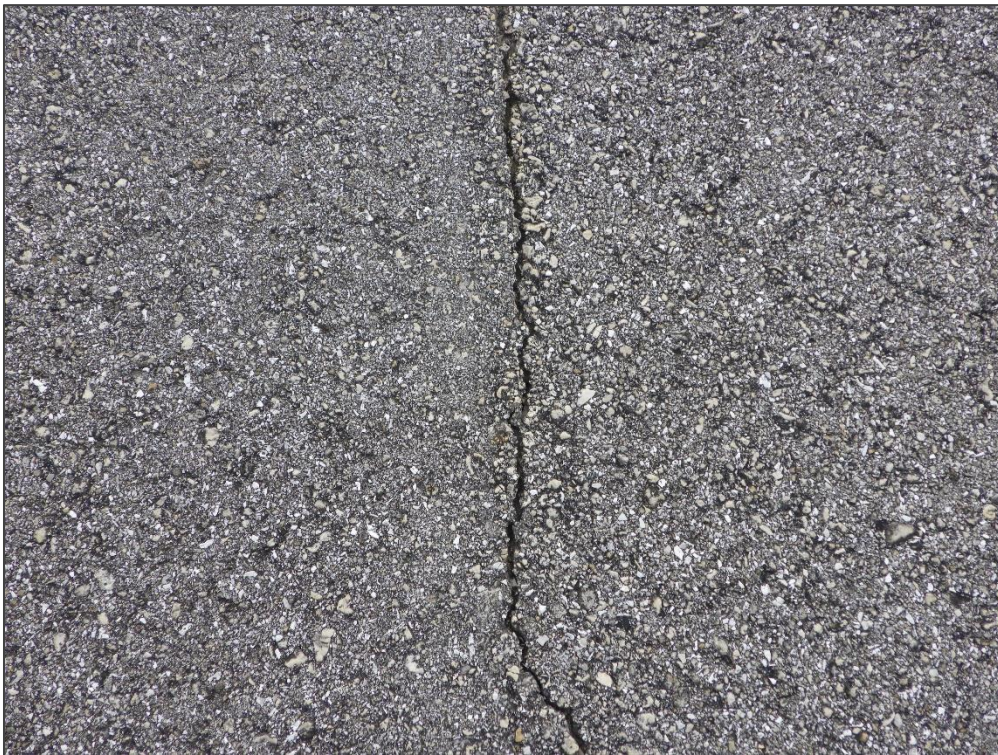
RW 10R-28L, Section 6210, Sample Unit 137 – Longitudinal & Transverse Cracking
