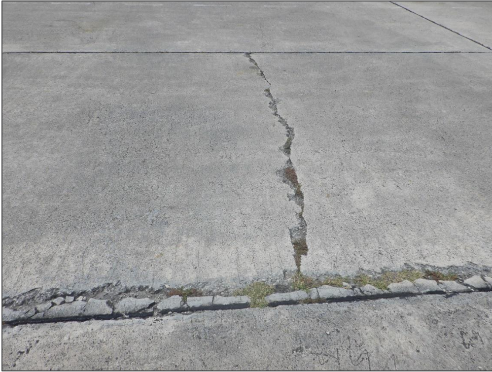
AP SE GA, Section 4515, Sample Unit 401 - Linear Cracking and Joint Spall
