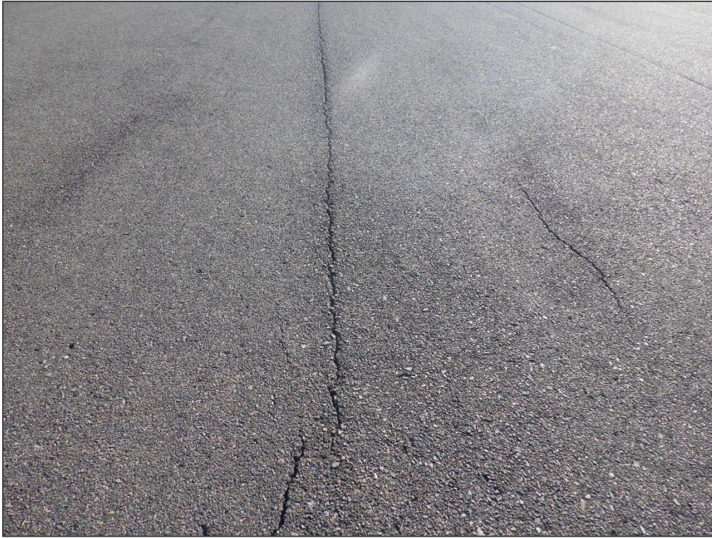
RW 9C-27C, Section 6305, Sample Unit 107 – Longitudinal & Transverse Cracking
