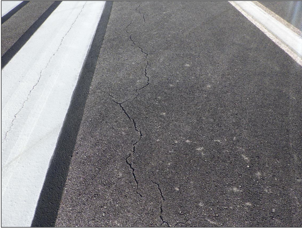
RW 9R-27L, Section 6405, Sample Unit 172 – Longitudinal & Transverse Cracking
