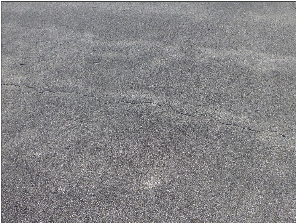
RW 9R-27L, Section 6405, Sample Unit 114 – Longitudinal & Transverse Cracking and Swelling
