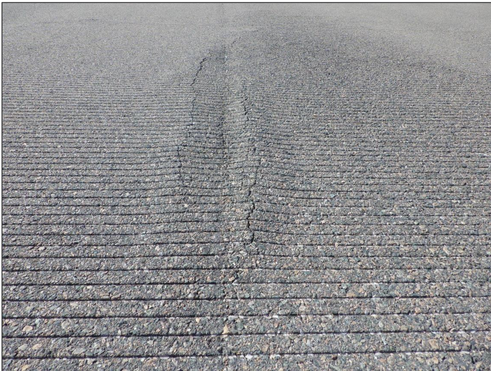
RW 9L-27R, Section 6105, Sample Unit 417 – Longitudinal & Transverse Cracking and Swelling
