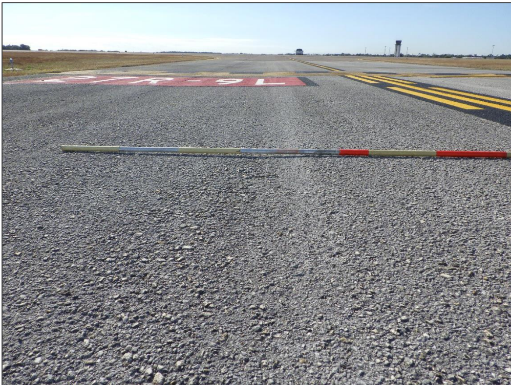
TW R, Section 1820, Sample Unit 184 – Rutting
