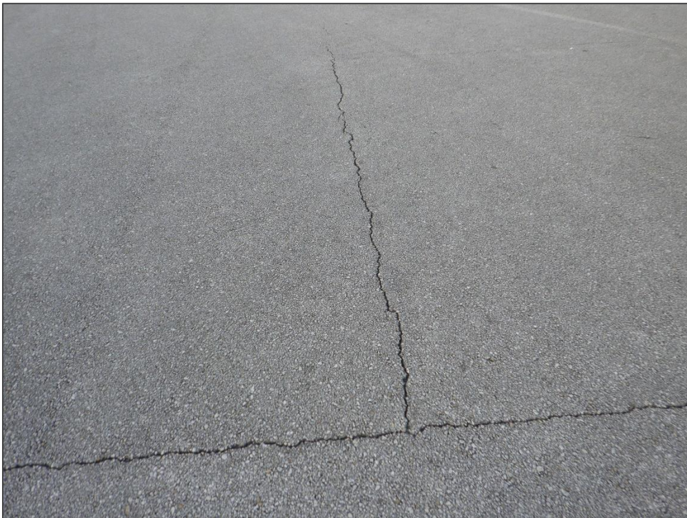
AP TERM, Section 4140, Sample Unit 360 – Joint Reflection Cracking
