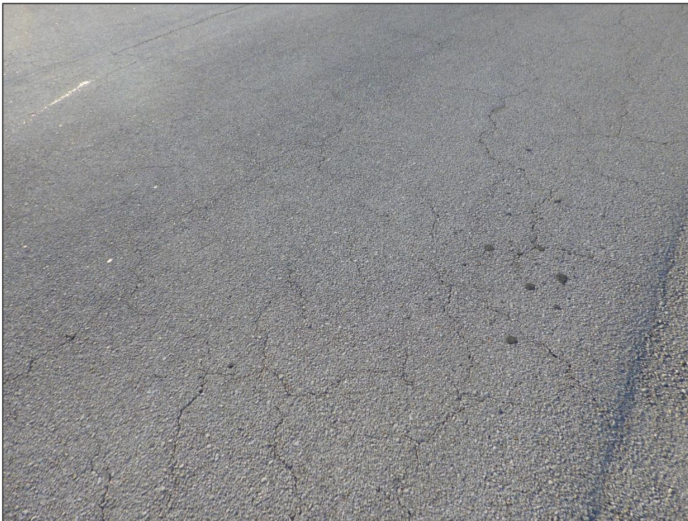
TW L, Section 1208, Sample Unit 131 – Alligator Cracking
