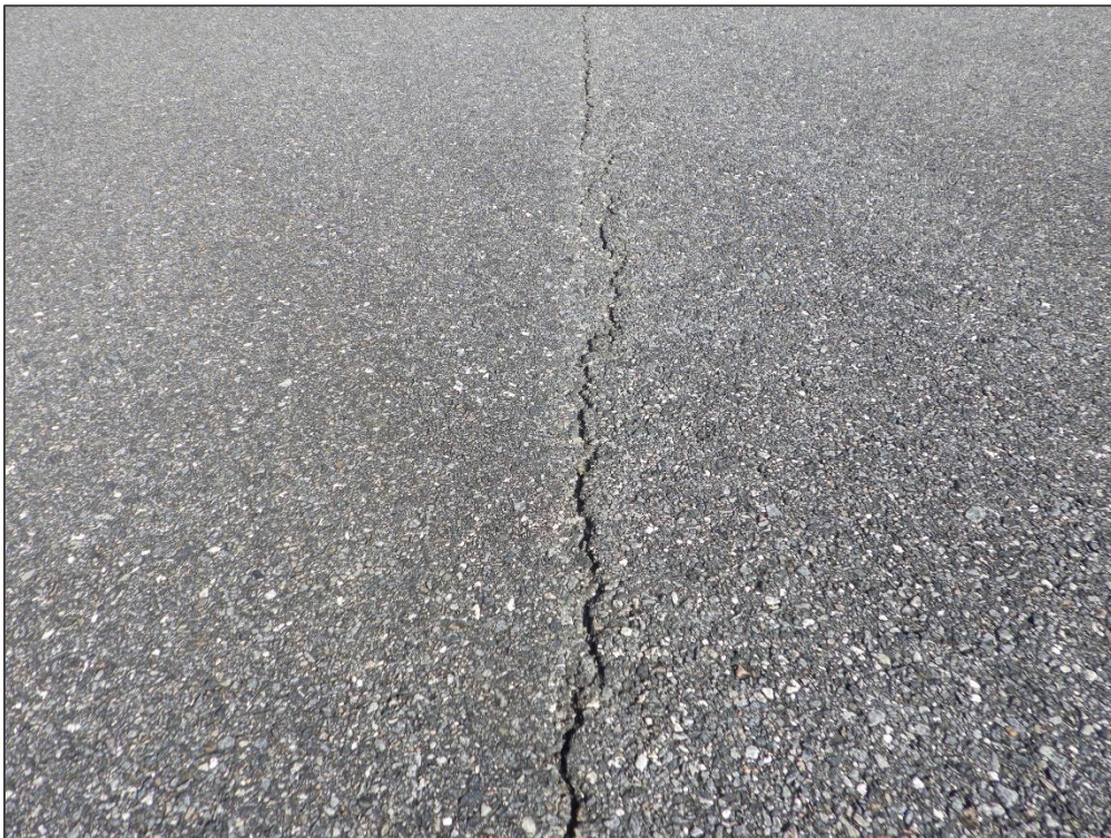
TW B, Section 615, Sample Unit 240 – Longitudinal & Transverse Cracking
