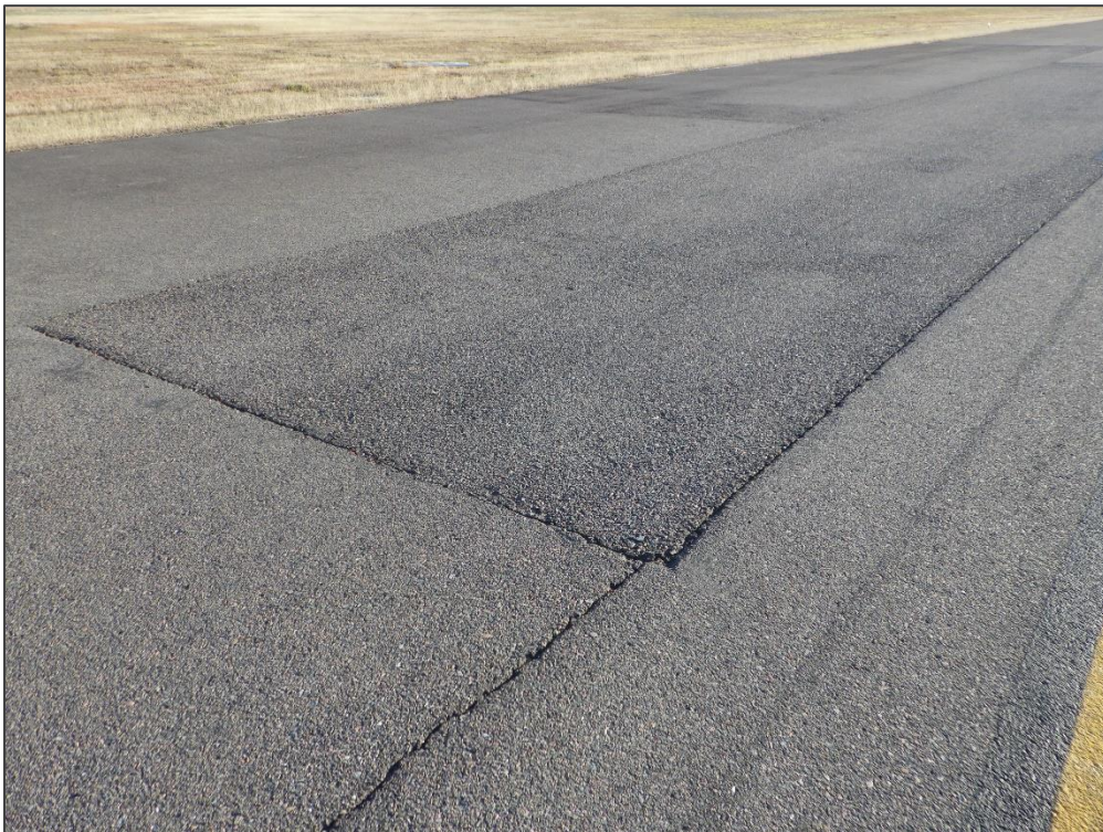
RW 9C-27C, Section 6305, Sample Unit 151 – Patching
