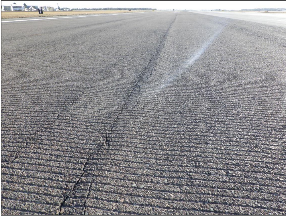
RW 9L-27R, Section 6105, Sample Unit 252 – Longitudinal & Transverse Cracking and Swelling
