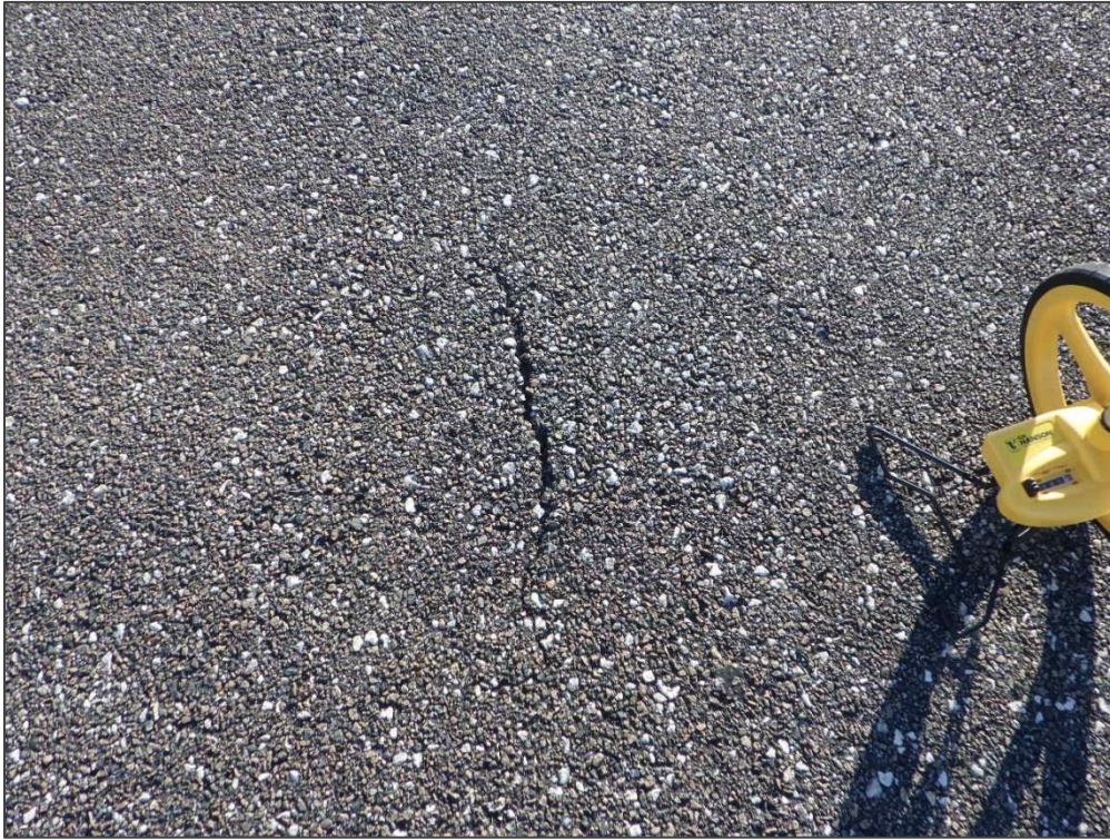
TW S, Section 1925, Sample Unit 201 – Longitudinal & Transverse Cracking
