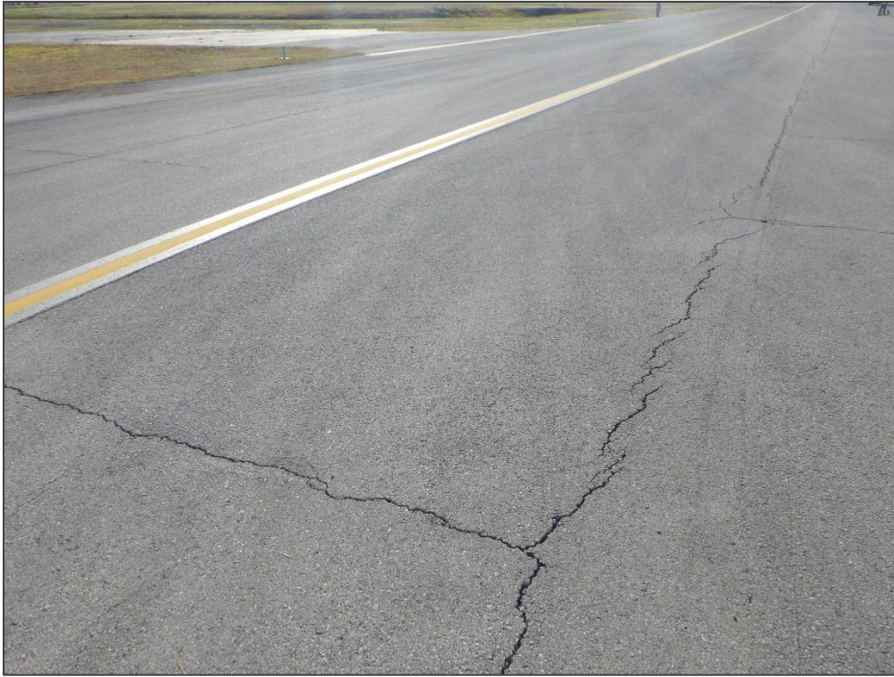
TW C, Section 355, Sample Unit 124 - Joint Reflection Cracking
