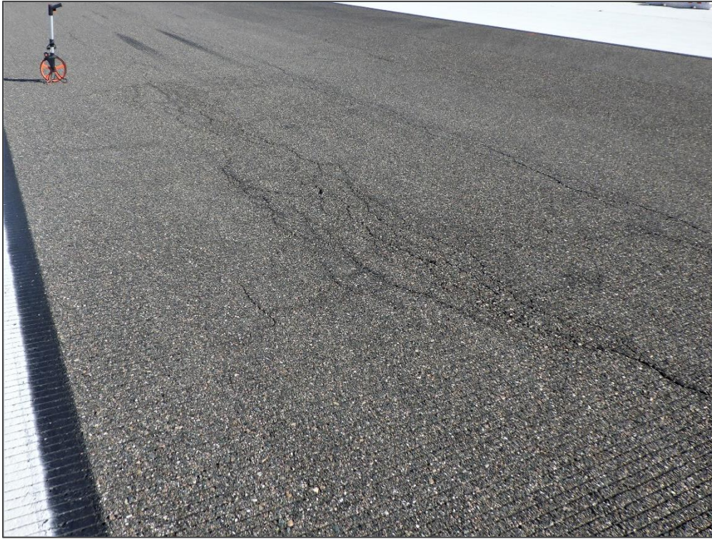
RW 18-36, Section 6290, Sample Unit 397 – Alligator Cracking
