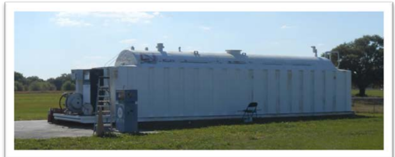
Above Ground Fuel Tank
